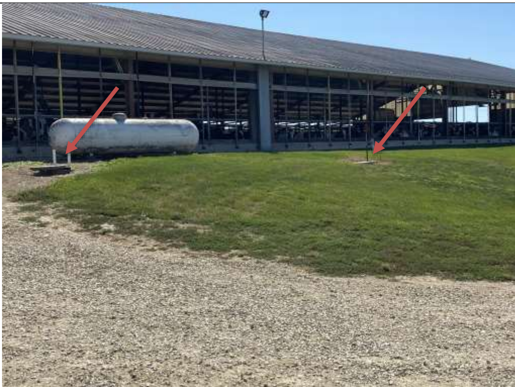
Photo #: IMG_3659 Date/Time: 9/4/2024 10:44 AM Photo taken by: J. Borgrud Photo Location Williams Bedrock Bovines – Main Farm Description: Looking east at the reception tanks south and west of the freestall barns that go to the sand separation system.
