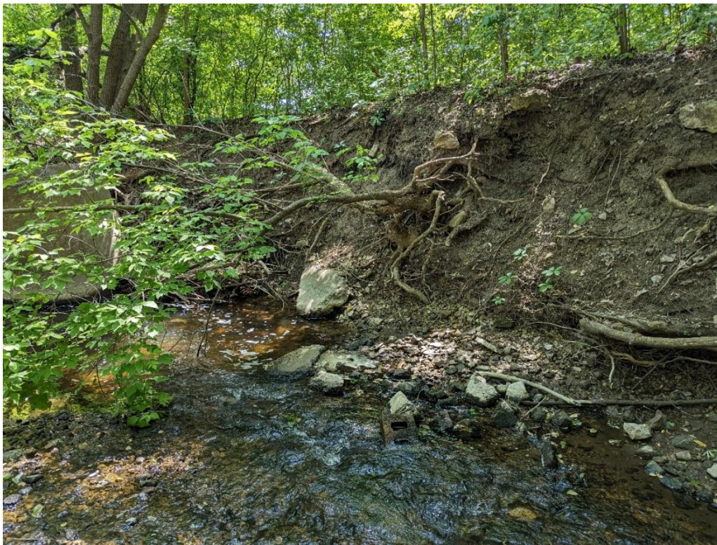
Image 2.1 – Bank, undercut with exposed roots..
