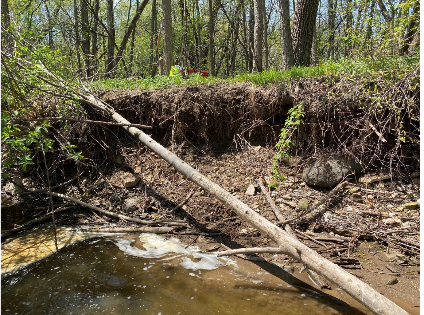
Image 1.3 – Bank, undercut, with fallen trees.
