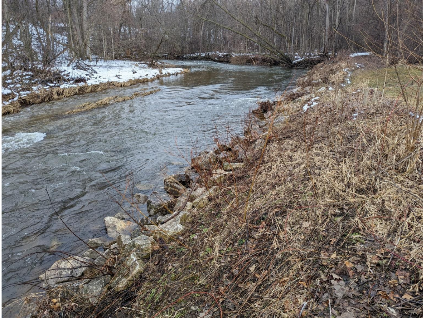
Image 1.1 – Looking southwest. Bank on top right, undercut with slumped sections in stream. Existing downstream riprap on lower right.
