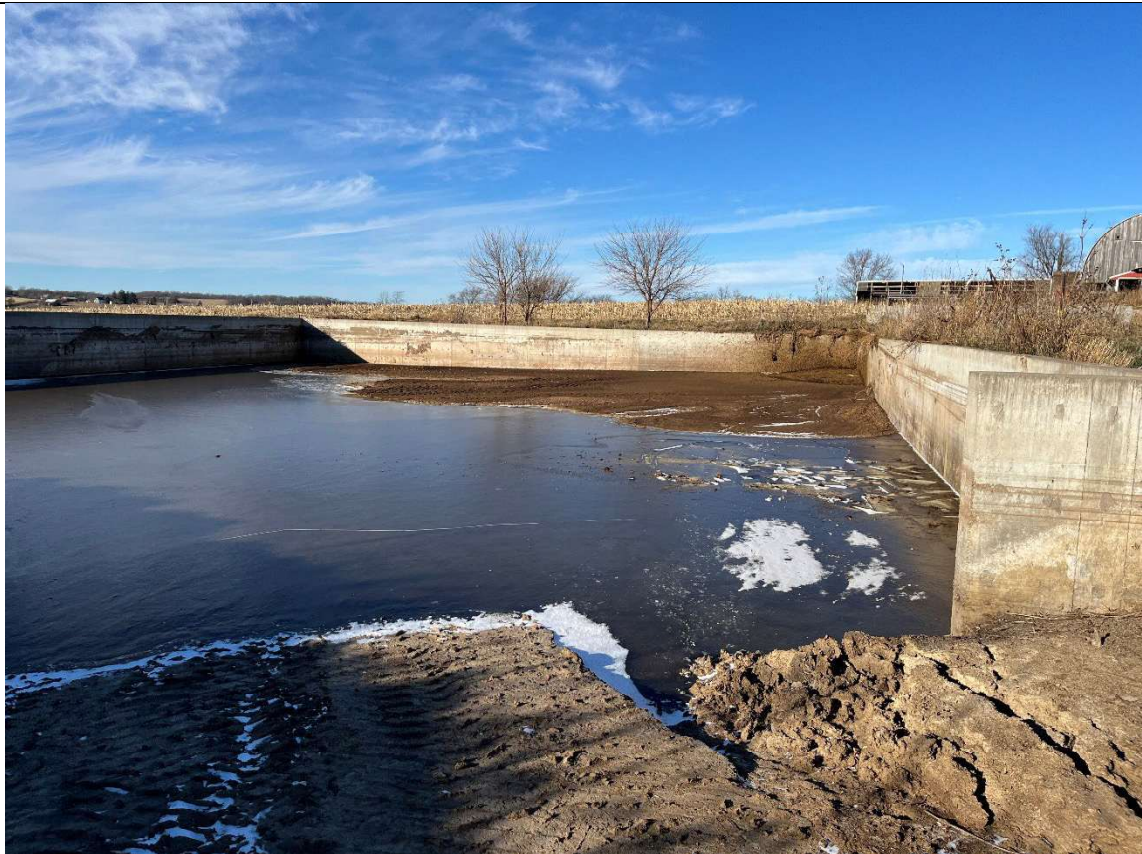
Photo taken by: E. Struck Photo date: 12/05/2024 Description: Photo 21. Marks Avenue WSF. Manure transferred with pushout in NE corner. Note erosion on the right side of the ramp in the foreground. Photo facing N.
