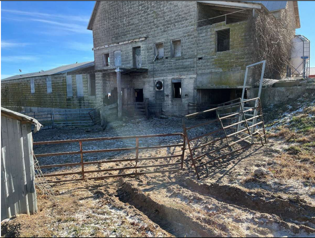
Photo taken by: S. Wettach Photo date: 12/05/2024 Description: Photo 5. Outdoor lot without runoff controls. Photo facing SE.
