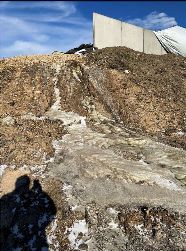
Photo taken by: E. Struck Photo date: 12/05/2024 Description: Photo 30. FSA leachate flow path and erosion from bunkers E. Photo facing NE.
