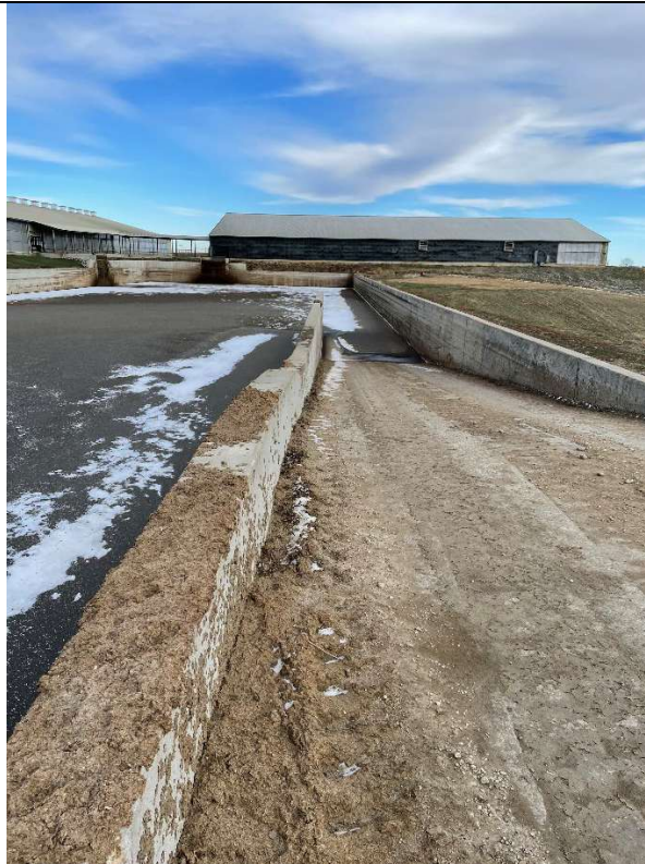
Photo taken by: E. Struck Photo date: 12/05/2024 Description: Photo 17. WSF2 western end access ramp. Photo facing E.
