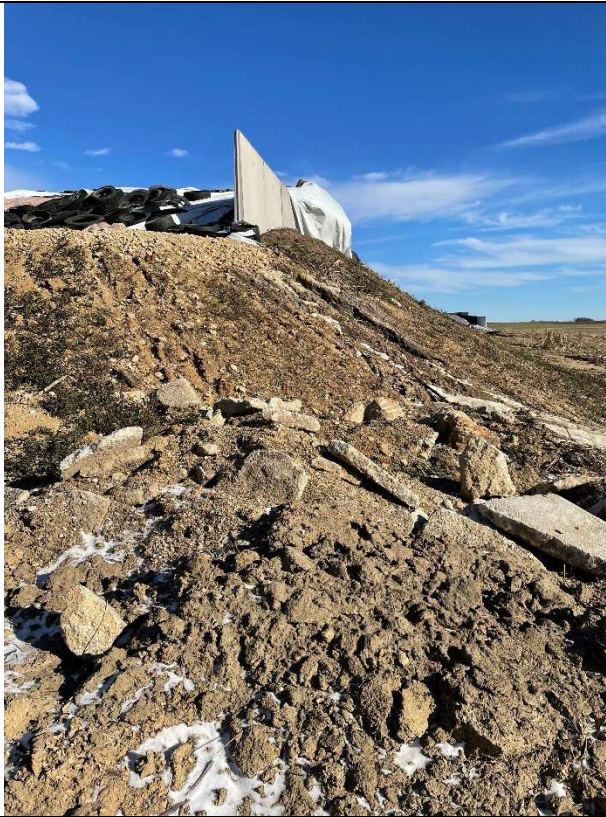
Photo taken by: E. Struck Photo date: 12/05/2024 Description: Photo 29. FSA leachate flow path and erosion between bunkers E and G. Photo facing E.
