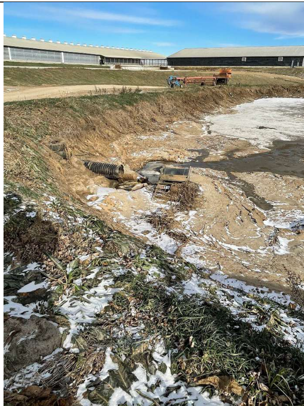
Photo taken by: E. Struck Photo date: 12/05/2024 Description: Photo 15. WSF1 northern end. Note frozen solids below transfer line and condition of earthen sidewalls. Photo facing E.
