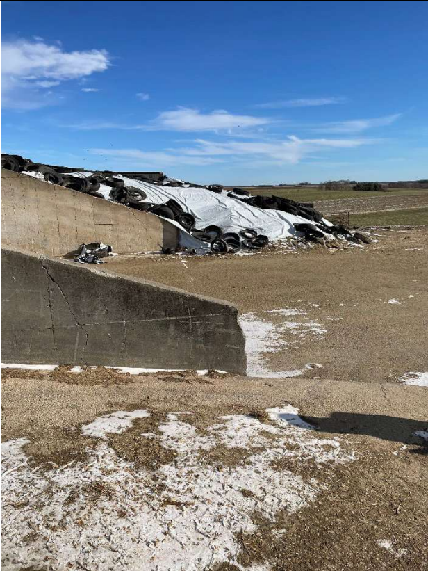
Photo taken by: E. Struck Photo date: 12/05/2024 Description: Photo 32. FSA bunkers C&D. Photo facing E.
