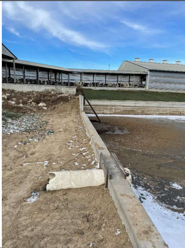
Photo taken by: S. Wettach Photo date: 12/05/2024 Description: Photo 18. WSF2 western sidewall with pushout from free stall barn. Photo facing N.
