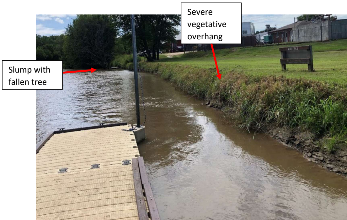
Image 2 – Severe vegetative overhang and slump with fallen tree
