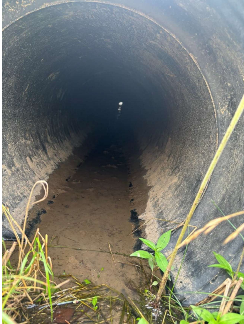
Image 2.5 – Outfall piping of Pond #2
