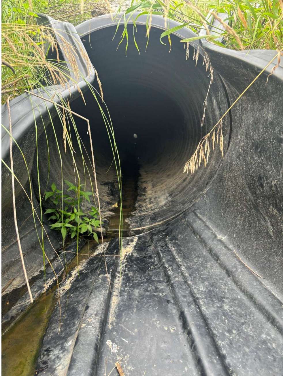
Image 1.1 – Outfall piping of Pond #1.
