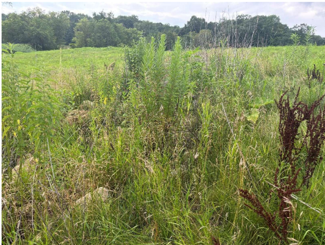
Image 1.2 – Vegetative growth within the Riprap at the Outfall of Pond #1.
