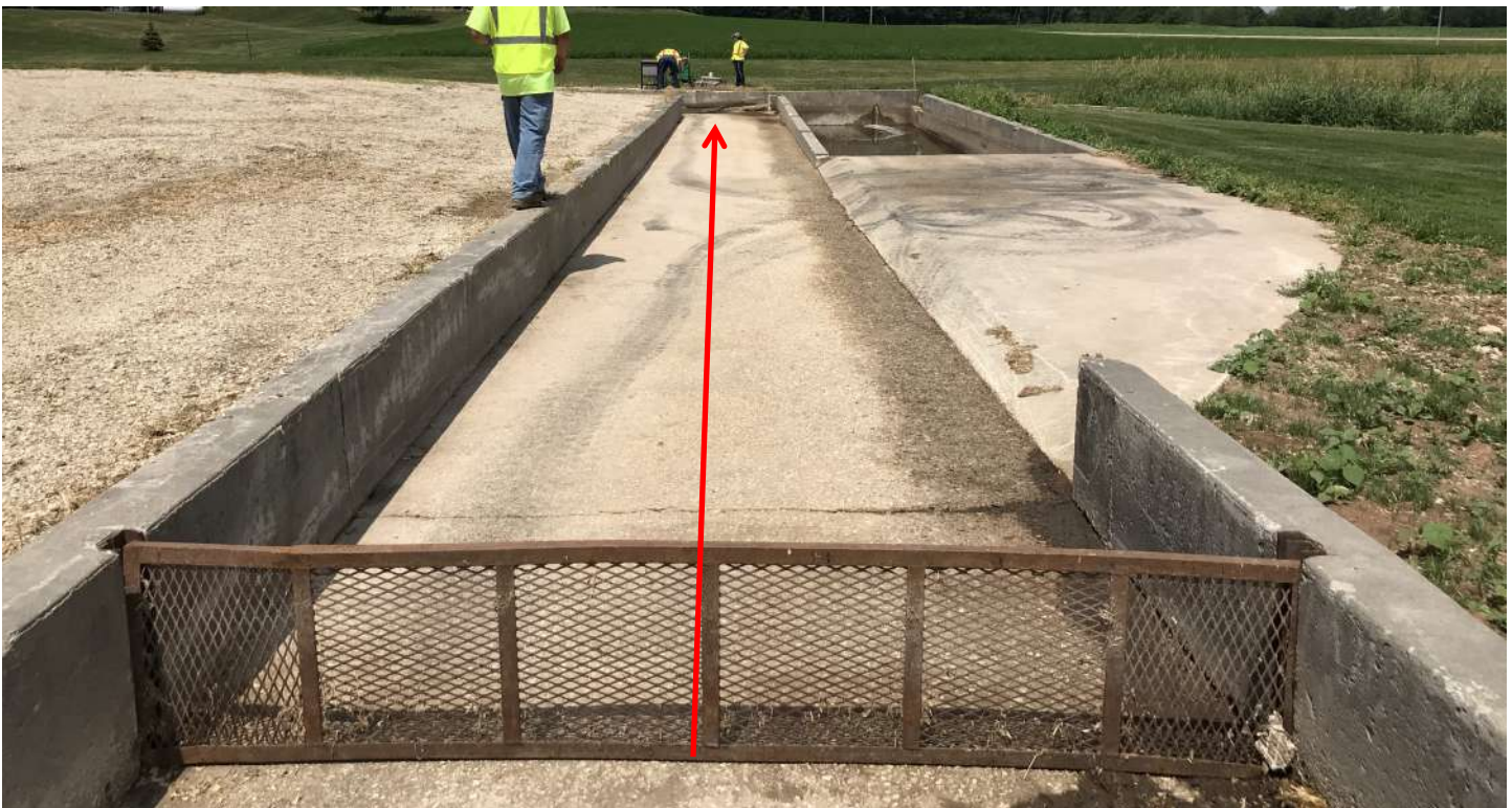
Photo #: 66 Photo Description: The runoff collection system for the east feed storage area. Runoff from the FSA is directed north and into this concrete swale. The red arrow represents the flow path. Date/Time of Photo: 07/07/2020 13:28 Photo Location: Main Site Photo By: James Salscheider
