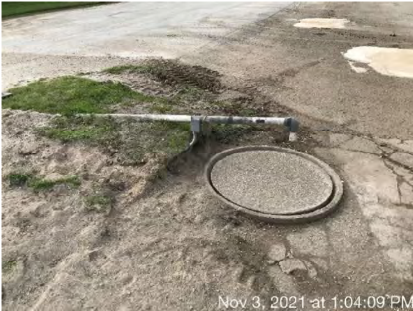
Photo 139. The second collection inlet for the northern feed storage area at Site 1. This photo was taken facing northwest. The inlet was covered to prevent stormwater collection.
