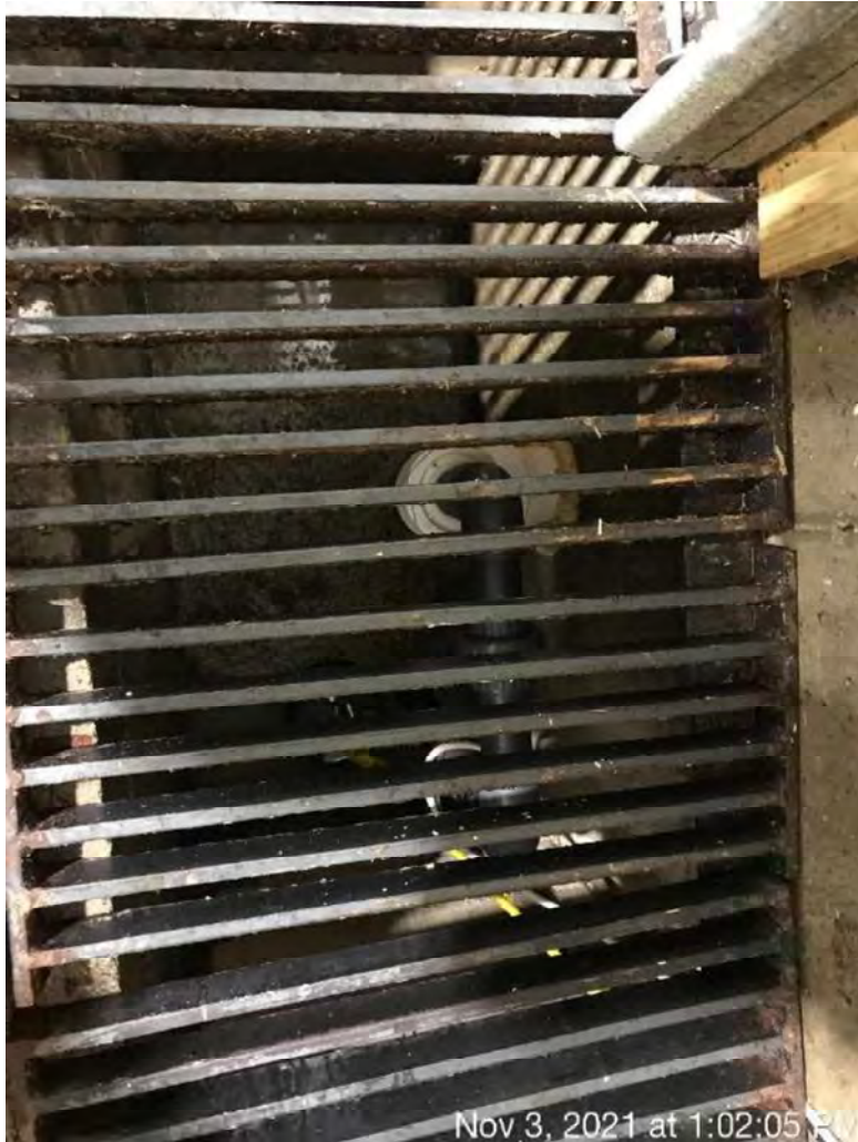
Photo 87. The pump that transfers process wastewater from the machine-washing area to the manure transfer system.
