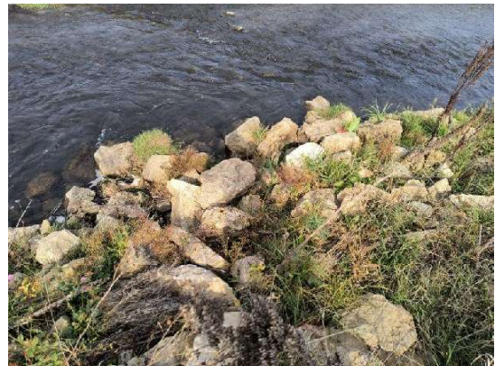
Site 1 – Loose Rock
