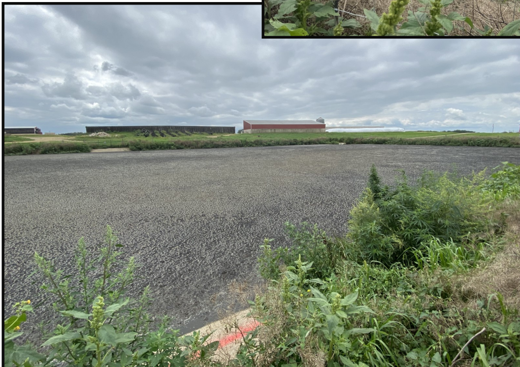
Photo 6 (Bottom Left): Looking south west across WSF 2. The permanent maximum operating level marker can be seen on the northern wall of the waste storage facility. A permanent margin of safety marker was not present in WSF 2.
