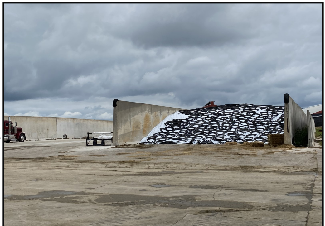
Photo 13 (Right): Looking east toward the eastern portion of the feed storage area from the center of the southern end of the feed storage. The eastern portion of the feed storage primarily slopes west toward the center of the feed storage area where leachate and feed storage runoff is directed to the runoff collection basin (pictured in photo 16).
