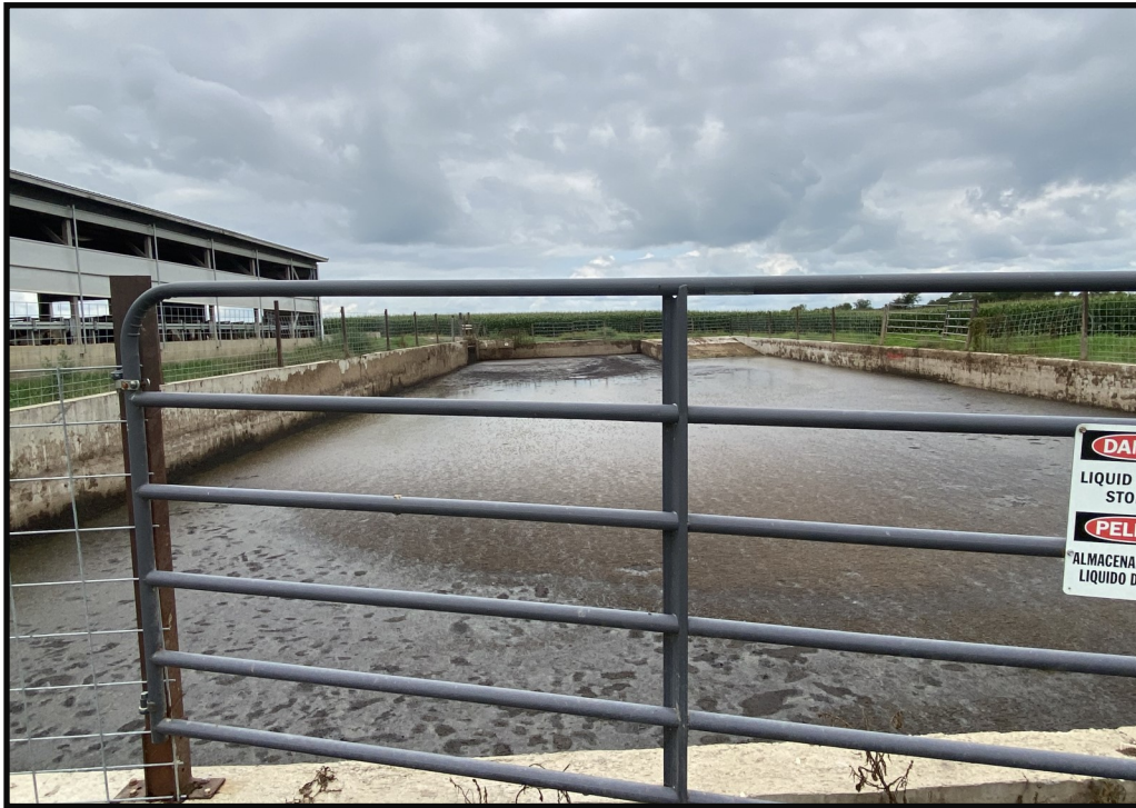
Photo 10 (Left): Looking west across WSF 4. A safety fence was observed around the entire perimeter of the of the waste storage facility and a permanent maximum operating level marker can be seen on the northern wall. A layer of dried manure extending above the maximum operating level can also be seen along the walls of WSF 4.
