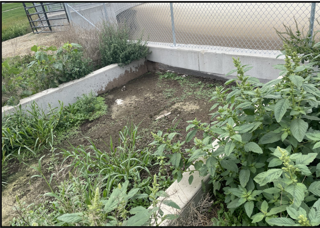
Photo 7 (Top Left): Looking at the overflow channel where manure from WSF 2 flows into WSF 3. Manure solids and vegetation growth can be seen accumulating within the overflow channel.
