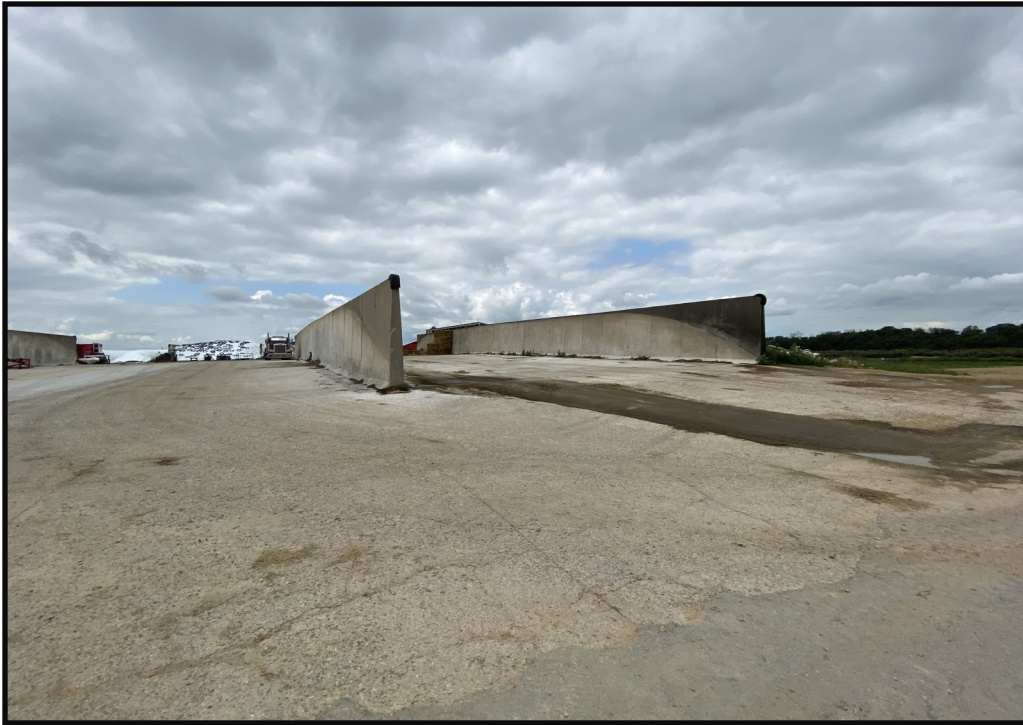
Photo 14 (Top Left): Looking west toward the east end of the feed storage area. Portions of the east end of the feed storage slope east away from the center of the feed storage area where leachate and feed storage runoff is directed to the runoff collection basin. Leachate and feed storage runoff that does not flow west toward the runoff collection basin flows east where it directly enters inlets to the runoff transfer system (pictured in photo 15).
