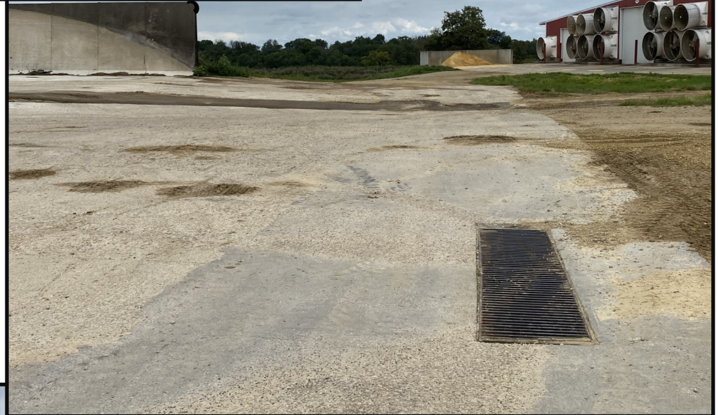
Photo 15 (Right): Looking north along the east end of the feed storage area where inlets to the runoff transfer system are located. Leachate and feed storage runoff that enters the runoff collection basin or directly enters through the inlets to the runoff transfer system are transferred to WSF 3.
