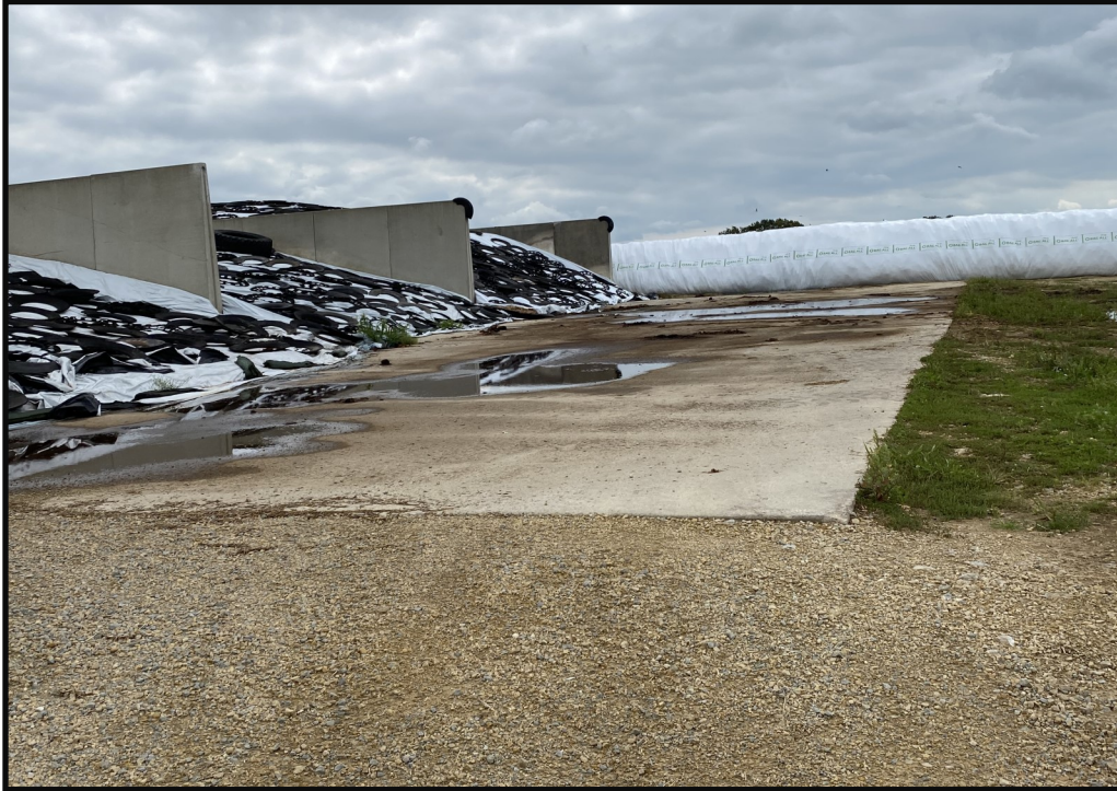
Photo 12 (Left): Looking south along the west end of the feed storage area. The western portion of the feed storage slopes east toward the center of the feed storage area where leachate and feed storage runoff is directed to the runoff collection basin (pictured in photo 16).
