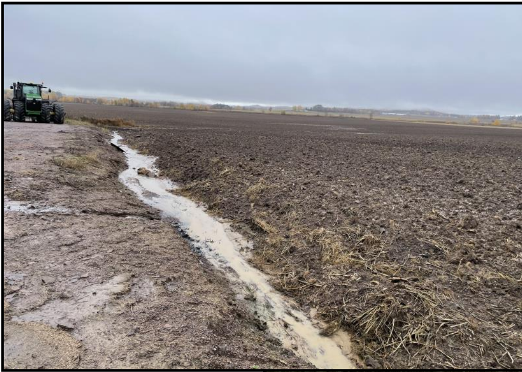
Photo 16 (Top Left): Looking east along the outside south edge of the feed storage area. The feed storage runoff seen discharging around the feed storage in photo 15 can be seen flowing east along this edge toward the area where the runoff collection tank is located (pictured in photo 19).
