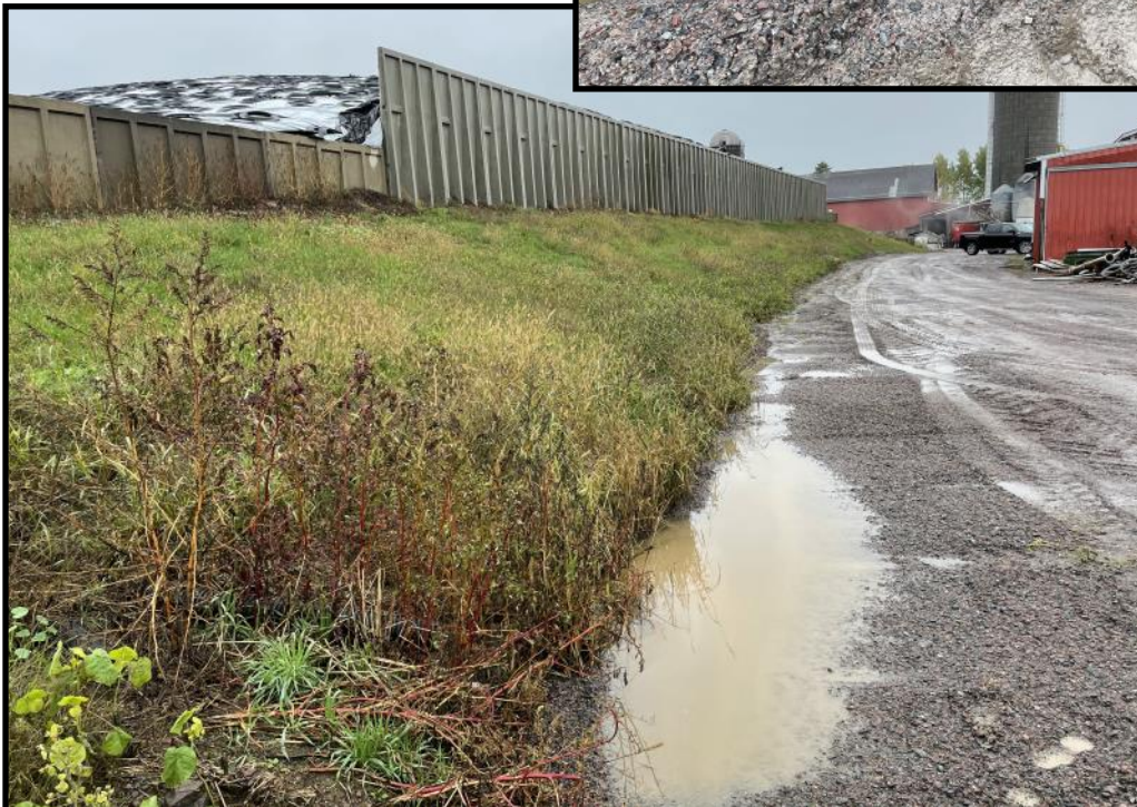
Photo 18 (Bottom Left): Looking north along the eastern edge of the feed storage area from a culvert inlet on the south east corner of the feed storage. The culvert outlets into the field directly south of the feed storage area where the runoff collection tank is located (pictured in photo 19). An outlet to another tile line that runs underneath the feed storage can be seen in this area, which discharges into the culvert.
