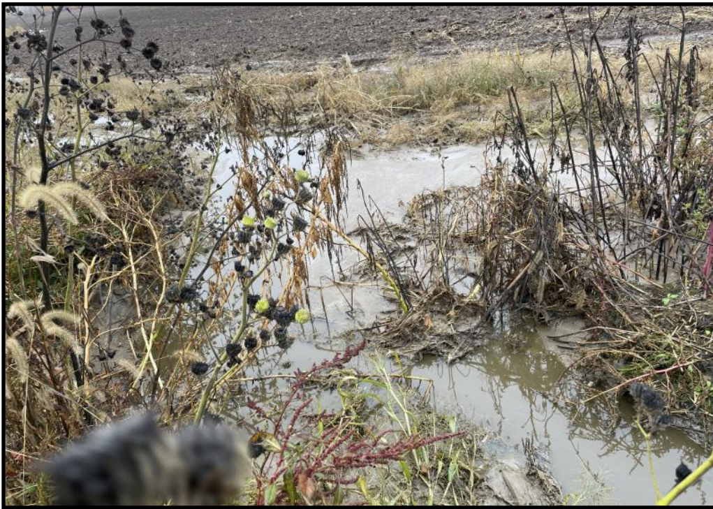
Photo 21 (Left): Looking at material pooling in the field east of the main farm just east of the culvert pictured in photo 20, near the solid manure stacking area adjacent to the abandoned calf hutch area. A significant amount of runoff discharging from the culvert pictured in photo 20 and from the solid manure storage area can be seen pooling in this area. The observed material was very cloudy and greenish brown in color.
