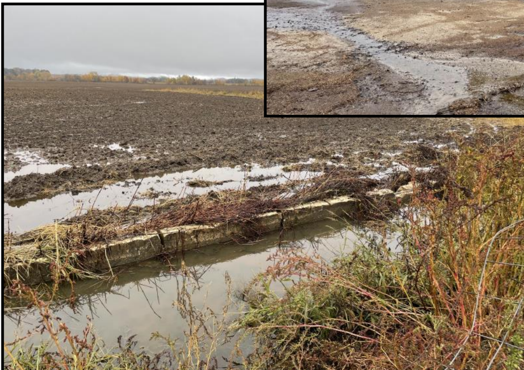
Photo 4 (Bottom Left): Looking east at the runoff spreader bar located along the east edge of the abandoned calf hutch area pictured in photo 3. Runoff from the surrounding area can still be seen pooling in front of the concrete spreader bar. The observed material was cloudy and greenish brown in color.
