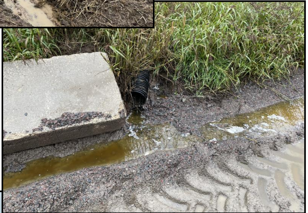
Photo 17 (Right): Looking at an outlet to a tile line or culvert which runs underneath the feed storage area just off the east side of the feed storage. The contents discharging from this outlet mainly flow south toward the runoff collection tank near the south east corner of the feed storage. However, some of the material from this outlet can also be seen along the east edge of the feed storage heading north.
