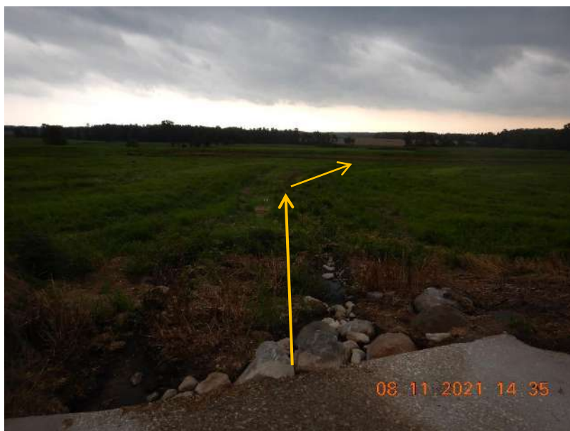
Photo 90. The toe drain where runoff overflows from the leachate basin and gravity flows to the detention basin. The yellow arrows represent the flow path of runoff. This photo was taken facing south.
