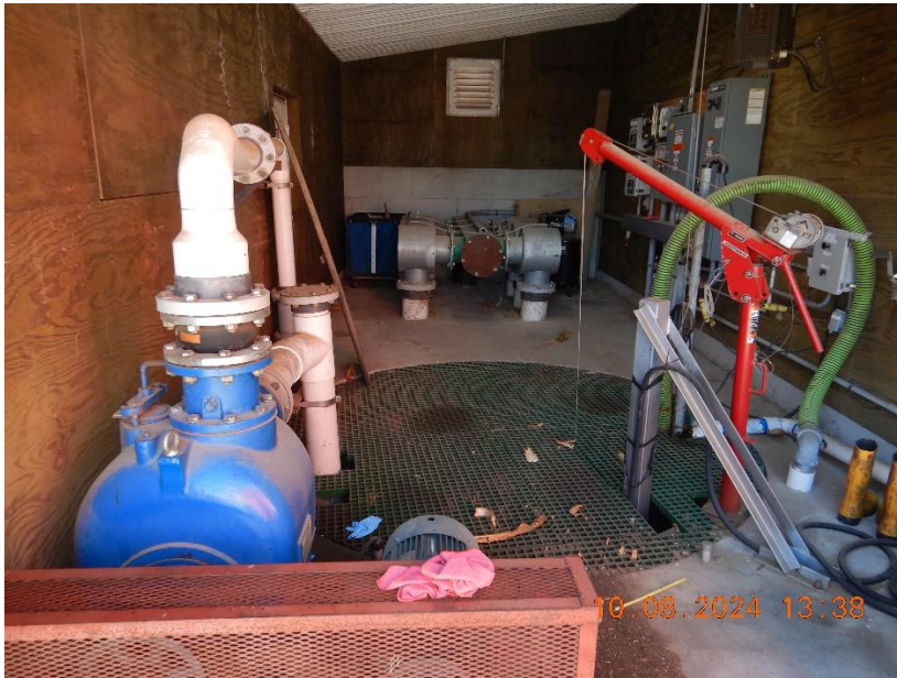
Photo 60. The pump station associated manure transfer system for the milking parlor at the Main Site.
