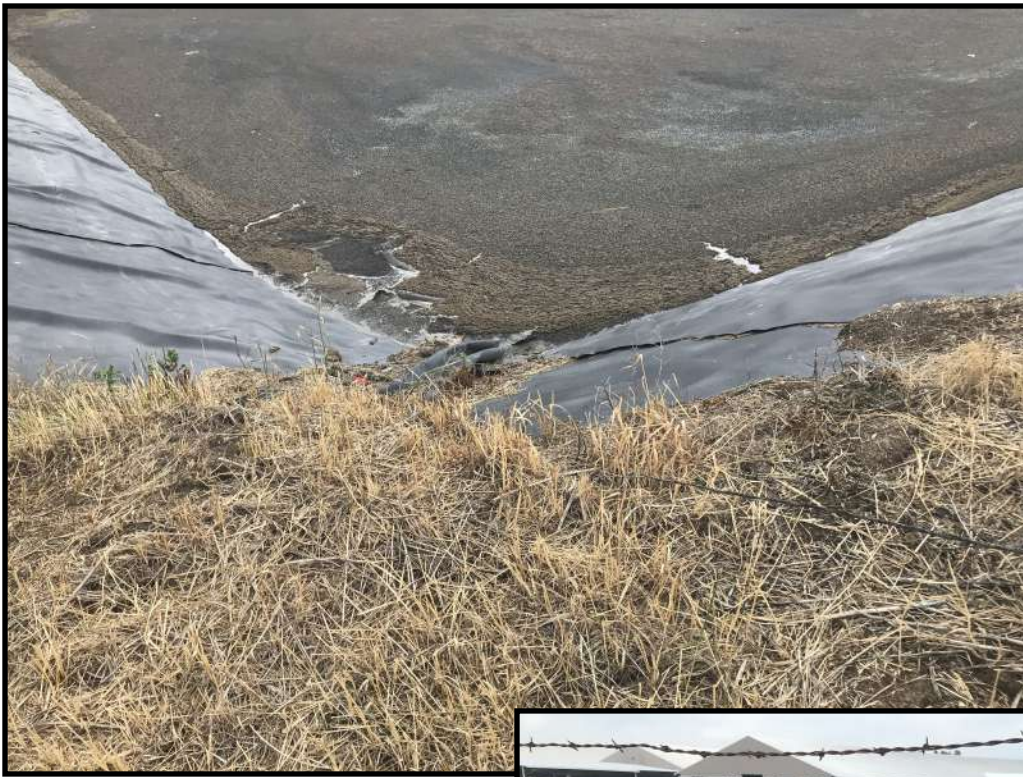
Photo 3 (left): Looking at the north west corner of WSF 1. Rippling within the HDPE liner was observed in this corner of the storage.
