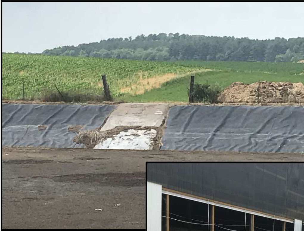
Photo 14 (left): Looking south west at the western side of WSF 1. A pile of waste feed (pictured right) can be seen on the bare ground just west the storage facility. A permanent MOL marker can also be seen painted in white on the concrete ramp.
