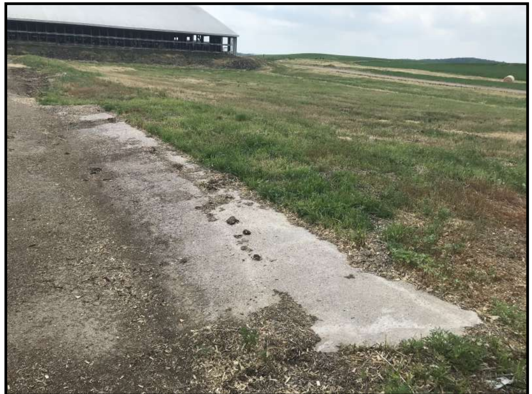
Photo 8 (right): Looking at the west end of the concrete area between the feed pad and the feed bunkers that was reconstructed as part of the interim runoff controls. A concrete lip has been installed to prevent runoff from leaving this end of the feed storage.
