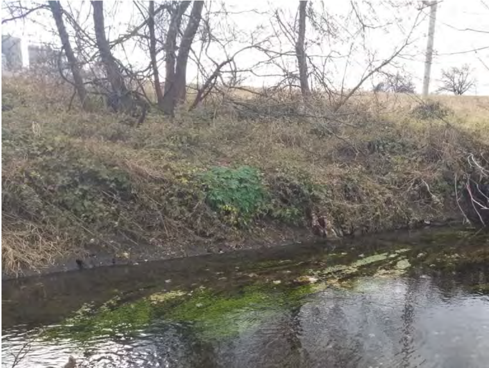
SEGMENT 3 – Bare banks with some root exposure.
