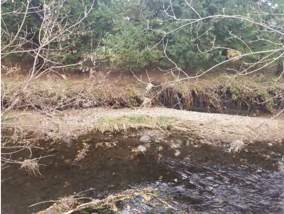
SEGMENT 5B – Slumping soil, exposed banks, vegetative overhang.
