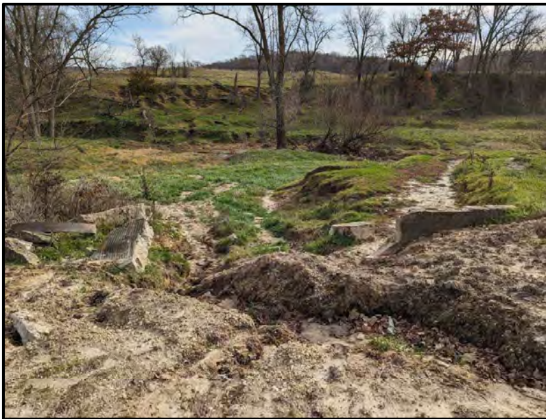
Figure 5: Dutch Creek Stream Crossing Erosion.
