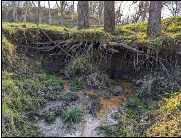
Figure 6: Outlet Area Erosion.
