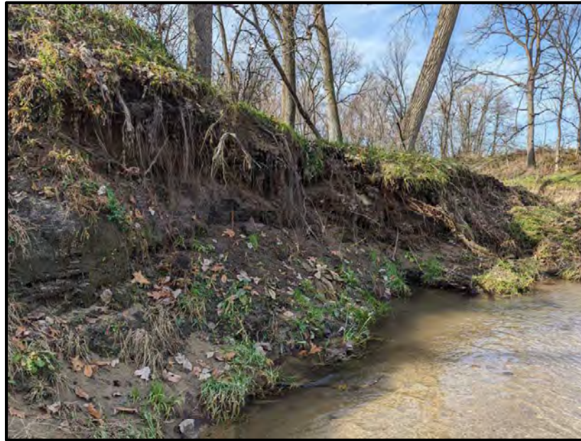
Figure 3: Dutch Creek Streambank Erosion on Halama Property.
