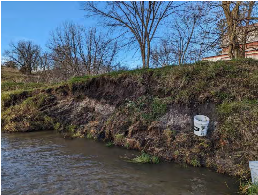
Figure 9: Bank 1 North Side Straight On
