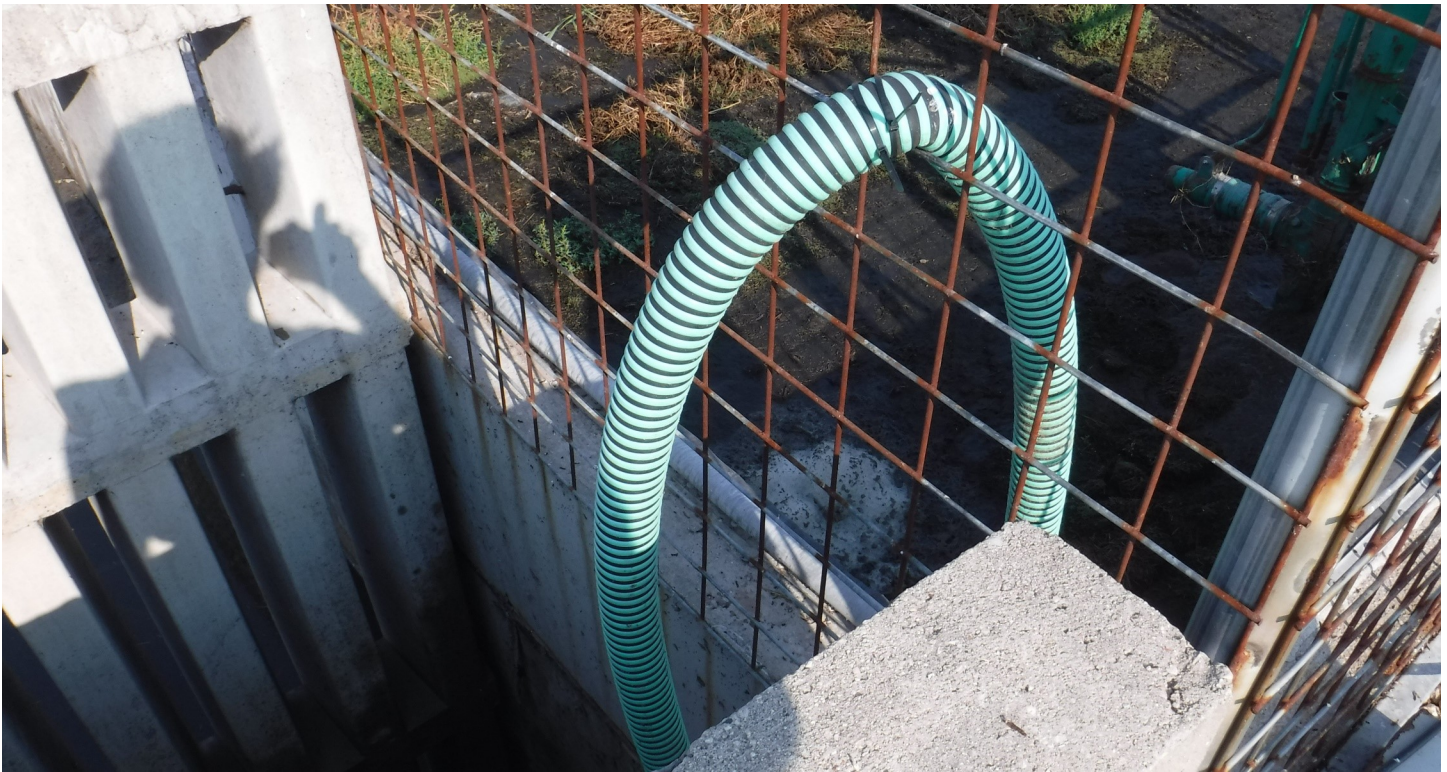
Photo #: 5766 Photo Description: Close-up transfer line in Photo 5765 and its outlet to the concrete liquid manure storage Date/Time of Photo: 8-26-21 / AM Photo Location: Calf Source Photo By: Uvaas
