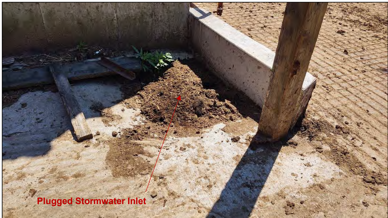
Figure 28: Photograph of plugged stormwater inlet Lot #3 taken on June 27, 2022
