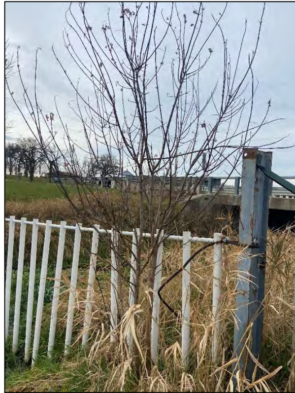
Figure 30: Photograph of tree growing in the west side flood gate taken on November 20, 2023
