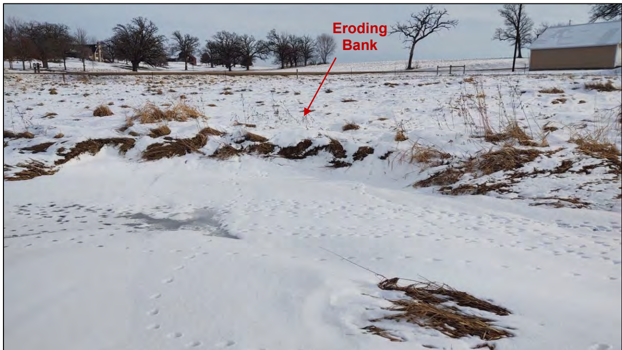
Figure 12: Photograph of new eroding streambank between banks W33 and W34 taken on December 28, 2022
