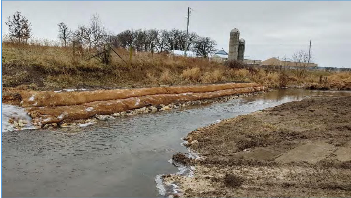
Figure 5: Photograph from December 2019 of bank S1, still under construction. This bank is being stabilized with riprap, vegetated reinforced soil (VRSS) lifts, and live cuttings. Top of bank yet to be fully completed.
