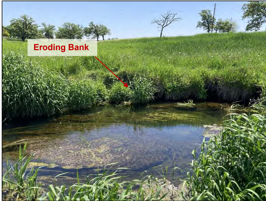
Figure 4-3: Photograph of eroding streambank between banks W33 and W34 (RBFD) taken on May 26, 2023
