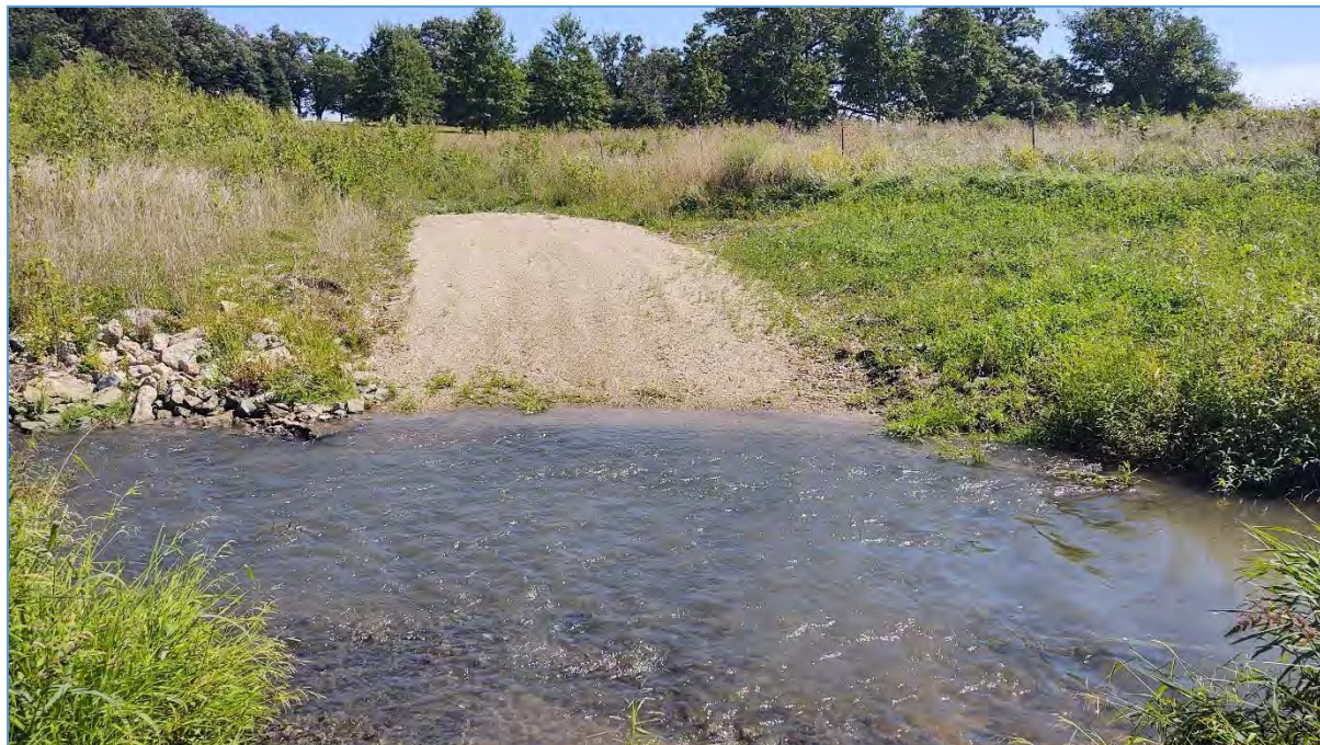
Figure 16: Photograph of a stream crossing (ford) installed near bank S1. A total of three (3) rock crossings were installed at Site B to allow safe crossing of the stream by agricultural equipment and livestock.
