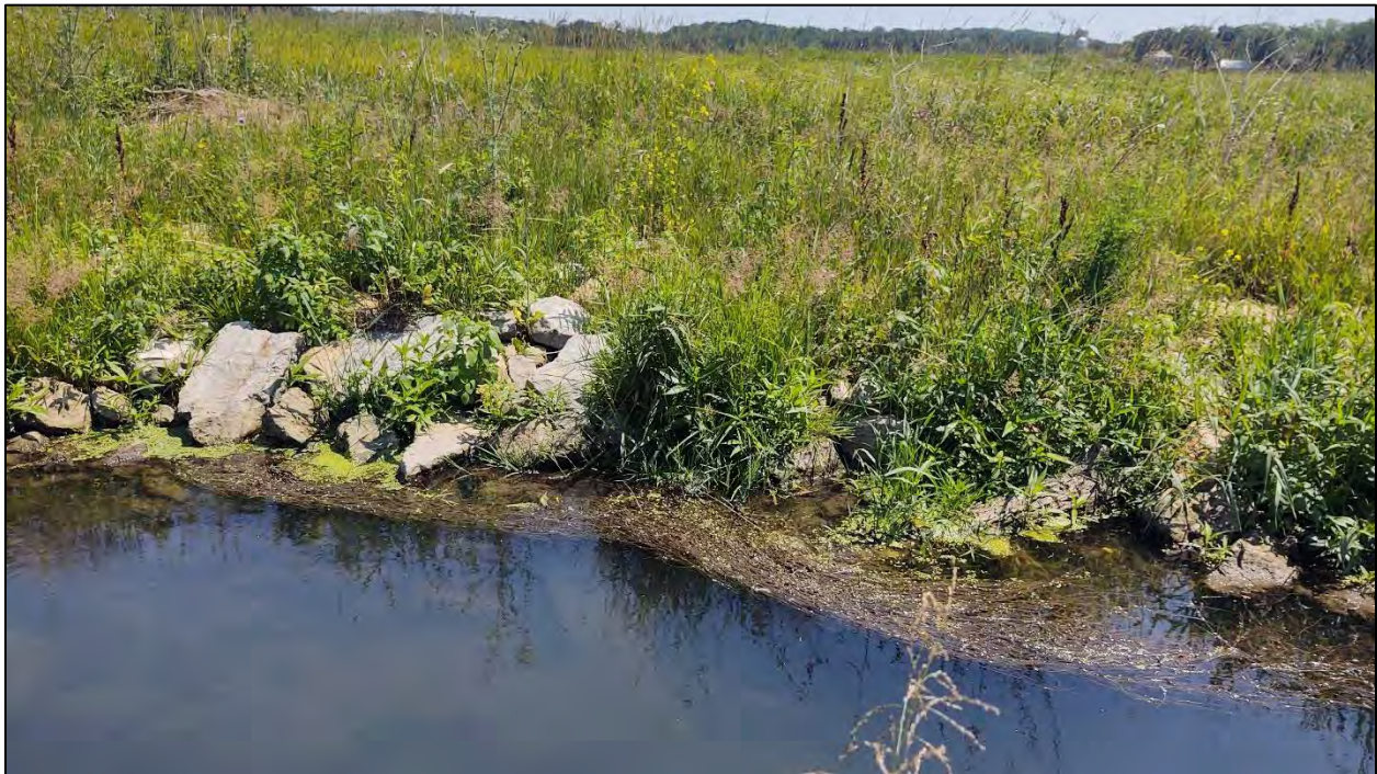
Figure 6: Photograph of Streambank W14 on July 1, 2021
