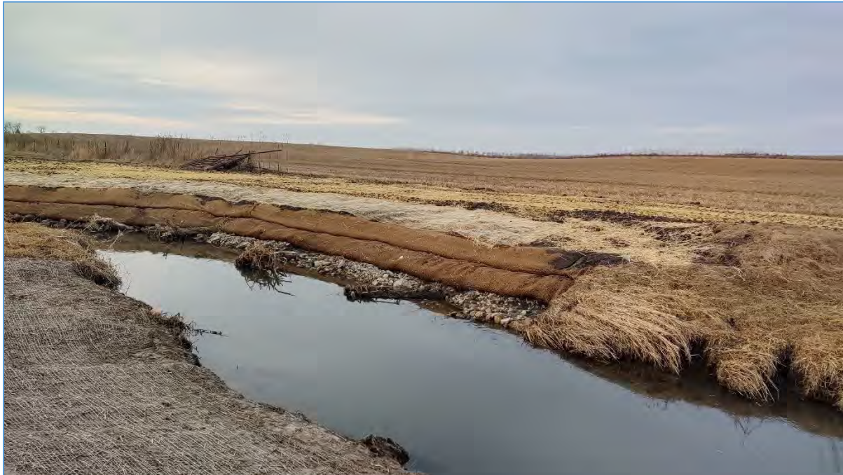
Figure 2: Photograph from December 2019 of bank W28. Site was stabilized using a combination of riprap and vegetated reinforced soil (VRSS) lifts. Willow live cuttings and root wads were added to further stabilize the site and provide woody aquatic habitat.
