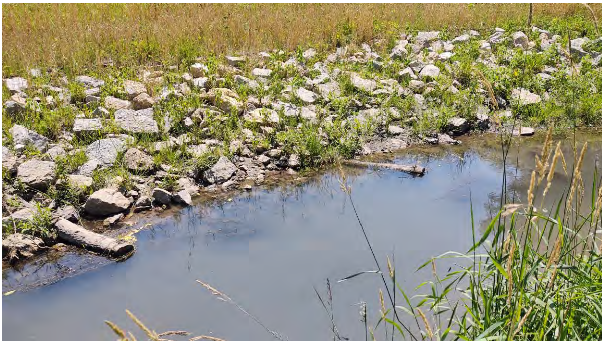
Figure 14: Photograph of escape logs (aquatic habitat) installed along bank S17. A total of seven (7) escape logs and two (2) root wad log revetments were installed at Site B.
