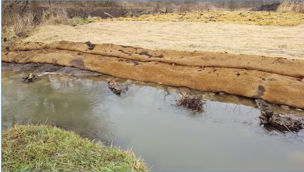
Figure 7: Photograph from December 2019 of bank S21. This site was stabilized using riprap, vegetated reinforced soil (VRSS) lifts, willow live cuttings, and root wads.
