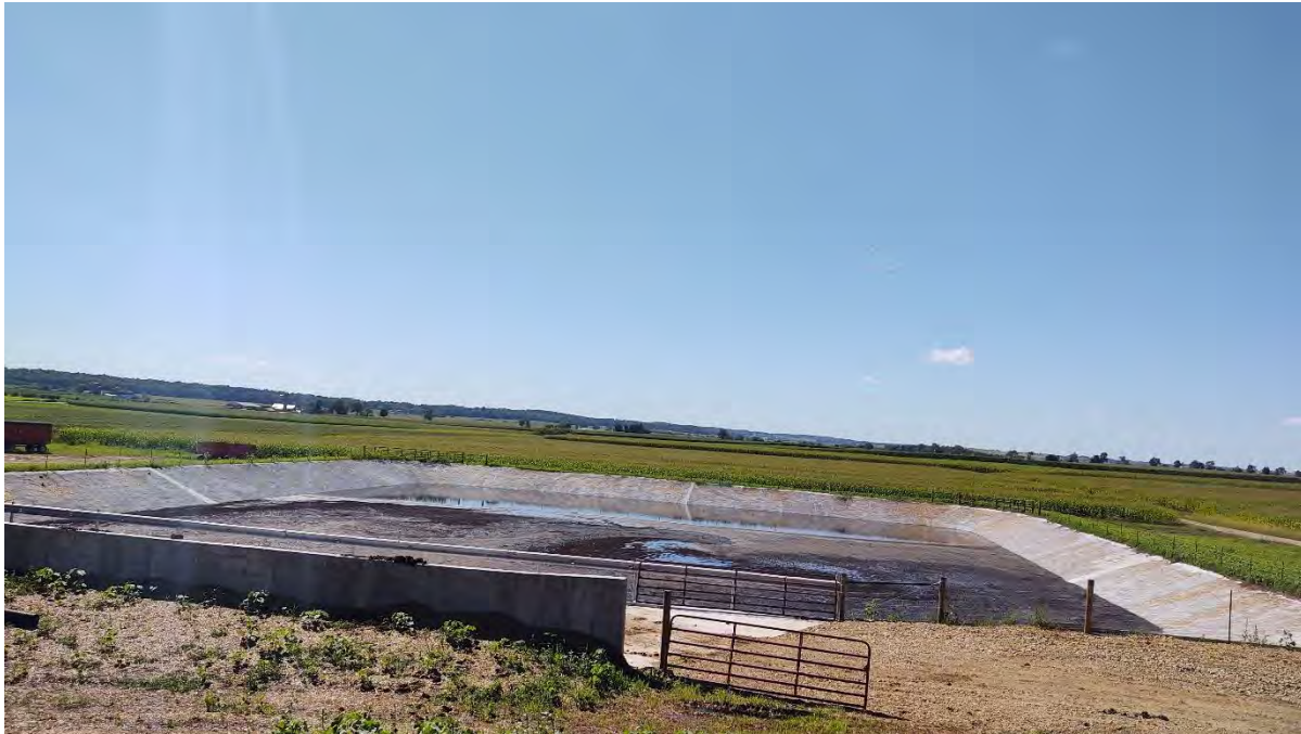
Figure 23: Photograph of the new waste storage facility. The facility will provide greater than 180-days of manure storage for Landowner C. Runoff from Lots #2 and #3 will be diverted to the new storage. This manure storage is significantly larger than the Landowner's previous, which only provided 2-weeks of storage capacity. The new waste storage will allow the landowner to avoid frequent hauling of manure to crop fields in winter to frozen or snow covered ground and apply the manure at less sensitive times of the year.
