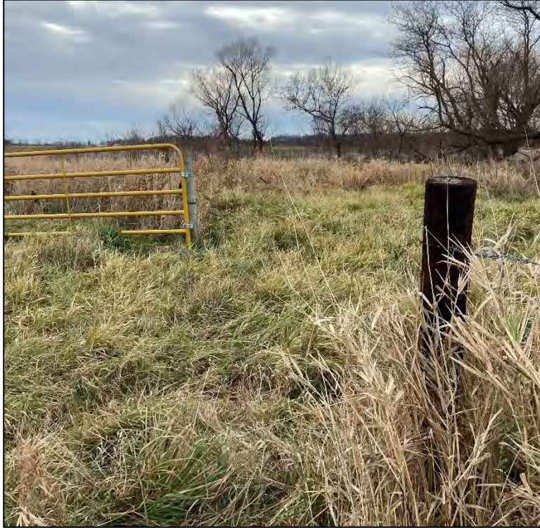
Figure 4-7: Photograph of leaning gate posts on west side of property taken on November 20, 2023
