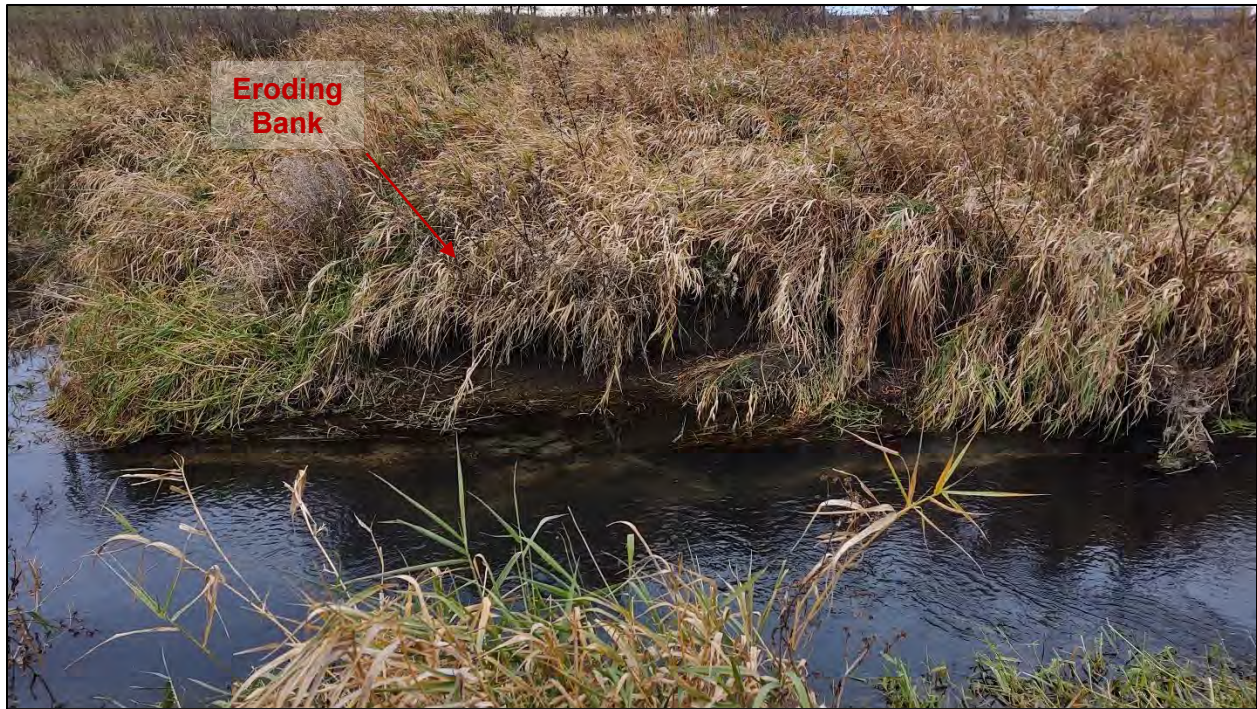
Figure 22: Photograph of new eroding streambank between banks S4 and S6 on November 15, 2021
