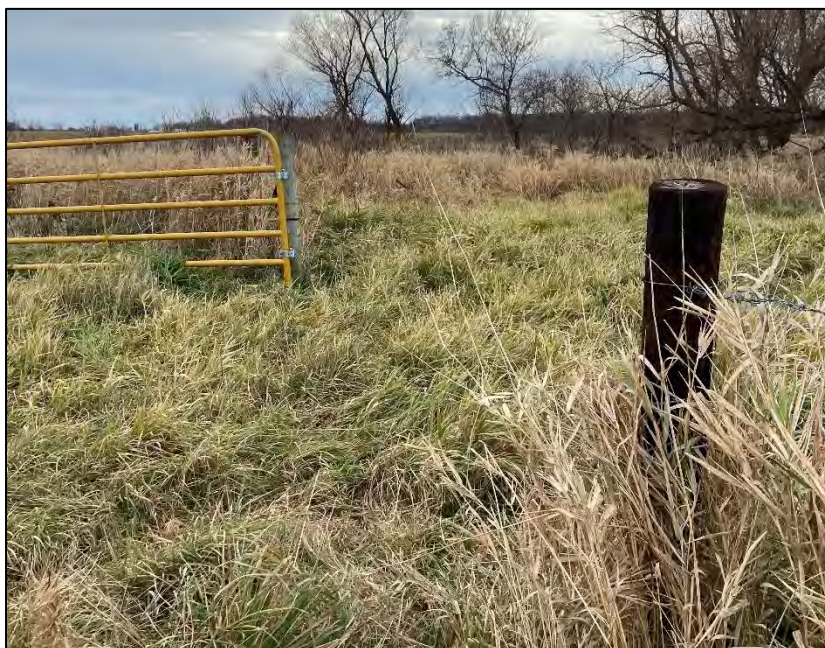
Figure 13: Photograph of leaning gate posts on west side of property taken on November 20, 2023.
