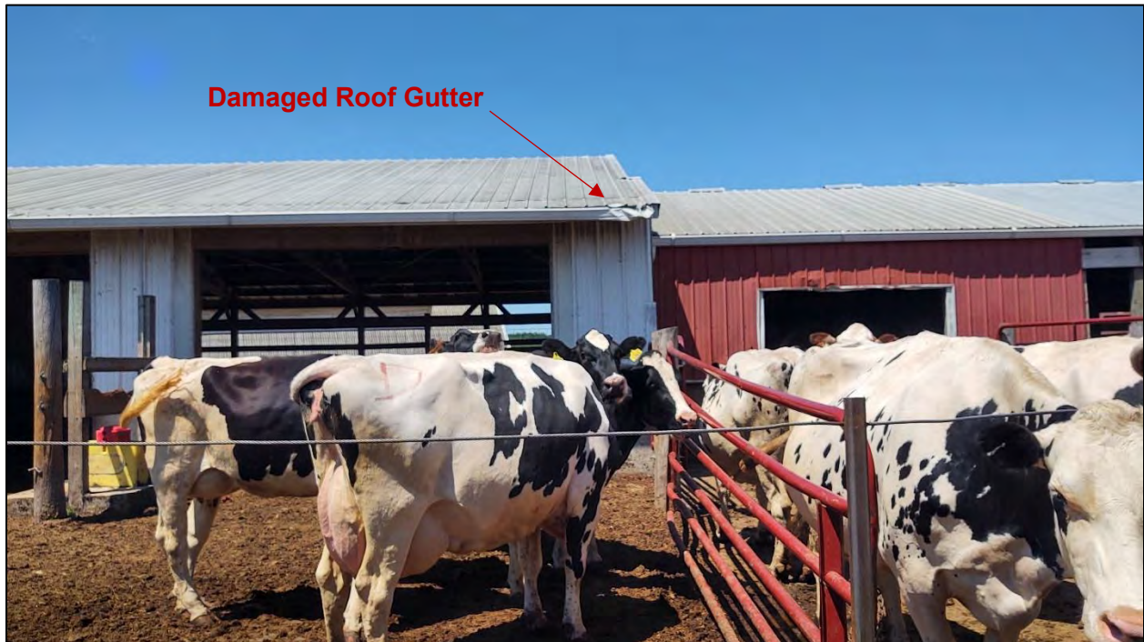
Figure 26: Photograph of damaged roof gutter for Lot #3 taken on June 27, 2022
