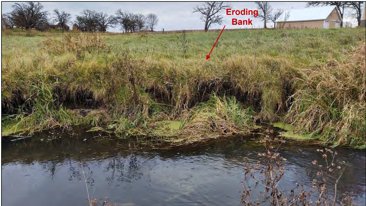
Figure 10: Photograph of new eroding streambank between banks W33 and W34 taken on November 15, 2021
