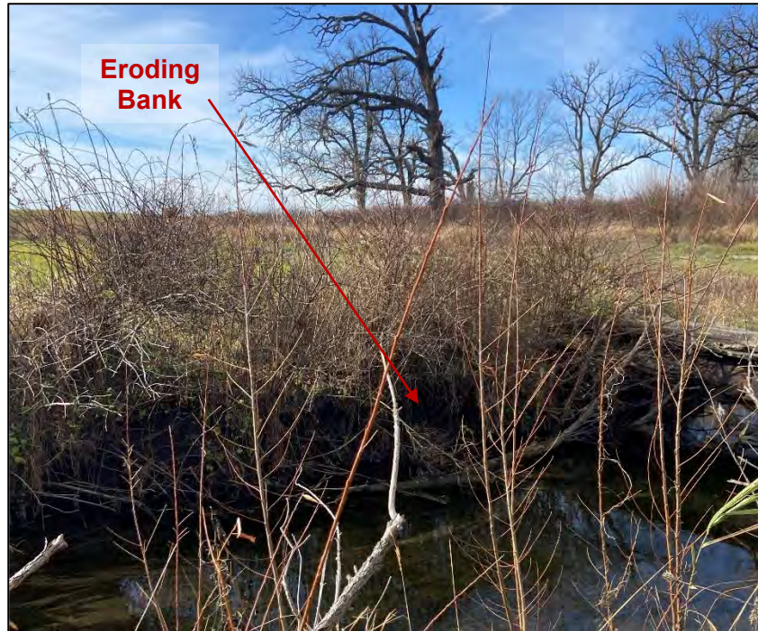
Figure 28: Photograph of new eroding streambank opposite S14 taken on November 20, 2023
