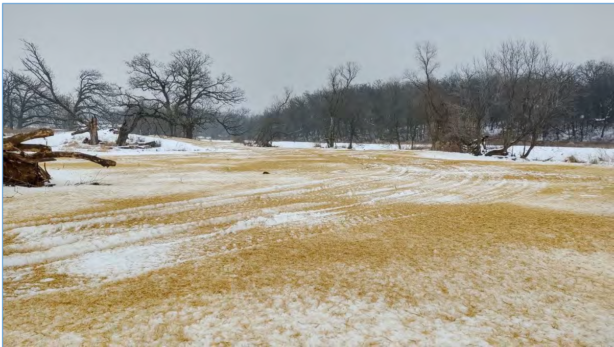
Figure 8: Photograph from January 2020 displaying the main mobilization area located on Site B. All soil piles have now been removed from the site or evenly spread in designated areas. Contractor has attempted to seed and mulch the site despite current snow cover.
