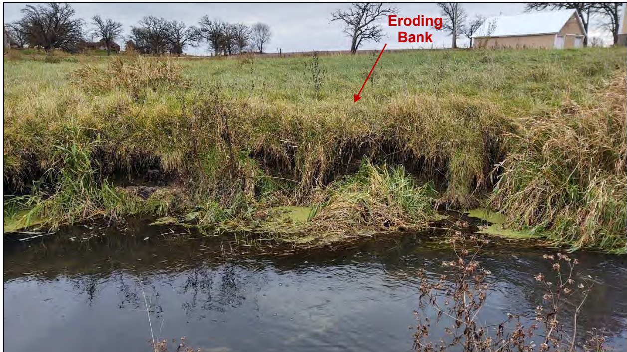
Figure 10: Photograph of new eroding streambank between banks W33 and W34 taken on November 15, 2021
