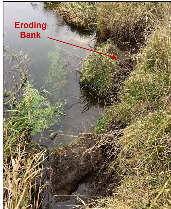
Figure 12: Photograph of new eroding streambank between banks W33 and W34 taken on November 20, 2023.
