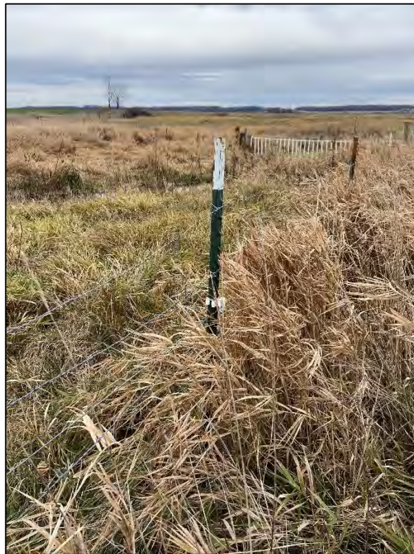
Figure 14: Photograph of leaning fence posts on west side of property taken on November 20, 2023.
