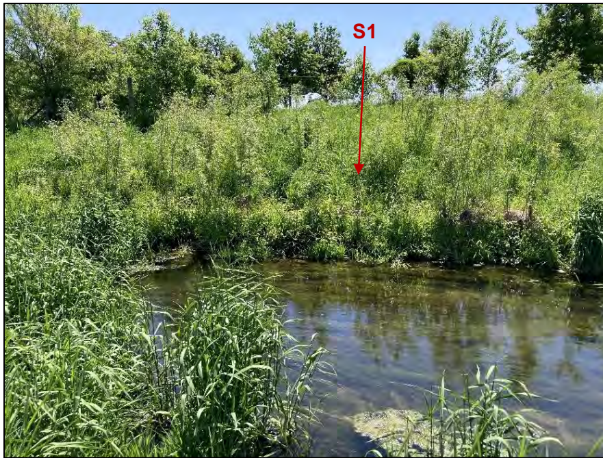
Figure 16: Photograph of Streambank S1 on May 26, 2023
