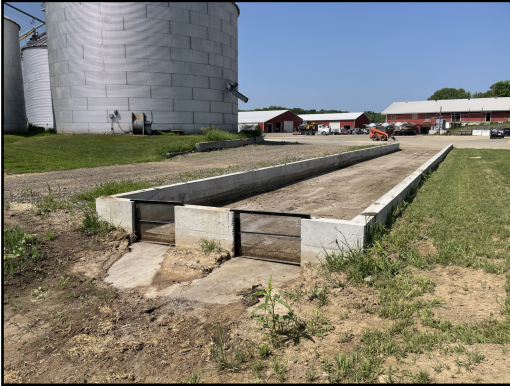
Photo 13 (Left): Looking west at the concrete storm water sediment basin located off the north east corner of the feed pad. Storm water from the rooftops and concrete areas just north of the first feed storage runoff collection tank (pictured in photo 11) flows into the sediment basin. Sediment is then trapped within the basin and remaining storm water is slowly filtered out through the screens where it proceeds through the grassed waterway pictured in photo 14.
