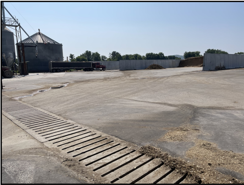
Photo 11 (Left): Looking at the first stage feed storage runoff collection tank located at the north end of the feed storage area. Leachate and feed storage runoff flows north across the pad and first enters this collection tank where it then gravity flows to the second collection tank pictured in photo 12.
