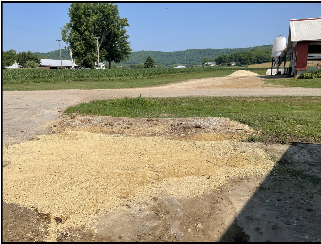
Photo 3 (Left): Looking at the gravel berm that was installed in front of the culvert inlet located off the west end of the outdoor concrete lot.
