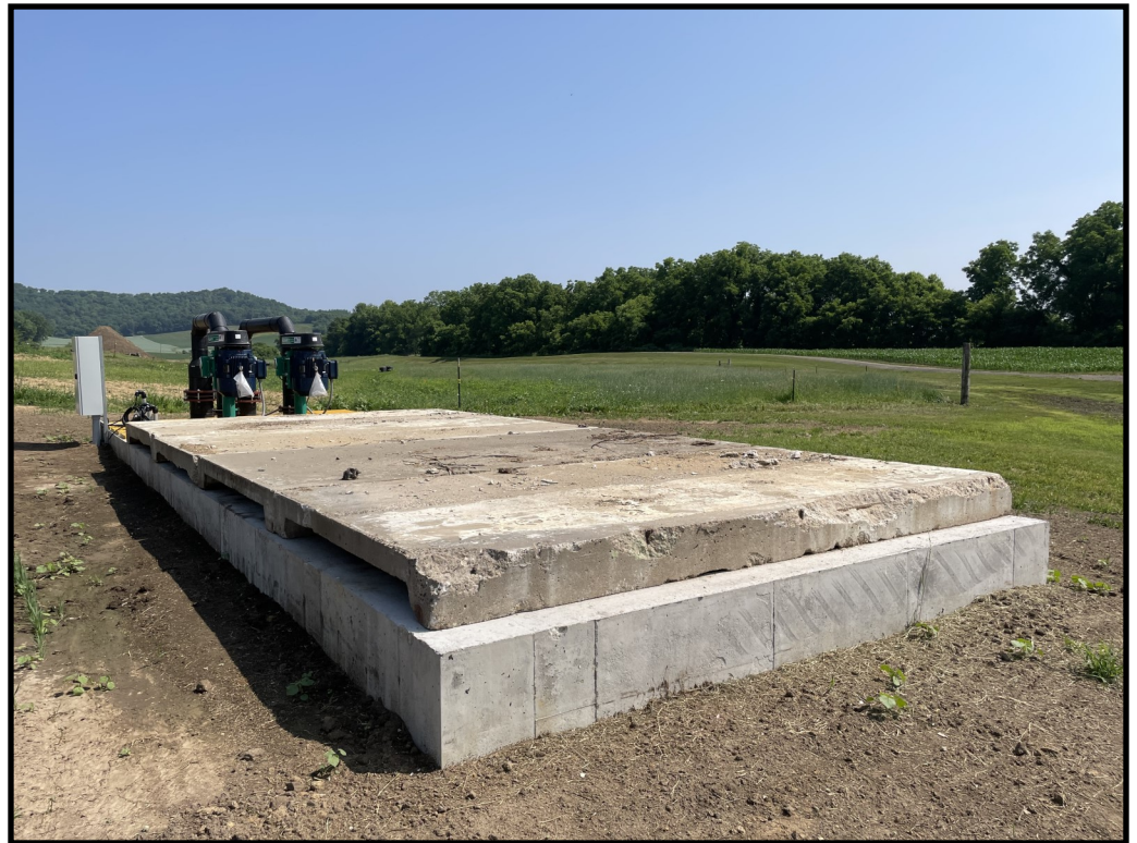
Photo 12 (Right): Looking at the second stage feed storage runoff collection tank. Leachate and feed storage runoff within this collection tank is pumped to WSF 1.
