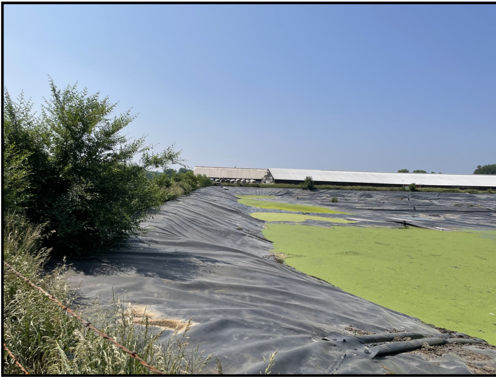
Photo 7 (Left): Looking south along the eastern wall of WSF 1. Considerable tree growth was present along the outer bank of this wall.
