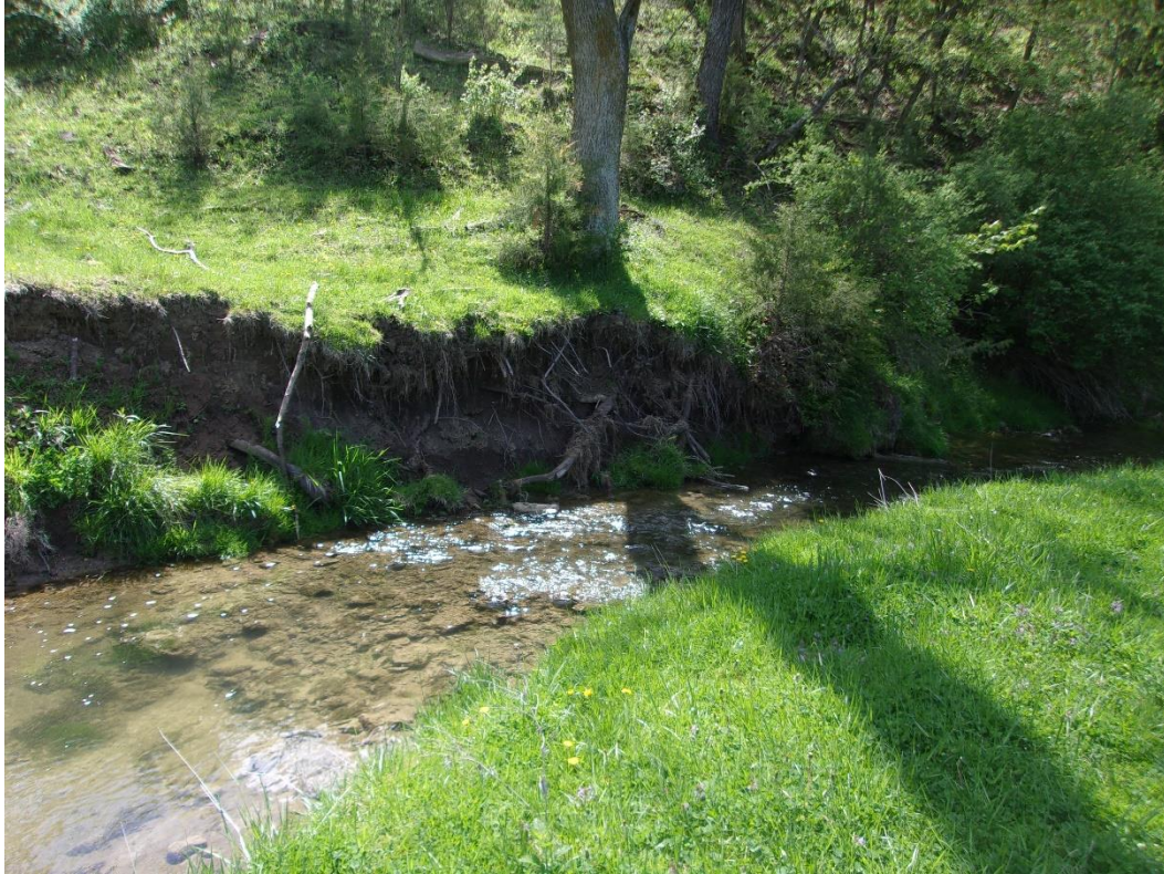
Image 7 – Severe undercut with slump, vegetative overhang, and exposed tree roots
