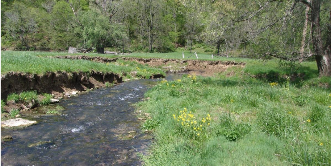
Image 18 – Severe undercut with slump and vegetative overhang
