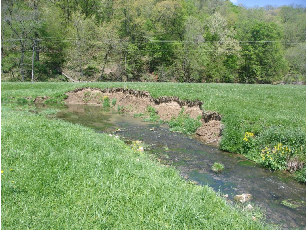
Image 1 – Severe undercut with slump and vegetative overhang
