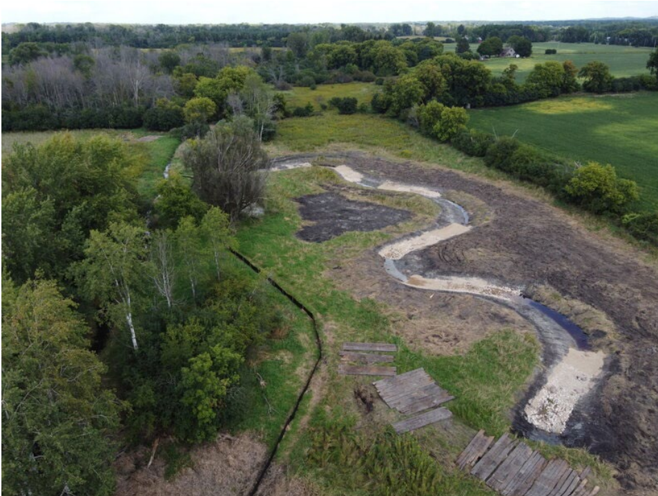
FIGURE F5: AERIAL IMAGE OF MASON CREEK RESTORATION MID-CONSTRUCTION. THE CHANNELIZED DITCH IS VISIBLE IN THE LEFT OF THE PHOTO, WHILE THE RESTORED/RECONSTRUCTED CHANNEL IS VISIBLE FOLLOWING THE ORIGINAL COURSE OF THE CREEK, AS IDENTIFIED FROM HISTORIC SURVEYS AND FIELD INVESTIGATION. NATURAL CHANNEL DESIGN FEATURES, FISH HABITAT (ENGINEERED RIFFLES, POOLS, ETC.), AND NATURAL DESIGN ELEMENTS WERE USED IN THIS PROJECT TO FULLY RESTORE MASON CREEK TO A NATURAL CONDITION AS A COLD-WATER TROUT STREAM (PHOTO CREDIT: TALL PINES CONSERVANCY)
