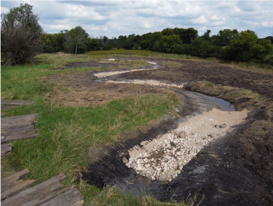
FIGURE F6: CLOSE-UP IMAGE OF MASON CREEK RESTORATION PROJECT, SHOWING AN ENGINEERED RIFFLE-POOL SEQUENCE WITH NATURAL STREAM MEANDERS AND CHANNEL METRICS FOLLOWING THE ORIGINAL CHANNEL. NATIVE VEGETATION AND BIOENGINEERING PRINCIPLES WERE USED TO STABILIZE STREAMBANKS, PROVIDE SHADING, AND COMPLETE THE RIPARIAN RESTORATION COMPONENT OF THIS NATURAL STREAM RESTORATION PROJECT.
