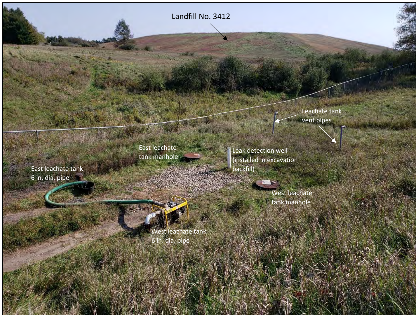
Photo 5: East and West leachate tanks, looking southeast. The East Tank collects leachate from Landfill No. 2638, and the West Tank collects leachate from Landfill No. 3171. Tanks are pumped via 6-inch pipe as shown.
