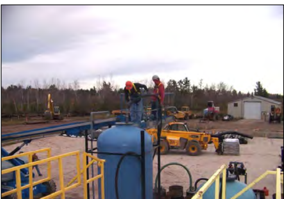
2 CARBON CHANGE OUT IN WATER TREATMENT SYSTEM.
