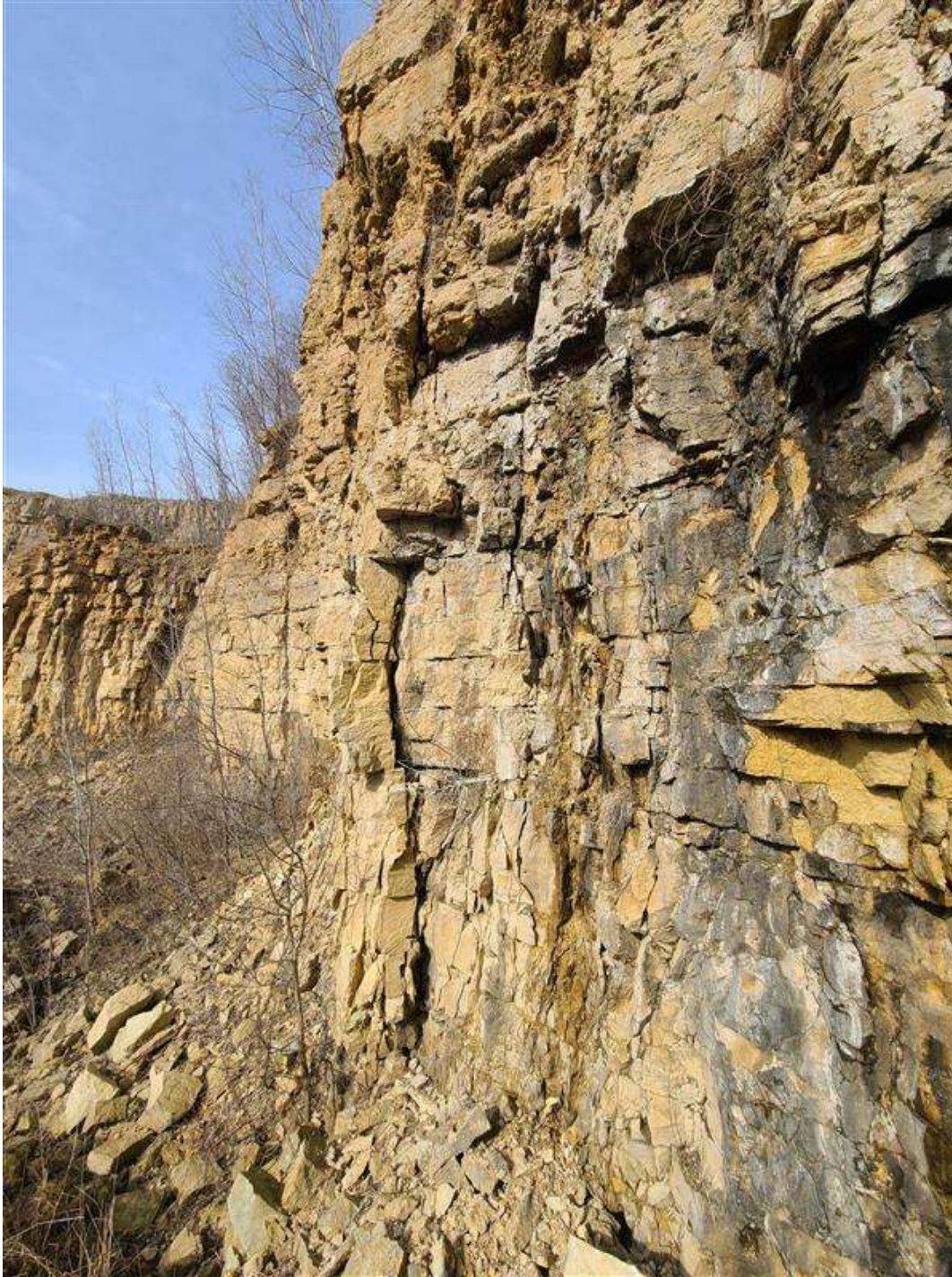
Photo 8 (SEH, April 2026) Seas Branch Quarry – Larger fractures (primarily vertical) are the result of natural separation of the rock along the exposed quarry wall. While natural fractures are present, the rock surface within the fracture did not contain evidence of mineral precipitates or secondary porosity. As a result, the larger fractures/cavities are recent, likely the result of historic mining operations (blasting/excavation) as well as the freeze-thaw process accelerating weathering of bedrock along exposed quarry walls.
