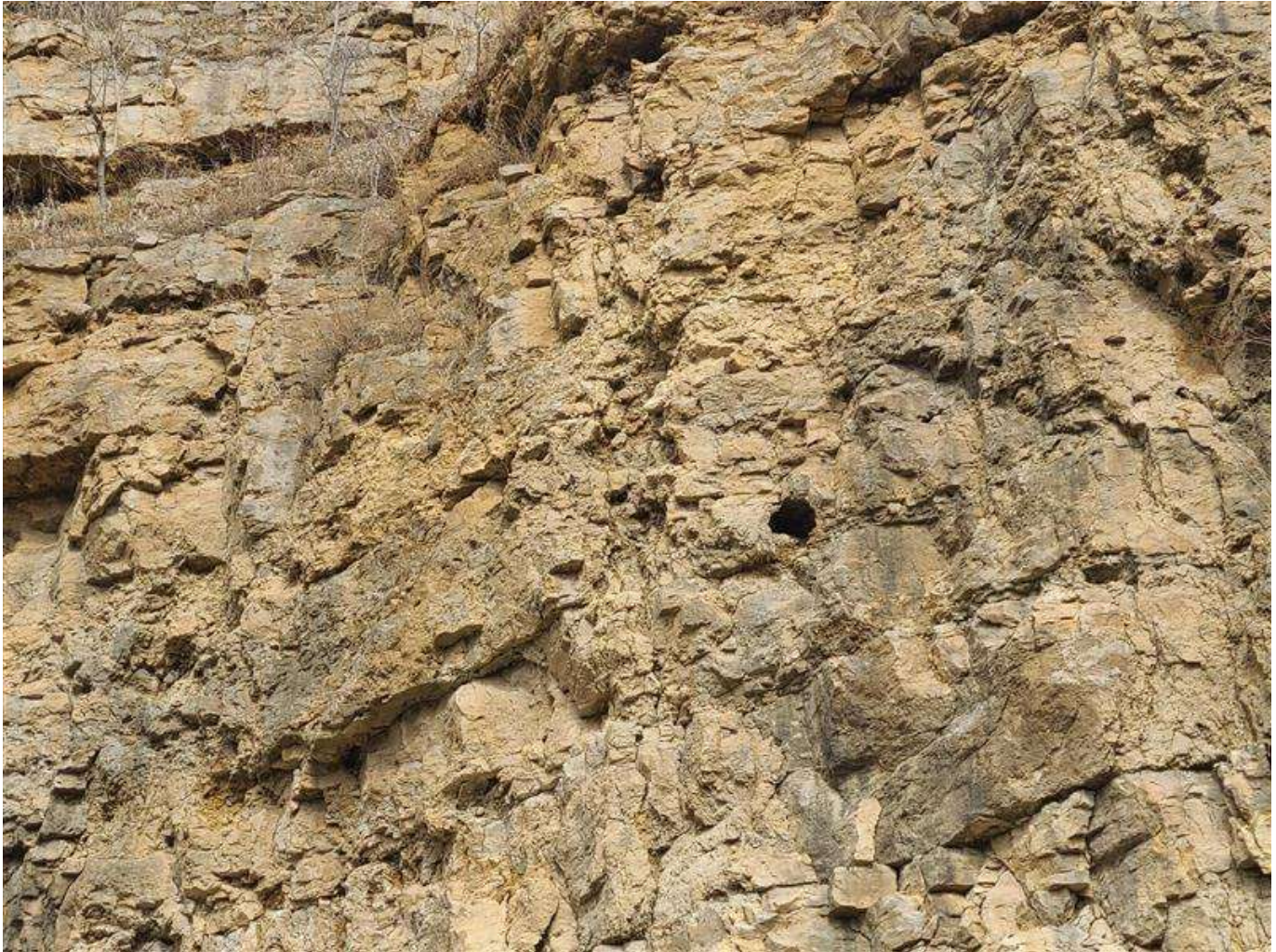
Photo 7 (SEH, April 2026) Seas Branch Quarry – Closer view of fractures/cavities in the upper bedrock layer of the Oneota Dolomite. While natural fractures are present, the rock surface within the fracture did not contain evidence of mineral precipitates or secondary porosity. As a result, the larger fractures/cavities are likely the result of historic mining operations (blasting/ excavation) as well as accelerated weathering of bedrock along exposed quarry walls.
