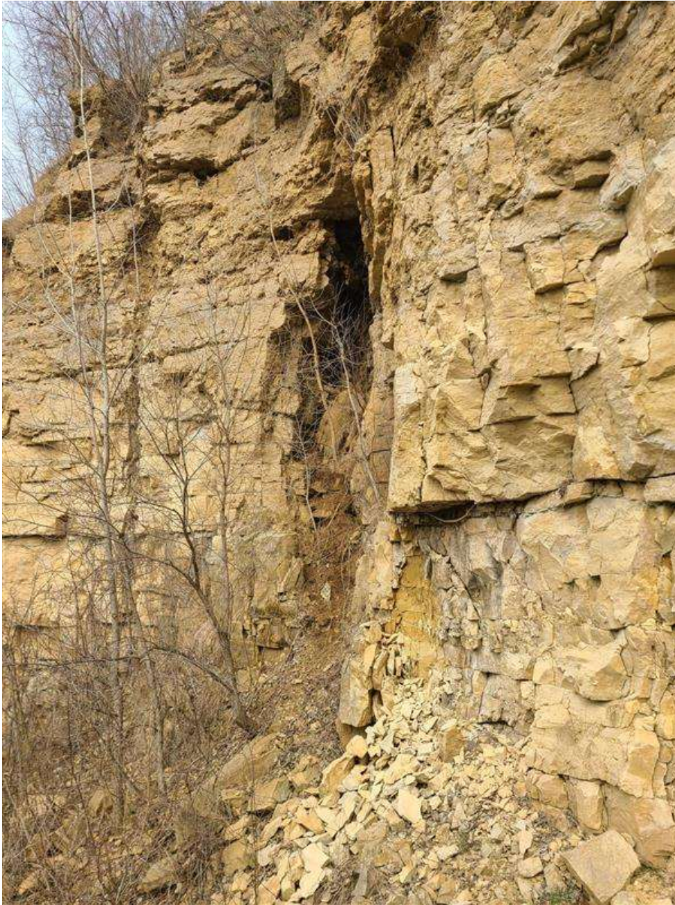
Photo 9 (SEH, April 2026) Seas Branch Quarry – Larger fractures (primarily vertical) are the result of natural separation of the rock along the exposed quarry wall. While natural fractures are present, the rock surface within the fracture did not contain evidence of mineral precipitates or secondary porosity. As a result, the larger fractures/cavities are recent, likely the result of historic mining operations (blasting/ excavation) as well as the freeze-thaw process accelerating weathering of bedrock along exposed quarry walls. Rockfall from weathering continues within the void space, with recent colluvium being deposited along the base of the quarry wall, fanning out from the void.
