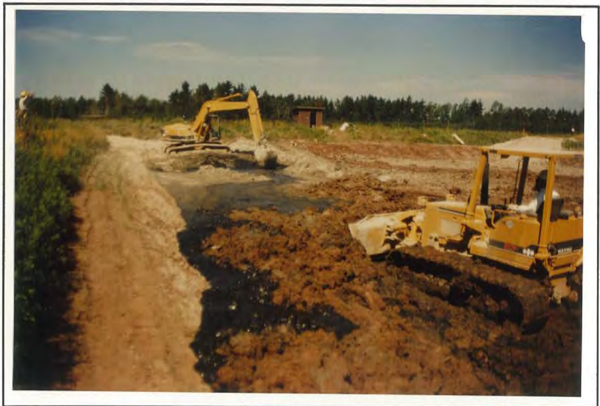
PHOTO 14 SLUDGE MIXING - S.W. CORNER
