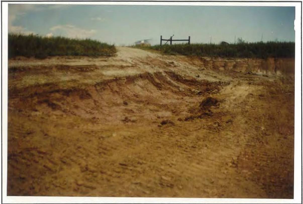
PHOTO 9 DEEPER SEEPAGE - N.E. CORNER
