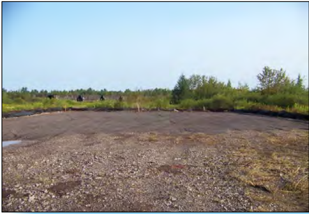
4 AREA F2 AFTER 2.5 INCHES OF RAIN; NO SETTLEMENT IN AREA.
