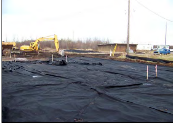
4 SUBGRADE OPERATIONS IN AREA B CONTINUE. GEOTEXTILE IS DEPLOYED PRIOR TO SOIL COVER INSTALLATION.
