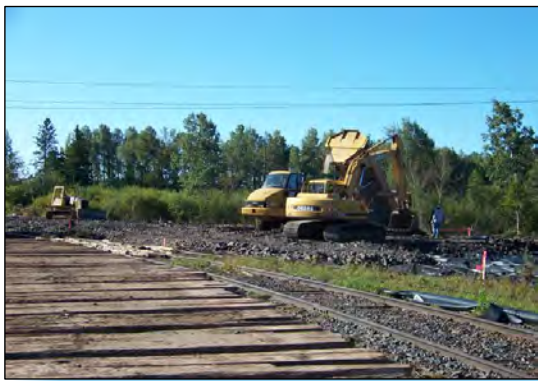
4 PLACEMENT OF GEOTEXTILE AND STONE FOR BRIDGING IN AREA G IS COMPLETED TODAY.
