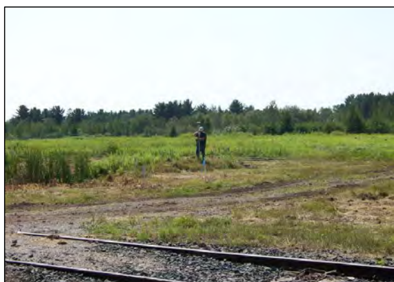
2 SURVEYOR ONSITE TO BEGIN LAYING OUT WORK AREAS AND TOPO OF EXISTING CONDITIONS.
