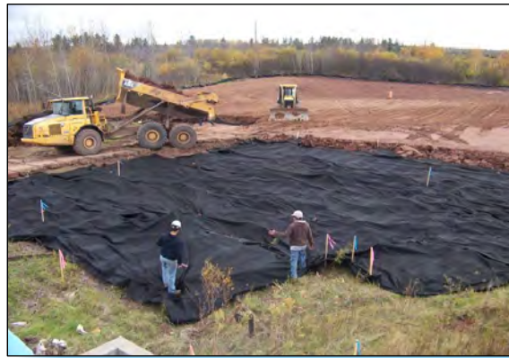
2 CREW DEPLOYS GEOTEXTILE PRIOR TO CLAY GENERAL FILL PLACEMENT IN AREA B.
