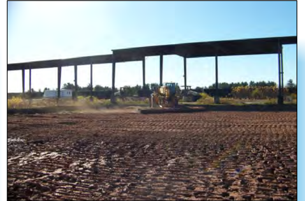
6 MATS ARE MOVED TO SOUTHERN END OF AREA B IN PREPARATION FOR TOPSOIL PLACEMENT.
