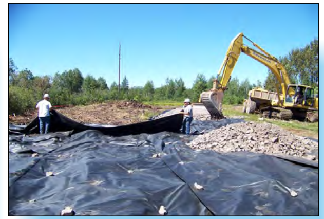
3 INSTALLATION OF FABRIC AND STONE IN AREA G TO BRIDGE OVER EXTREMELY WET CONDITIONS.
