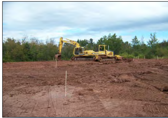
2 CLAY BACKFILL IS ADDED IN AREA H TO CREATE A PITCH FOR DRAINAGE AWAY FROM TRACKS. EXCAVATOR WORKS SLOPE ALONG TRACKS IN PREPARATION FOR TAPER STONE.
