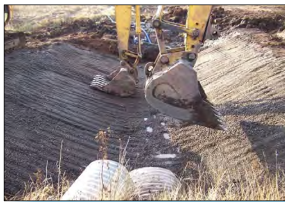
2 SECTION OF OUTFALL DITCH IS EXCAVATED; GRAVEL IS ADDED TO DITCH PRIOR TO RCM.
