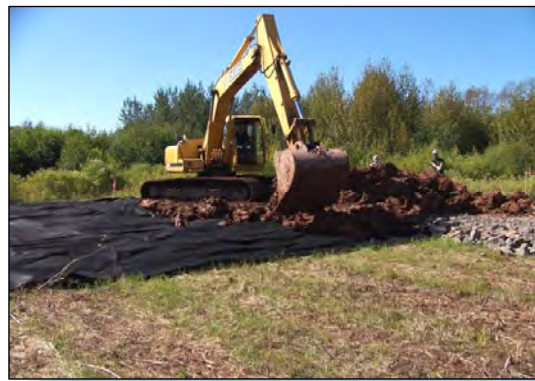
5 EXCAVATOR IS USED TO BEGIN PLACEMENT OF CLAY BACKFILL IN AREA H.
