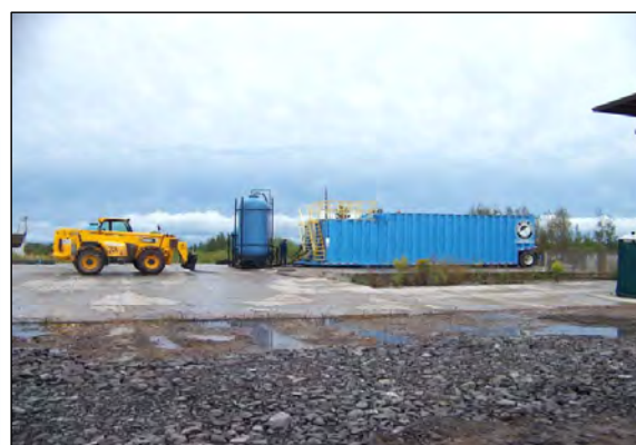
6 CREW STARTS WATER TREATMENT SYSTEM. ON SITE ENGINEER TOOK SAMPLE AND SENT IT OFF.
