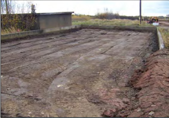
4 IN PREPARATION FOR SUBGRADE FILL PLACEMENT, EXISTING MATERIAL IN CONCRETE BASIN IS STABILIZED.
