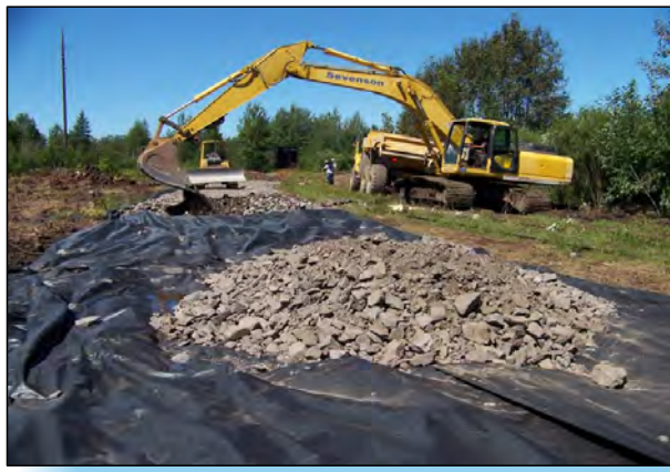
2 INSTALLATION OF FABRIC AND STONE IN AREA G TO BRIDGE OVER EXTREMELY WET CONDITIONS.
