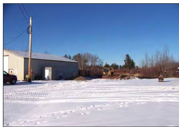
6 STONE IS PLACED NEXT TO SHOP AND AREA IS REGRADED TO PROMOTE DRAINAGE AWAY FROM SHOP.
