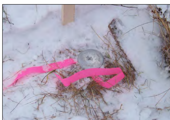
2 SURVEYORS ONSITE TO INSTALL SOIL MARKERS AT CORNERS OF SURFACE COVER AREAS.
