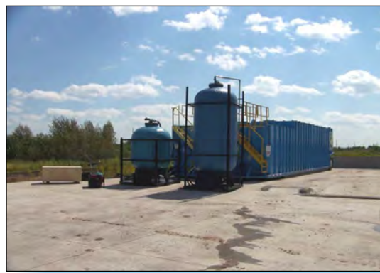
2 WATER TREATMENT SYSTEM IS HOOKED UP AND WILL BE TESTED TUESDAY.
