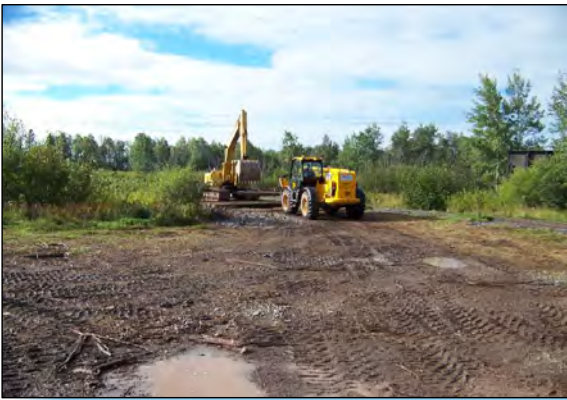
1 DUE TO RAIN OVER THE WEEKEND AREA H WAS TOO WET TO WORK IN SO OPERATIONS WERE MOVED TO AREA G.
