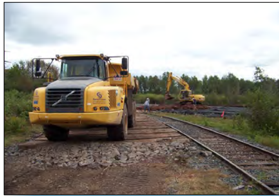
2 CLAY BACKFILL IS PLACED IN AREA G; EXCAVATOR IS USED TO BEGIN INSTALLATION TO PREVENT TEARING GEOTEXTILE.
