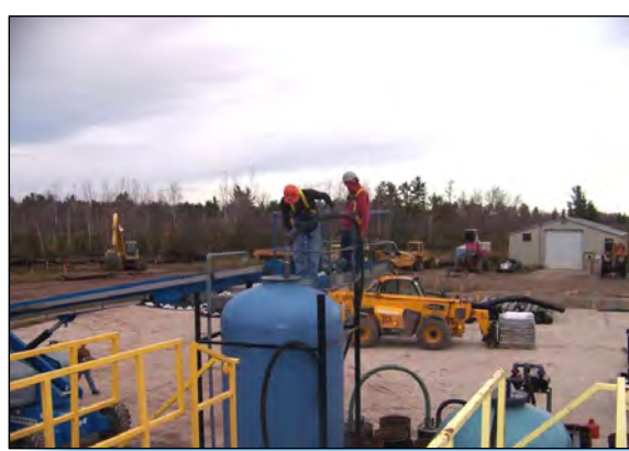
2 CARBON CHANGE OUT IN WATER TREATMENT SYSTEM.
