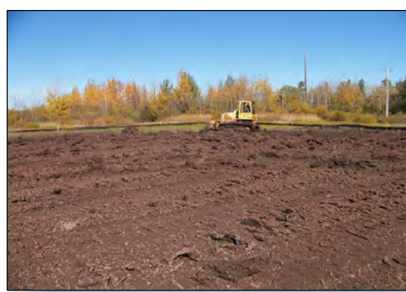
3 MATERIAL CUT FROM AREA B BEING PLACED AND GRADED IN AREA A.
