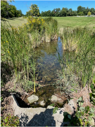
Standing water at outfall during dry weather. Photo Credit: Wisconsin DNR
