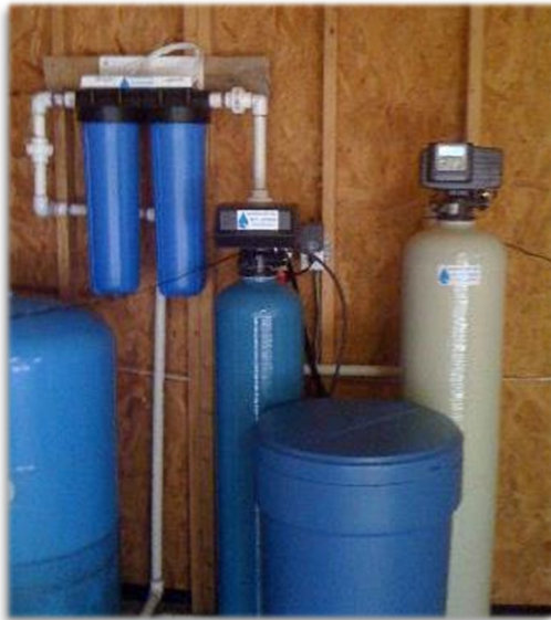
Whole-House Water Softener & Filter
