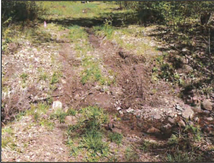
Wetland 12 at Drainageway Crossing - Looking East
