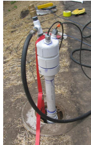
Pumping test at one of Madison's municipal wells, part of a WGRMP-funded study to enhance understanding of fractures and virus transport. Photo: Jean Bahr
