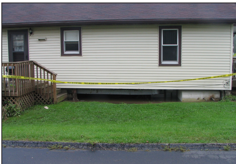
Flood damaged residence in Richland Center
