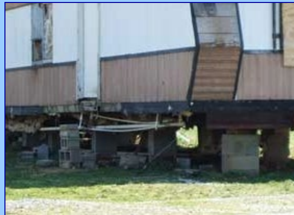
Mobile Home Tie-Downs
