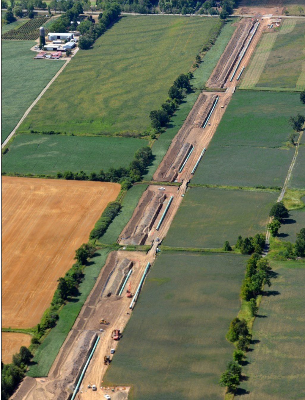
Figure 2.6-3 Aerial photo of construction workspace with pipe staged next to trenches. Photo: Stock image
