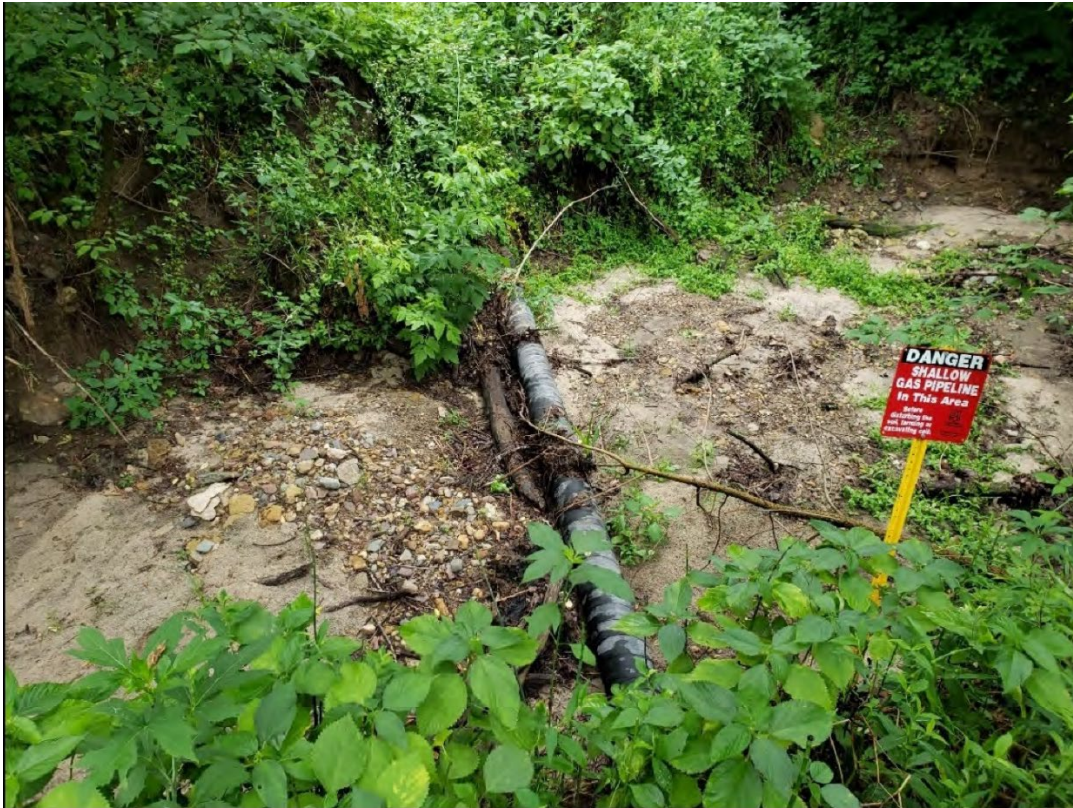
Figure 5.6-14 Northern Natural Gas Black River Falls pipeline exposure.
