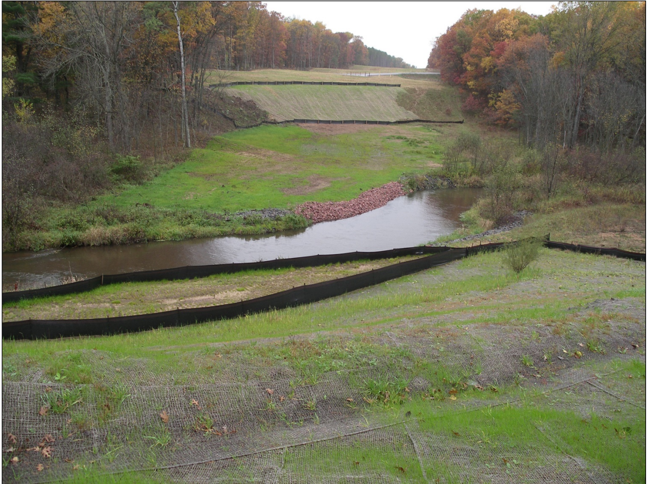
Figure 5.6-9 Examples of erosion control strategies used at a pipeline waterbody crossing mid-restoration.
