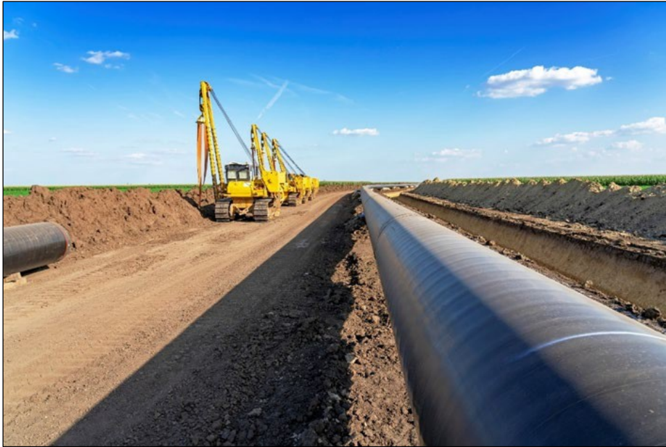
Figure 2.5-1 Pipeline trench installation in an agricultural setting. Excavated material is stockpiled separately from topsoil.
