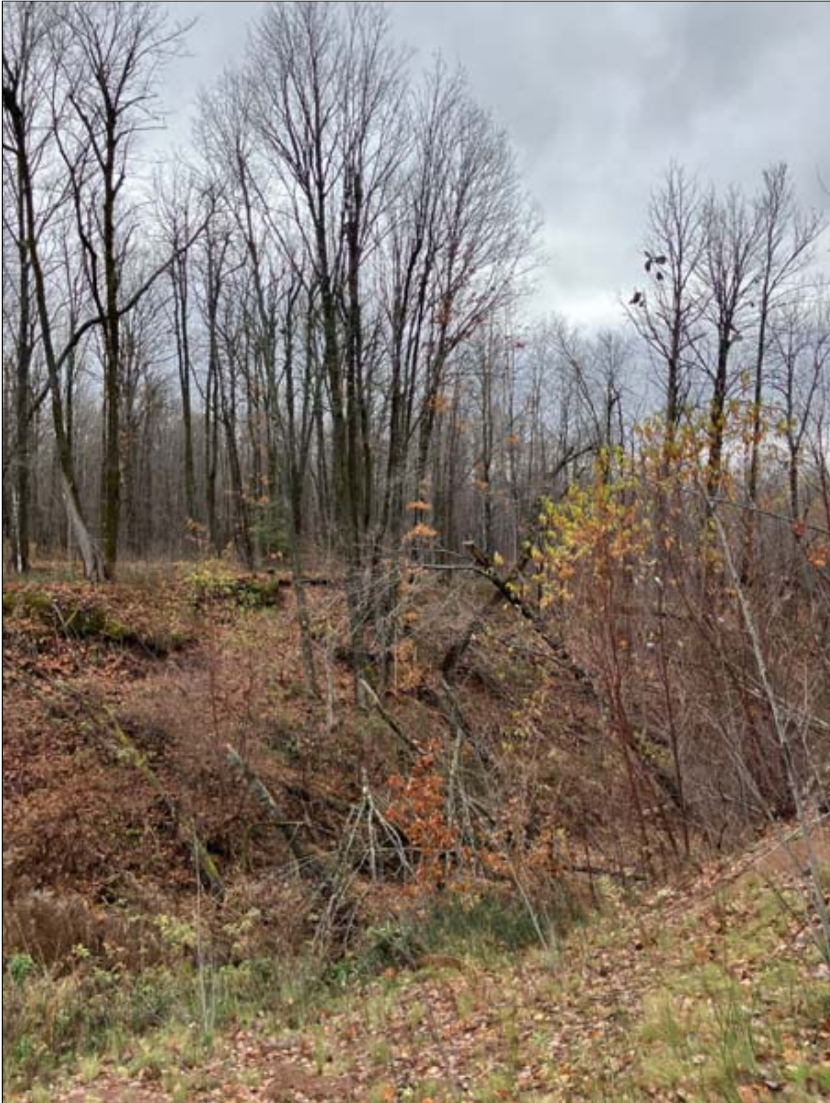
Figure 5.6-24 Newly formed gully along Potato River Road, October 2023.
