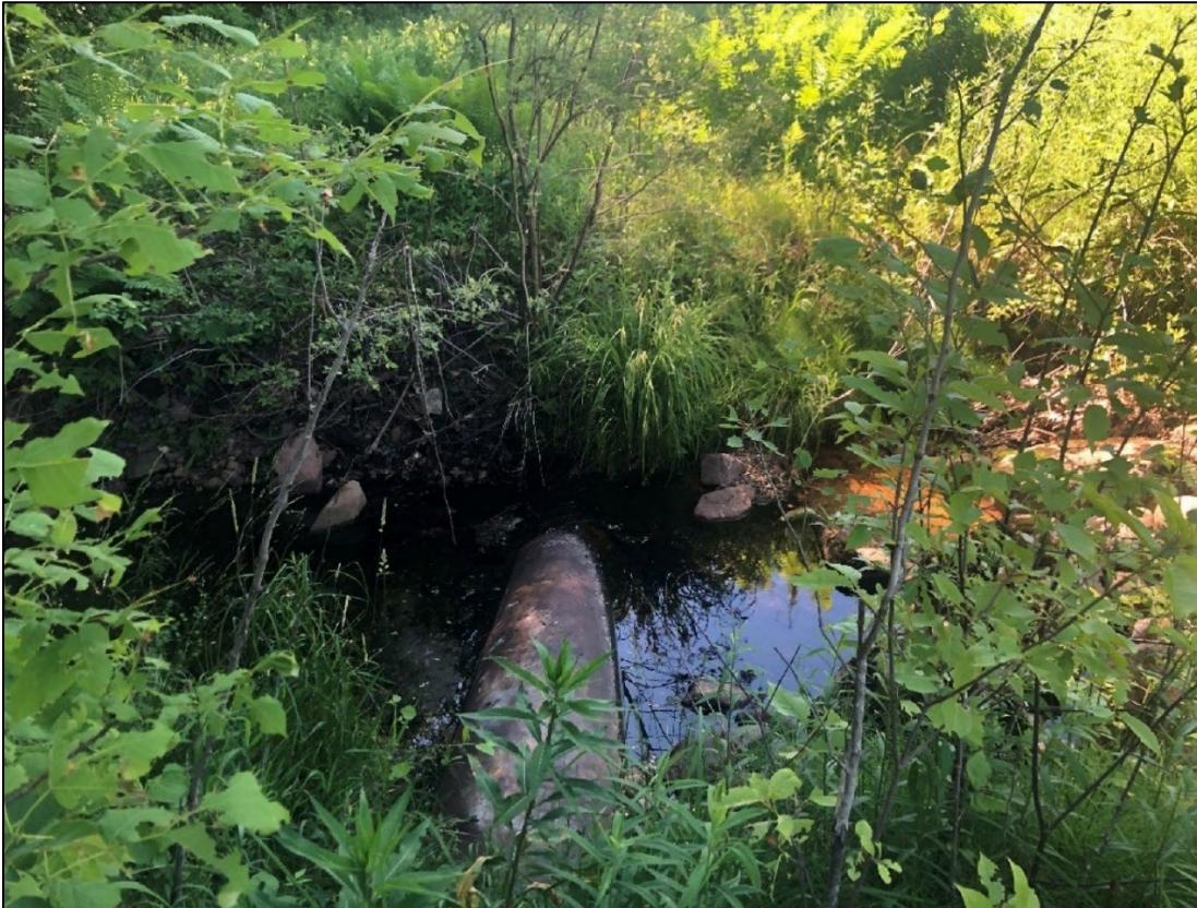
Figure 5.6-13 Enbridge Line 6A pipeline exposure at stream crossing June 2021.
