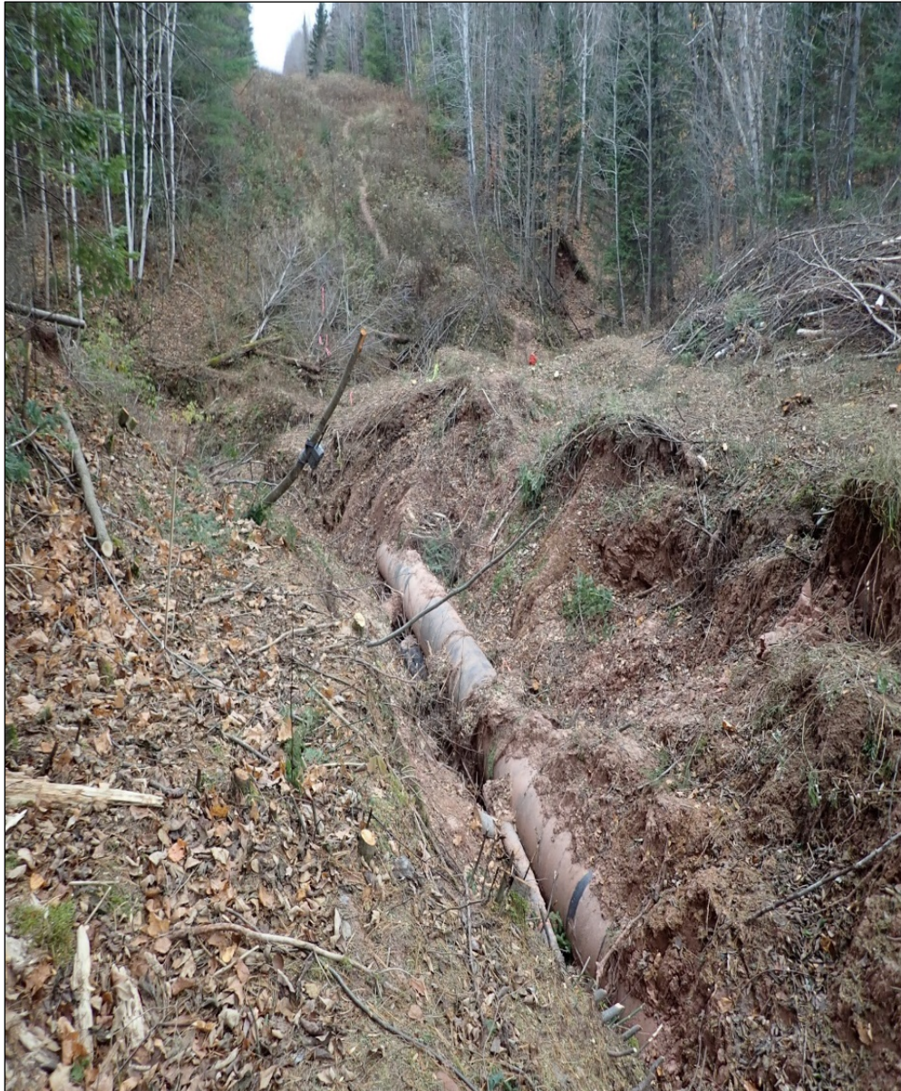
Figure 5.6-25 Gullying and pipeline exposure at Slope 18 failure.
