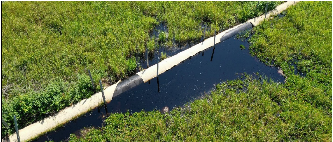
Figure 5.6-12 Enbridge Line 6A pipeline exposure in a wetland, Rusk County. Photo: DNR
