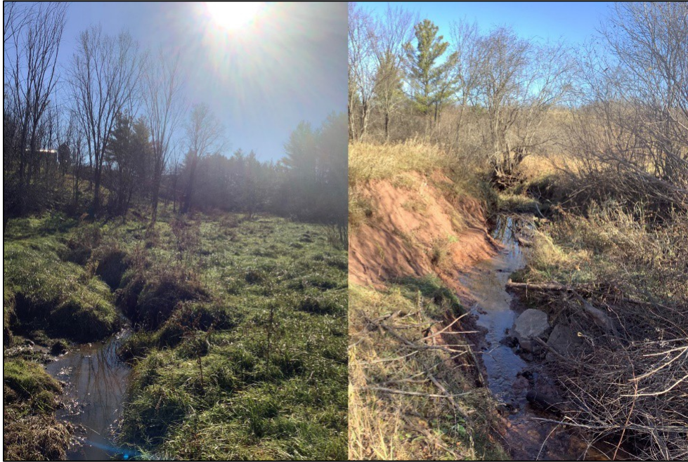
Figure 5.6-26 Knickpoint at a Culvert Crossing
