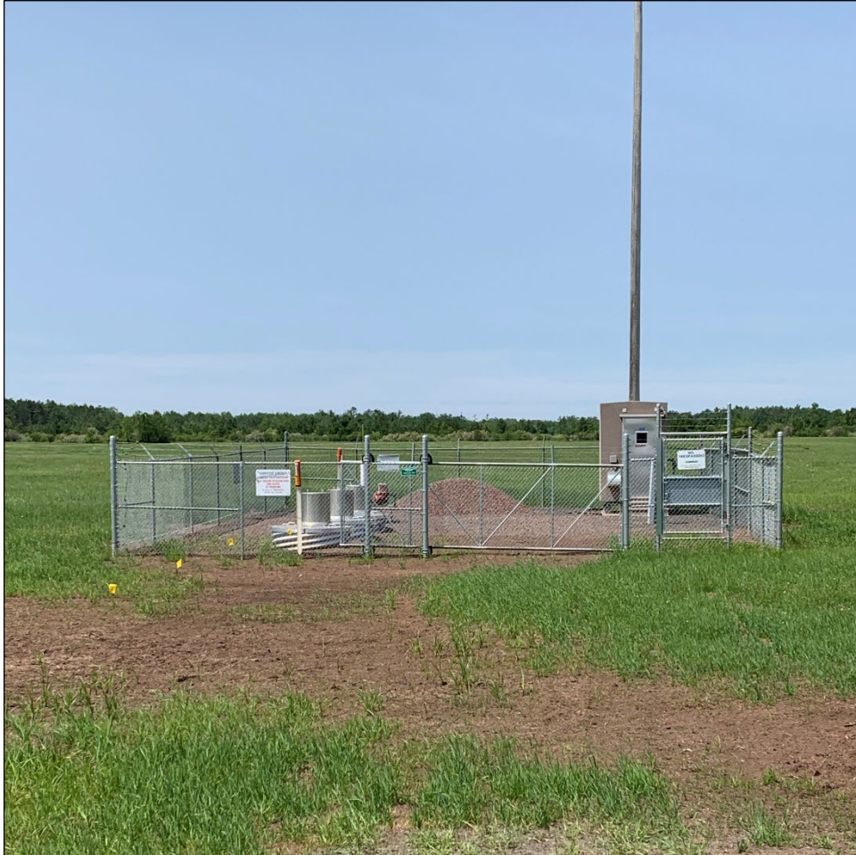
Figure 2.1-10 A mainline block valve site.
