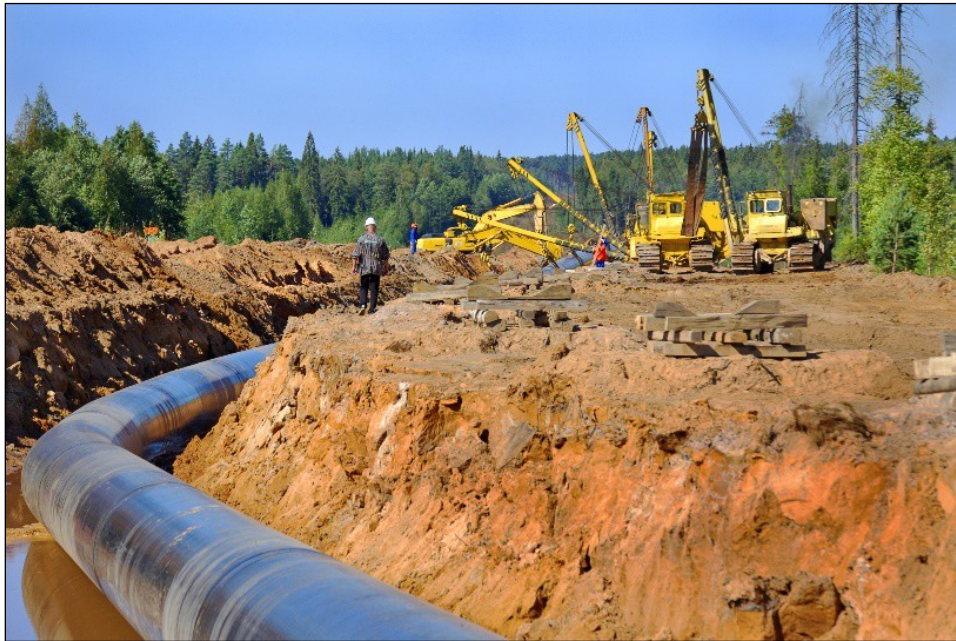
Figure 2.6-5 Bent section of pipe in trench.
