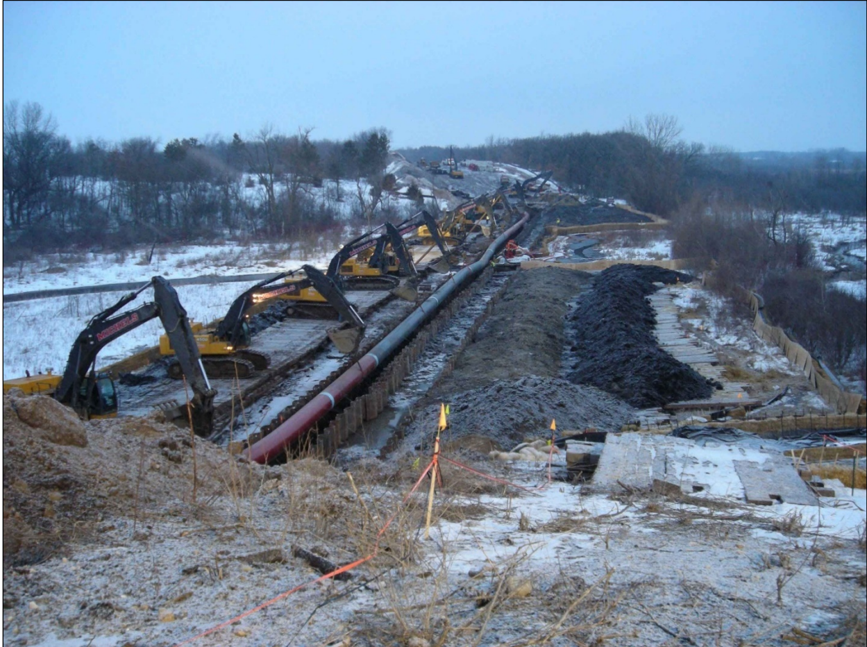
Figure 2.6-4 Trenching across an unnamed stream and riparian wetland, Enbridge Southern Access, Jefferson County.
