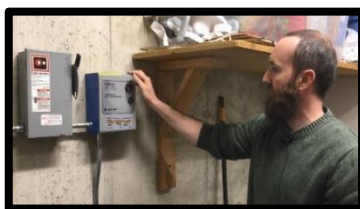
Electrical control box
