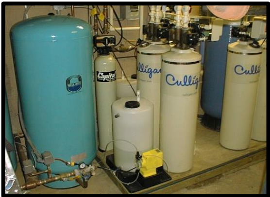
Chlorination injection system and pre-treatment devices
