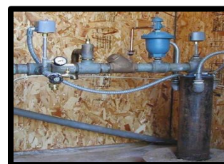
Above ground discharge & controls on discharge line
