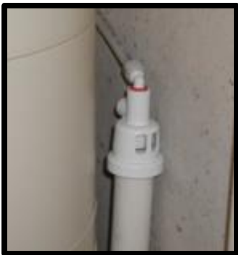
Manufactured air gap for water treatment backwash
