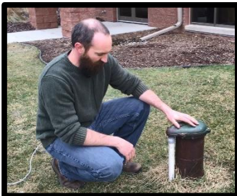
Well casing and well cap
