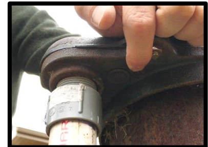
Well screen and conduit seal check
