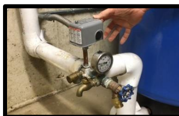
Well pump pressure switch box, pressure gauge and source sample faucet
