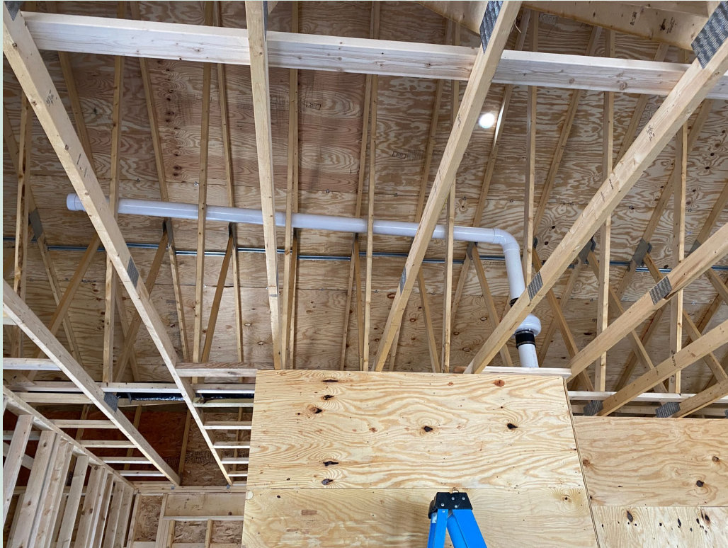
Riser, blower above ceiling
