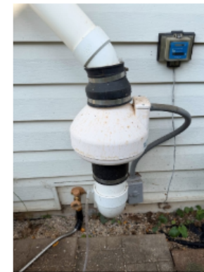
Example of vapor mitigation fan; typically located on the exterior.
