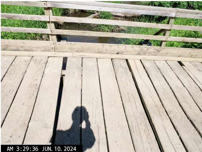
Timber Plank Gaps Looking Upstream to East
