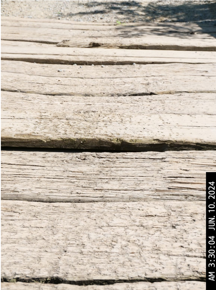
Deck Plank Wear looking to South at South end
