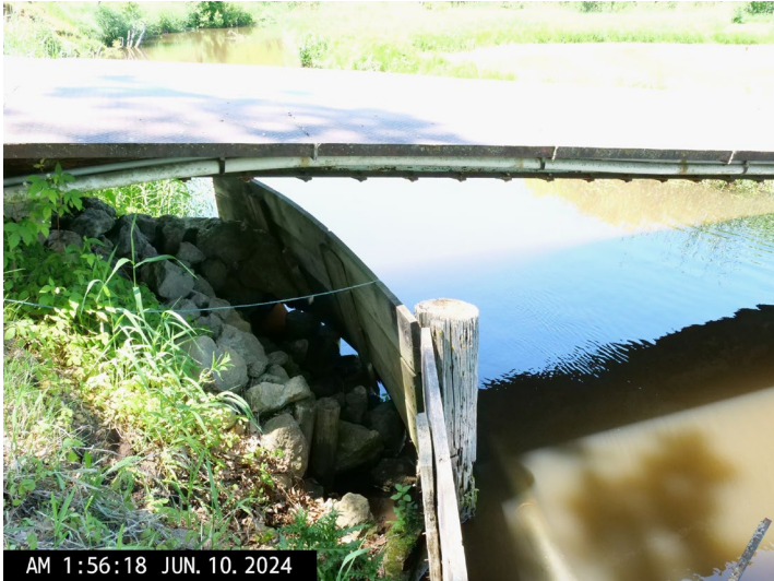
South Abut., Retaining Wall Timber Pile Deterioration
