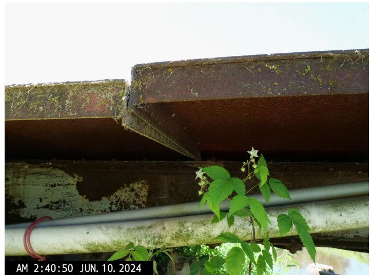
Bent Down Deck Panel
