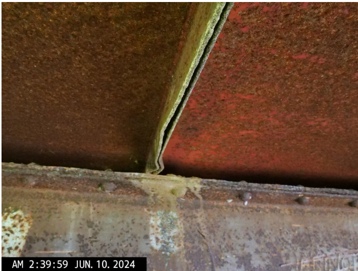
Failing Angle Iron Deck Panel Support
