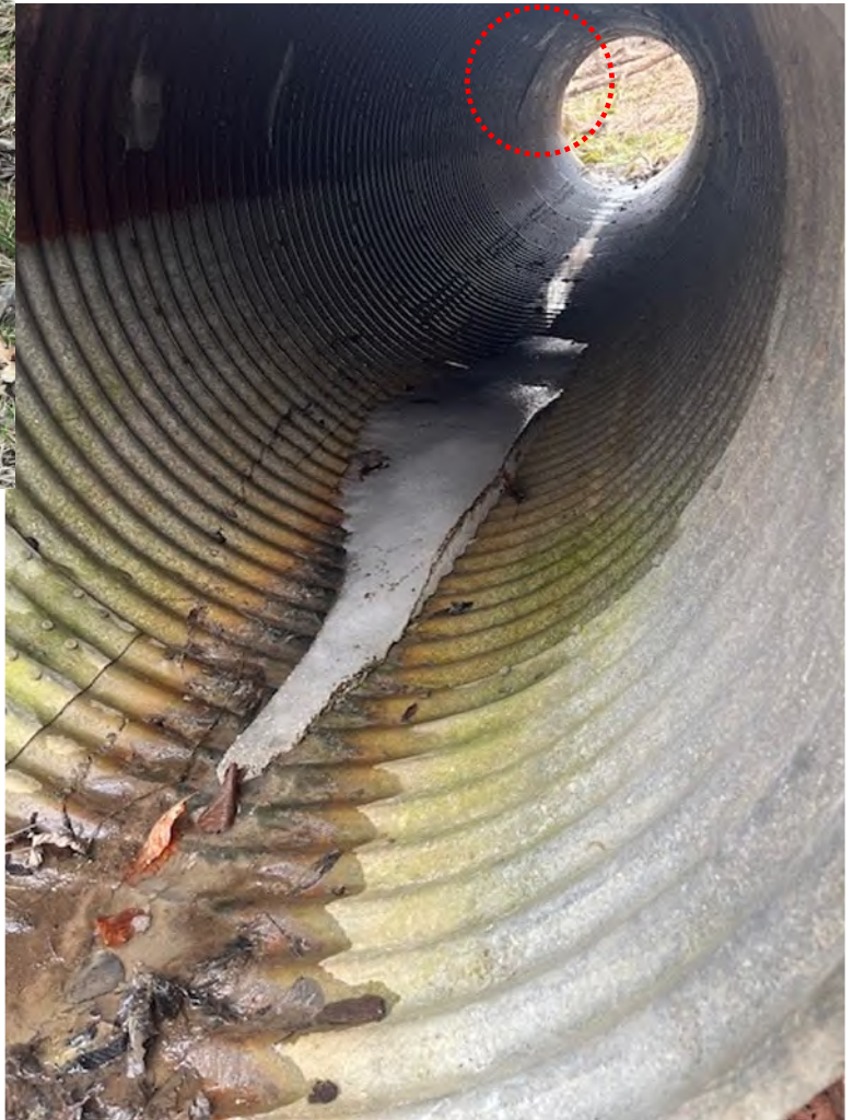
Culvert shows signs of rust and separation at the top in the back
