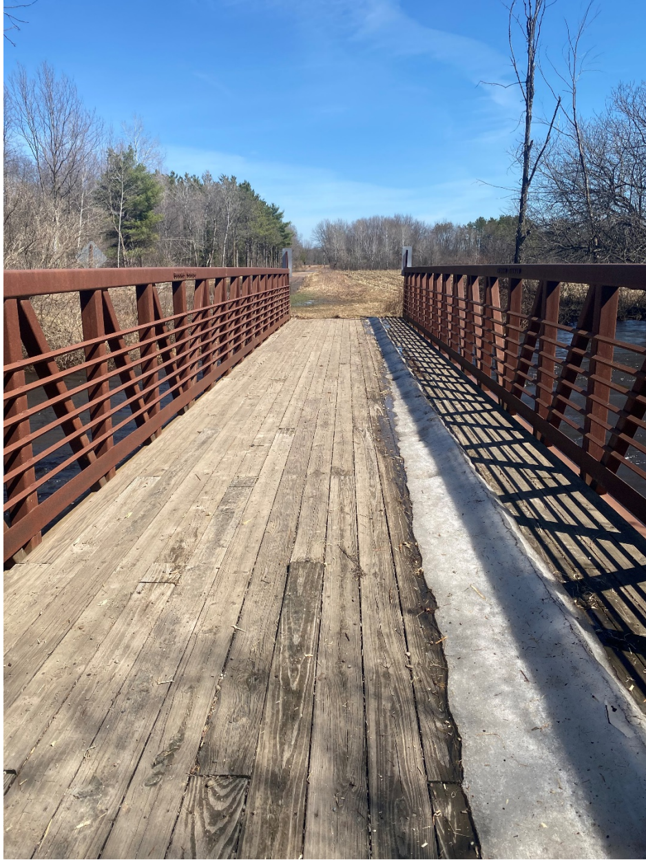
Looking east at the damaged bridge decking.
