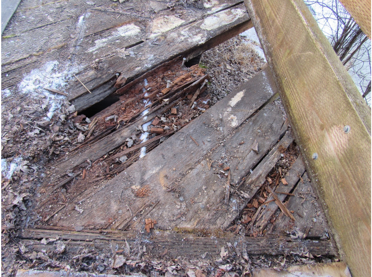
Bridge Deck Rotten
