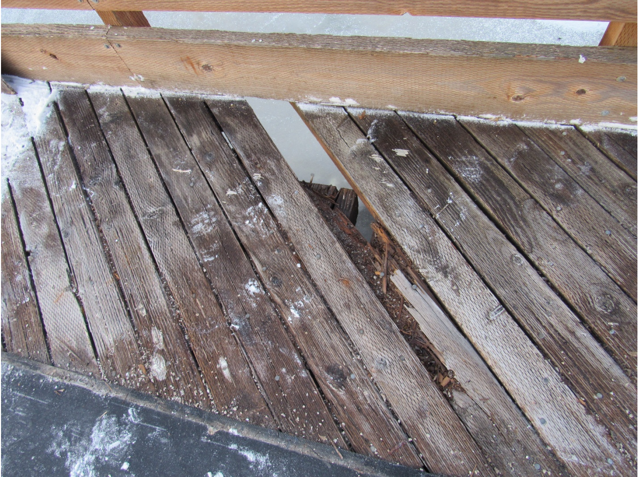
Bridge Deck Rotten
