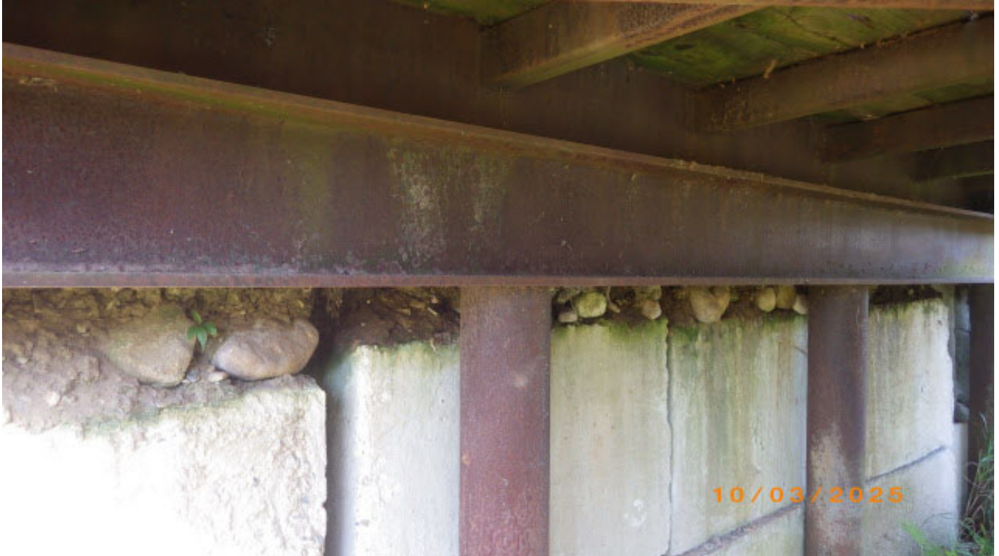
Large gap between bottom of pile cap and waste block backwall allowing fill to spill through
