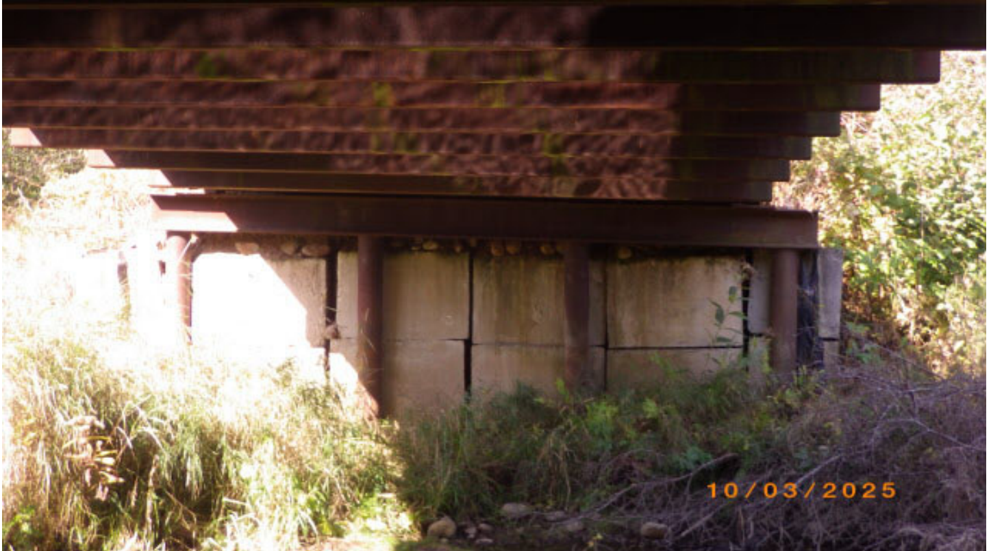
West abutment (note 4.8% tilt at pile cap)
