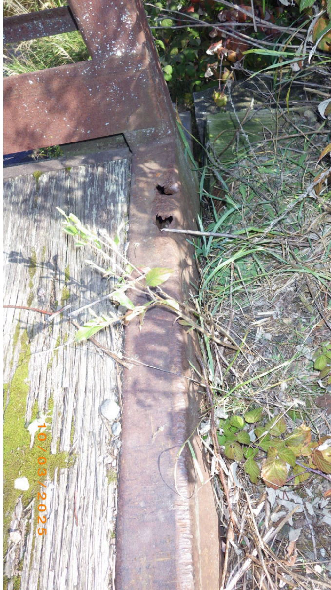
Horizontal end caps scraped and torn open from drag damage due to low approaches
