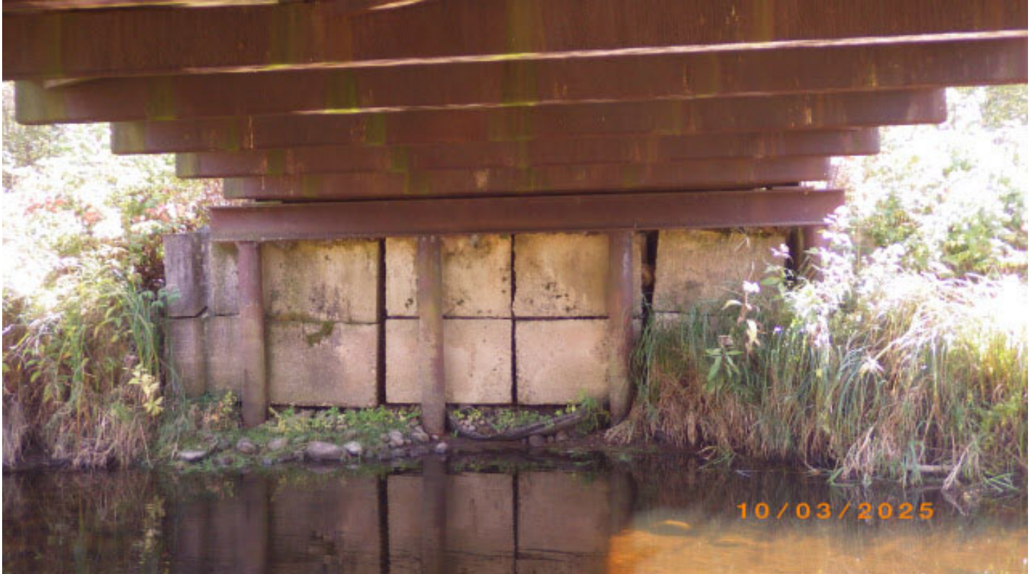
East abutment (note 1.6% tilt at pile cap)
