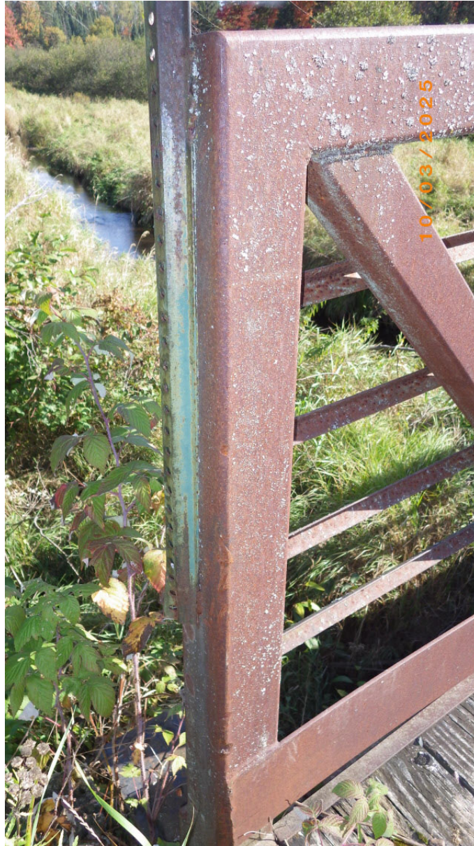
Superficial minor damage to NW corner truss vertical
