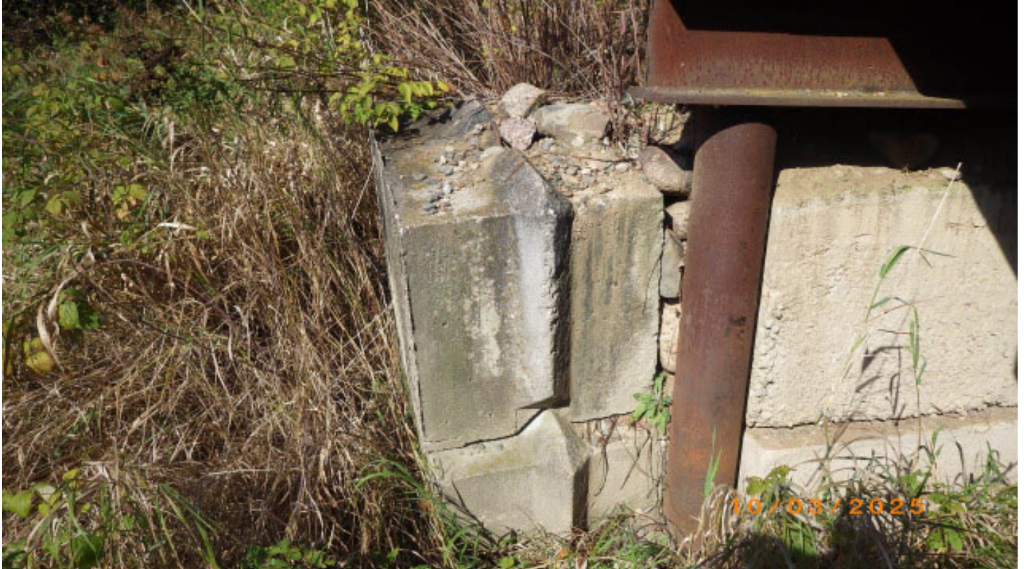
Waste block wingwalls out of plumb and level but not yet critical
