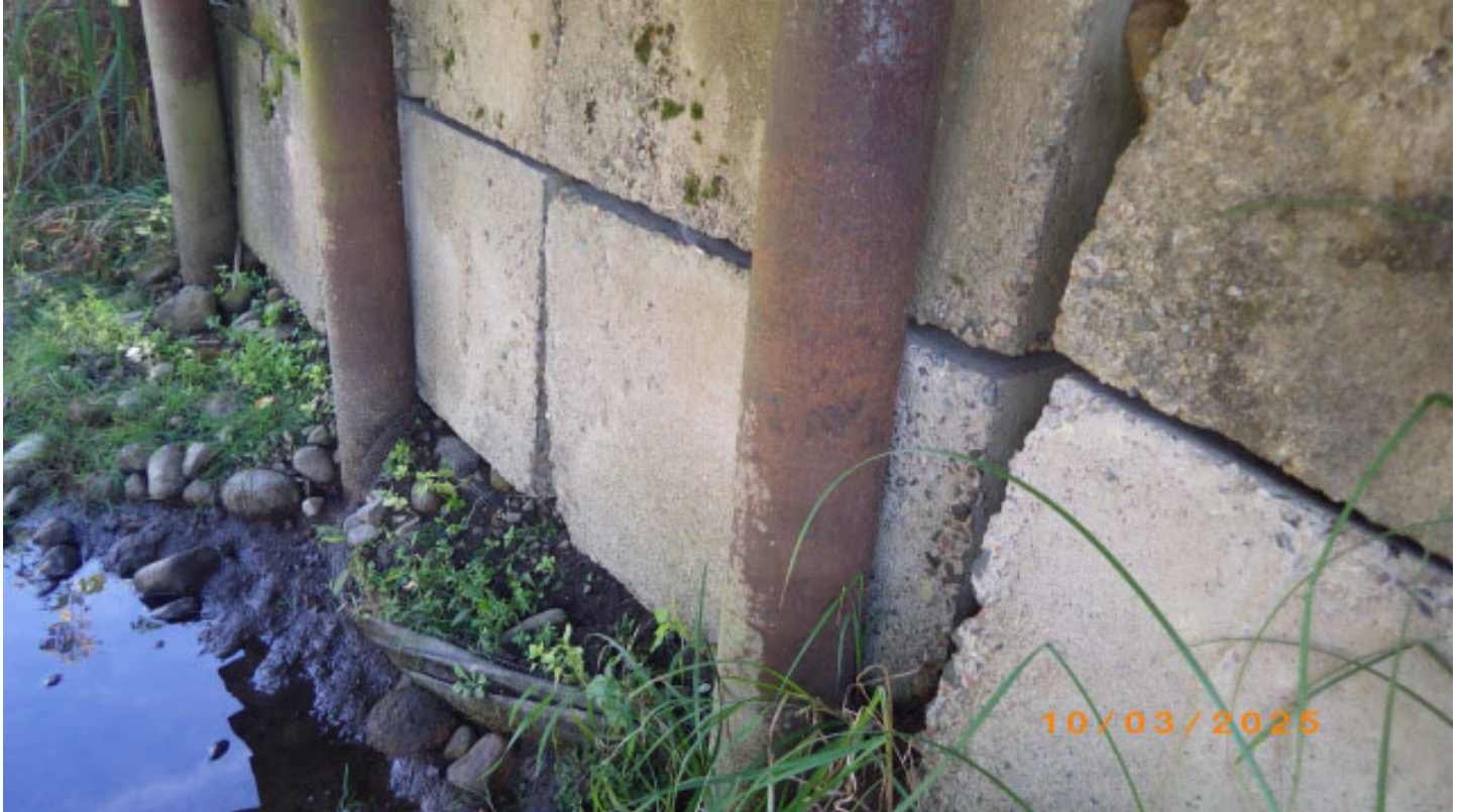
East backwall slightly undermined and SE corner moderate tilt
