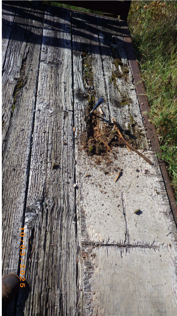
CS4 rotten deck planks
