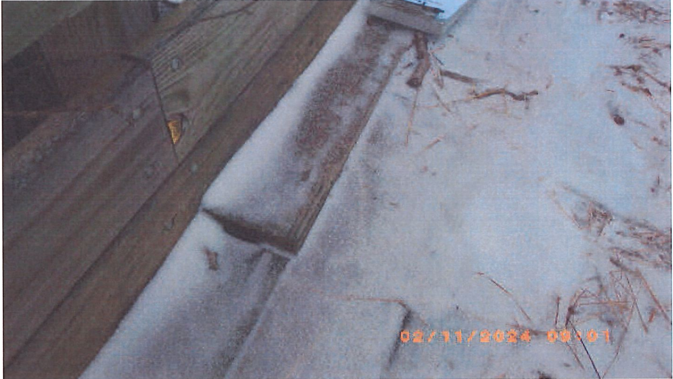
Wear plank loose and coming up
