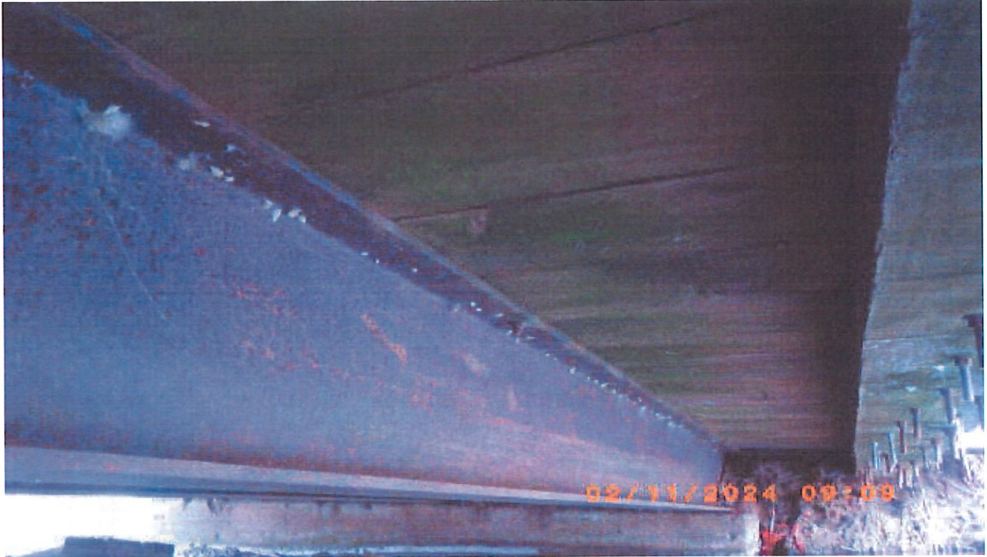
Typical underside of deck / green mold
