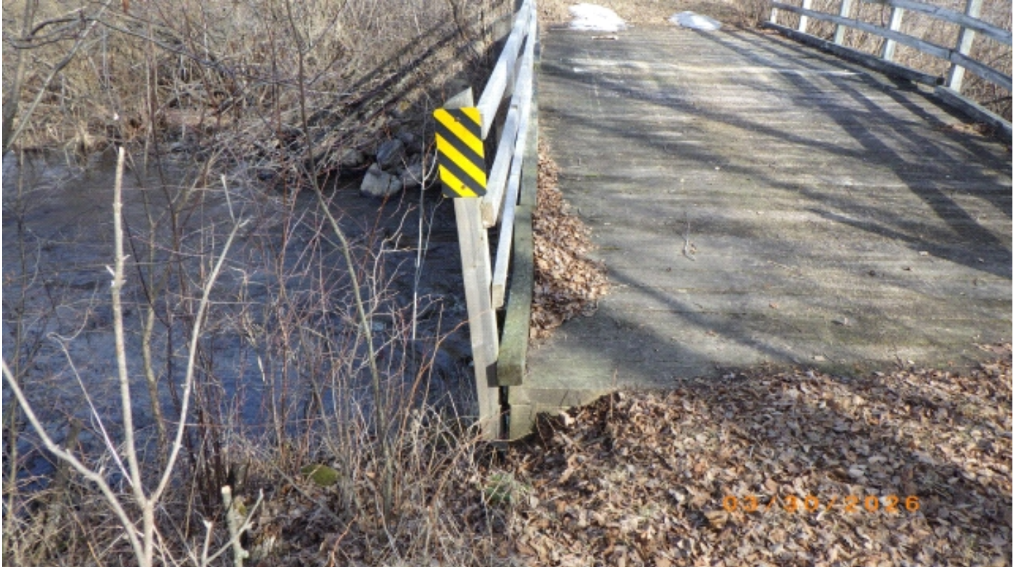
Leaning SW railing.
