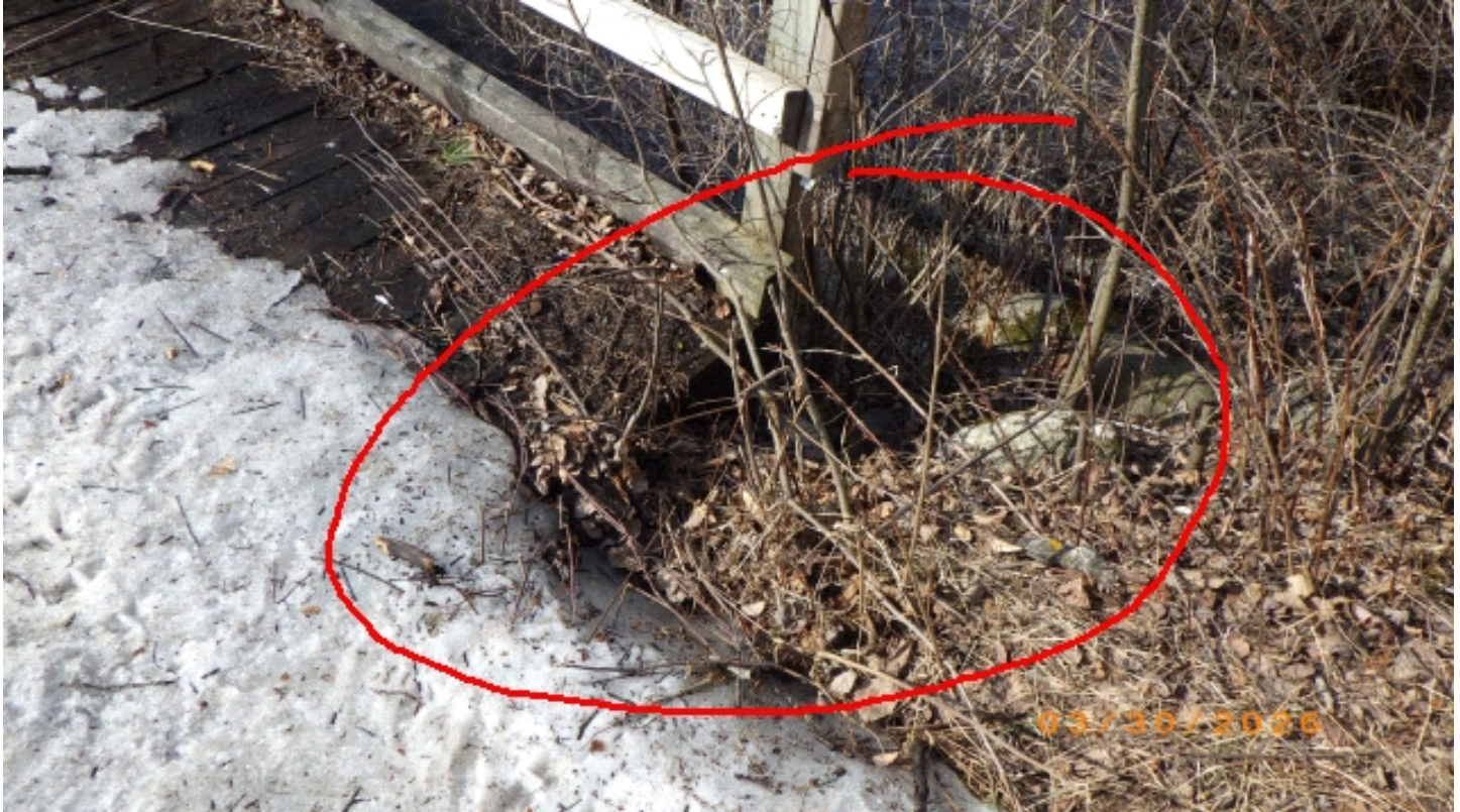
Hole at NW approach, Bring up to grade to protect the deck edge.
