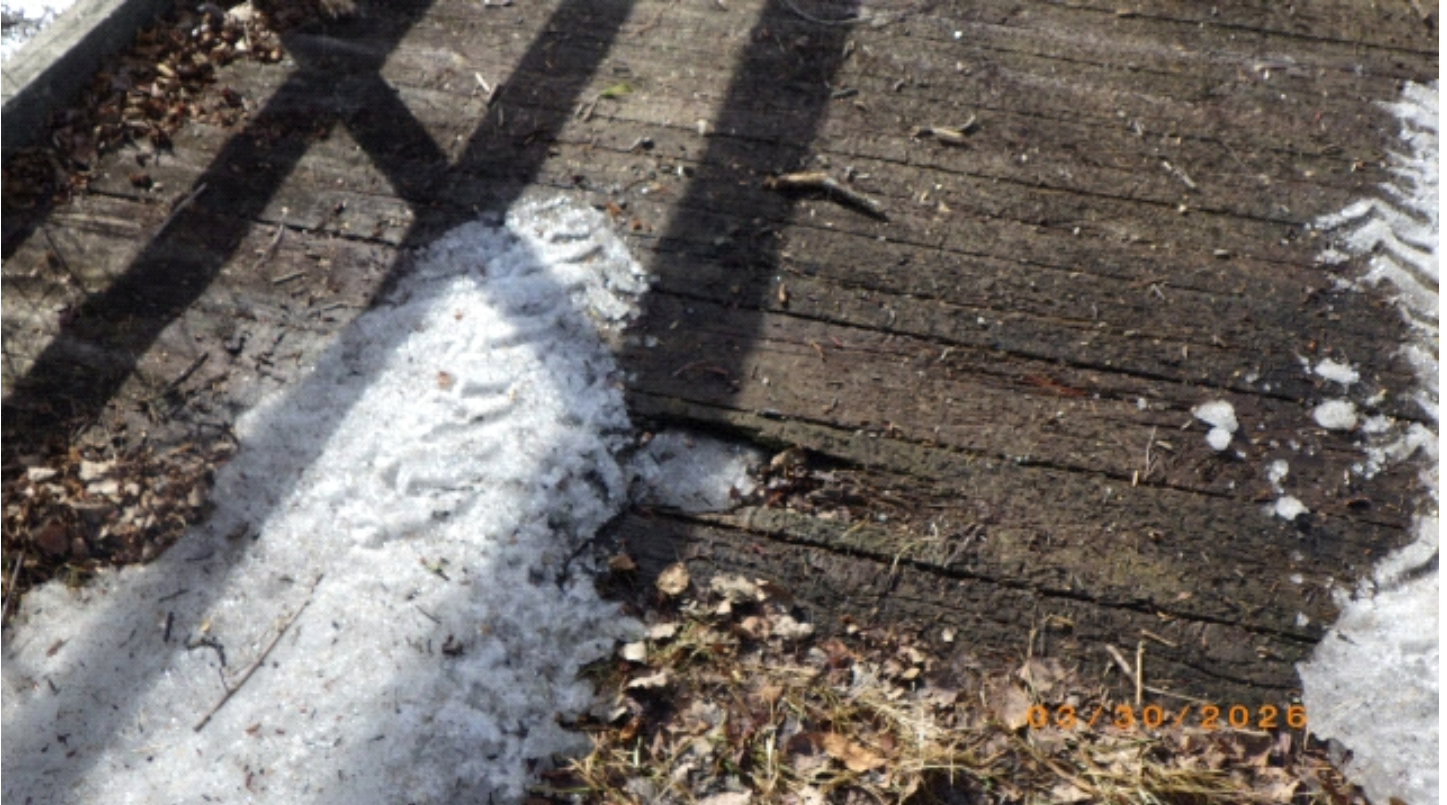
Hole in top of deck.
