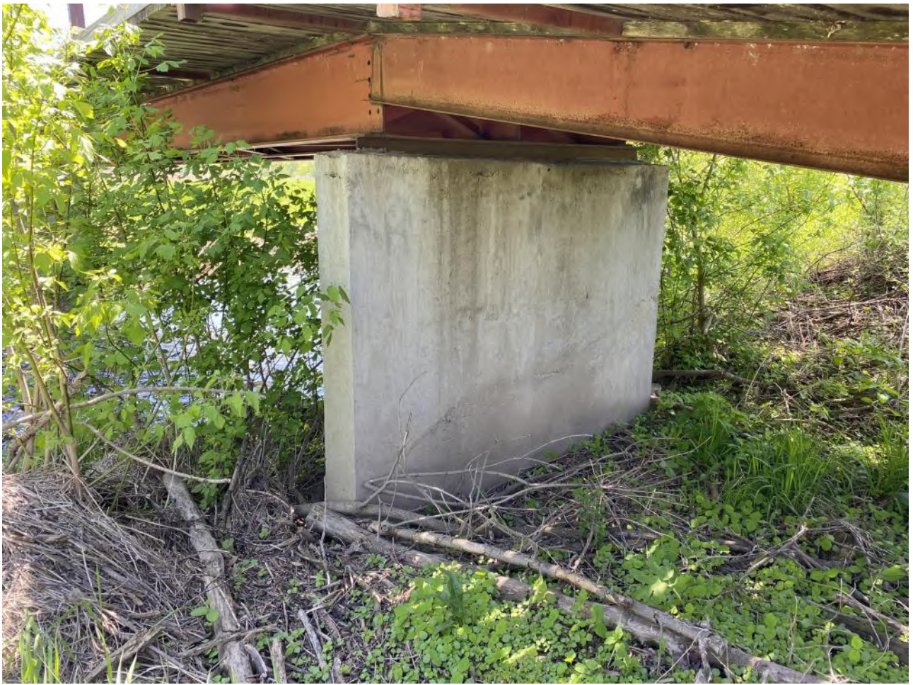
Set high on narrow concrete abutments. Rip rap missing so bridge has little protection
