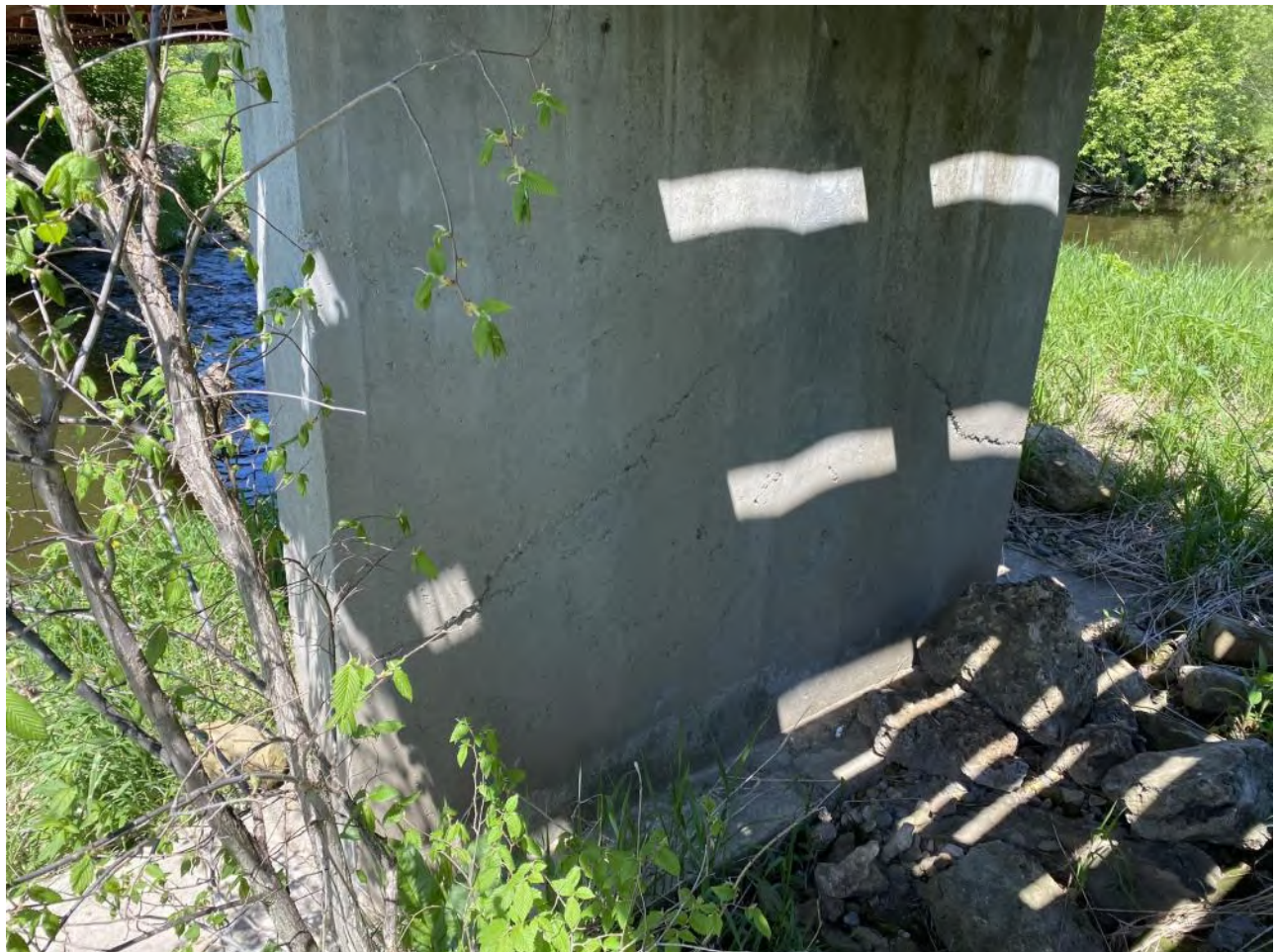
Not sure if this is just a pour line or a crack in the abutment
