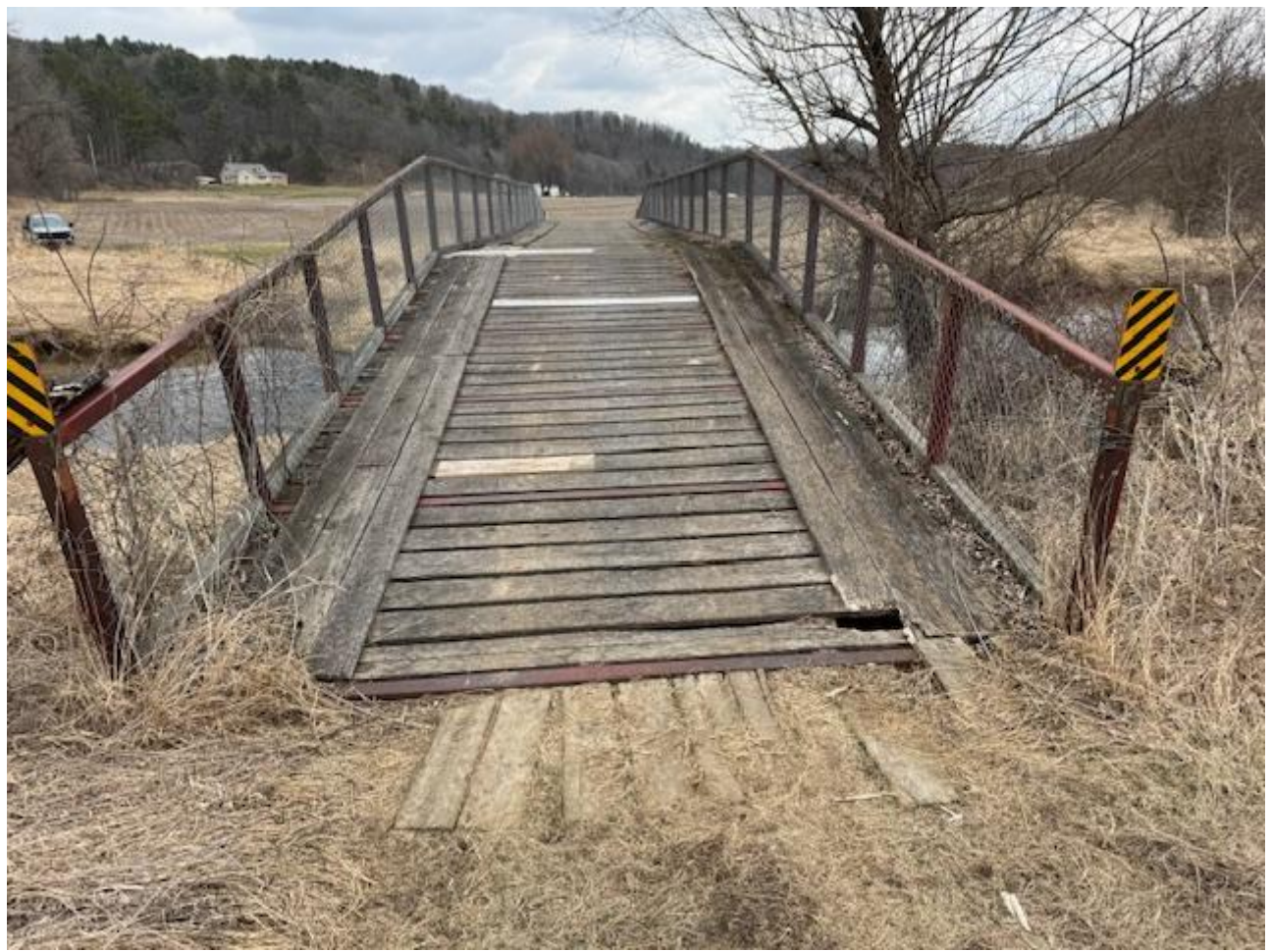
Approach from the north. Groomers are unable to cross this bridge and take a river crossing instead.
