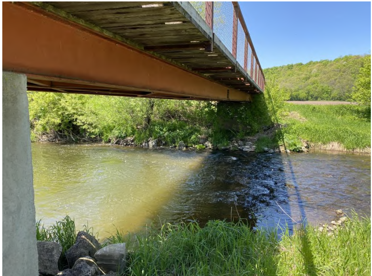
The area is in need of more rip rap to protect the bridge
