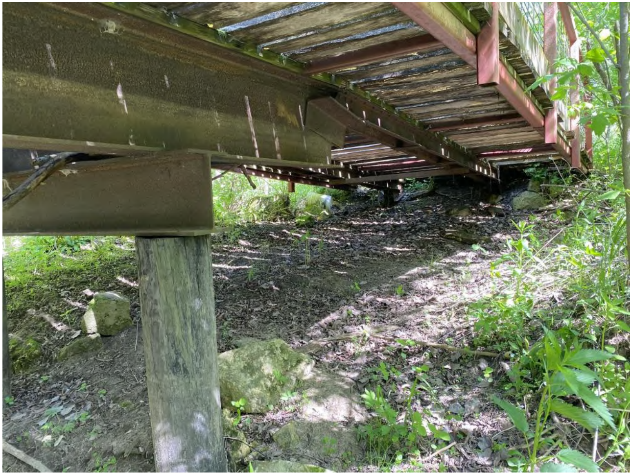
Ramp on North end. Very little rip rap remaining.
