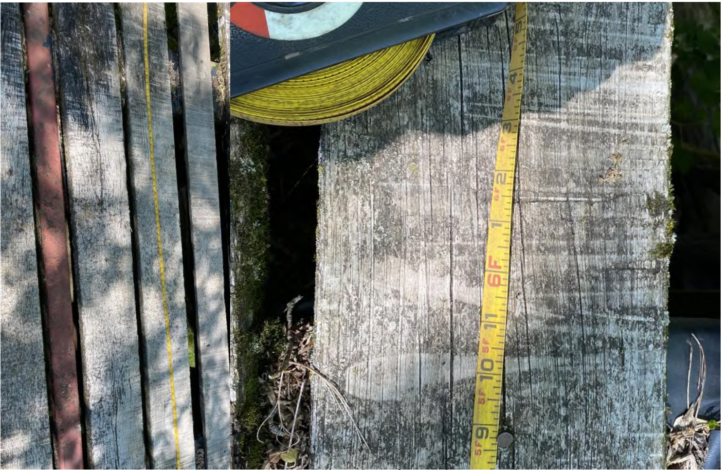
Measurement overview. I-Beam Spacing is a little less than 6' outside to outside
