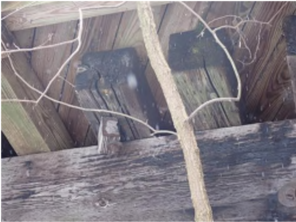
Typical splits in timber stringer ends, looking northwest (taken Jan 2026)
