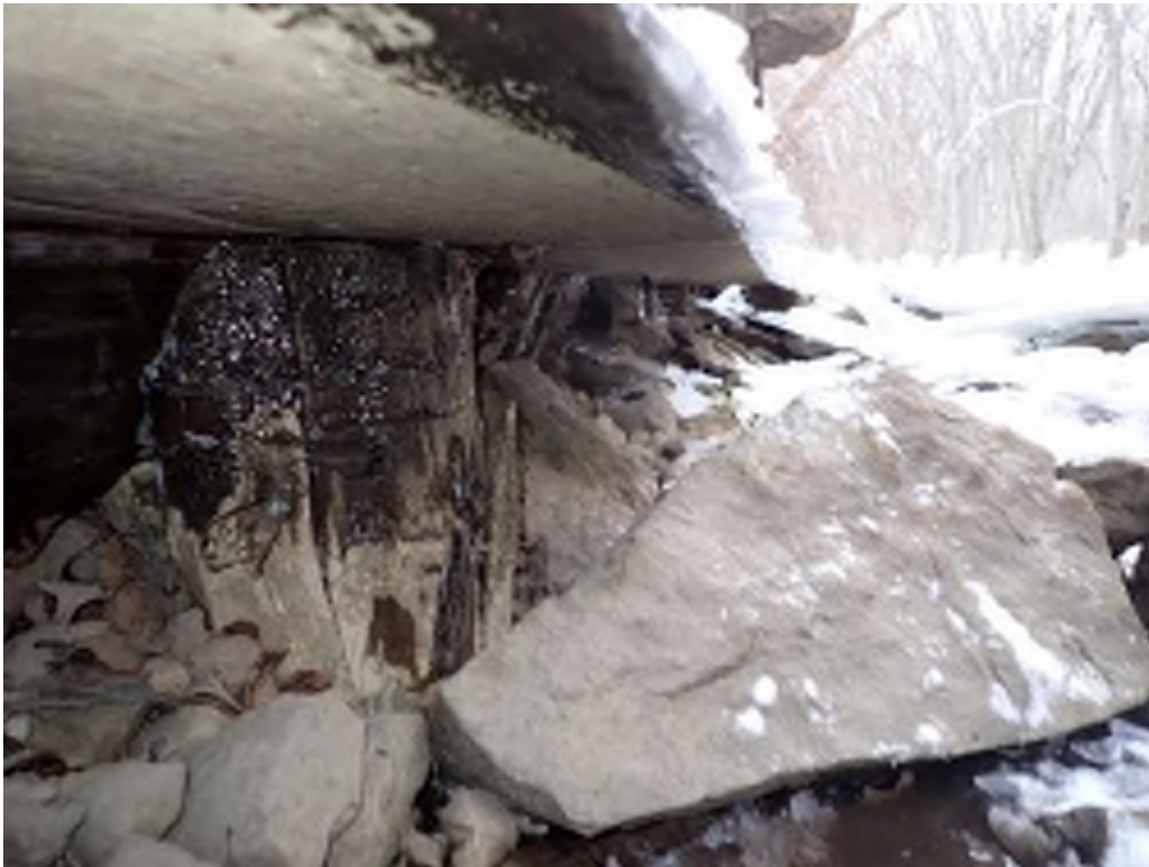
Pier 11W pile deterioration, looking south (taken Jan 2026)
