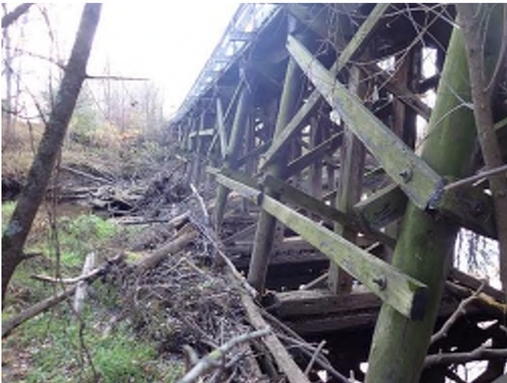
Debris on north side, looking southeast (taken Oct 2025)
