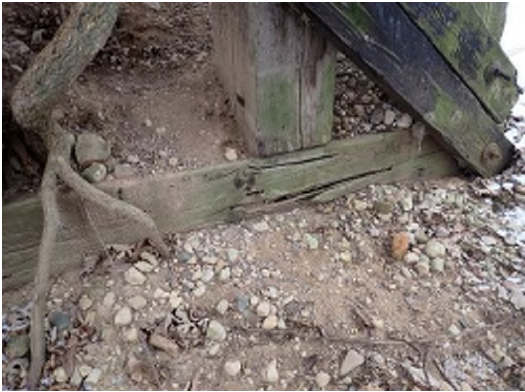
Typical pile cap delamination / decay, looking southeast (taken Jan 2026)
