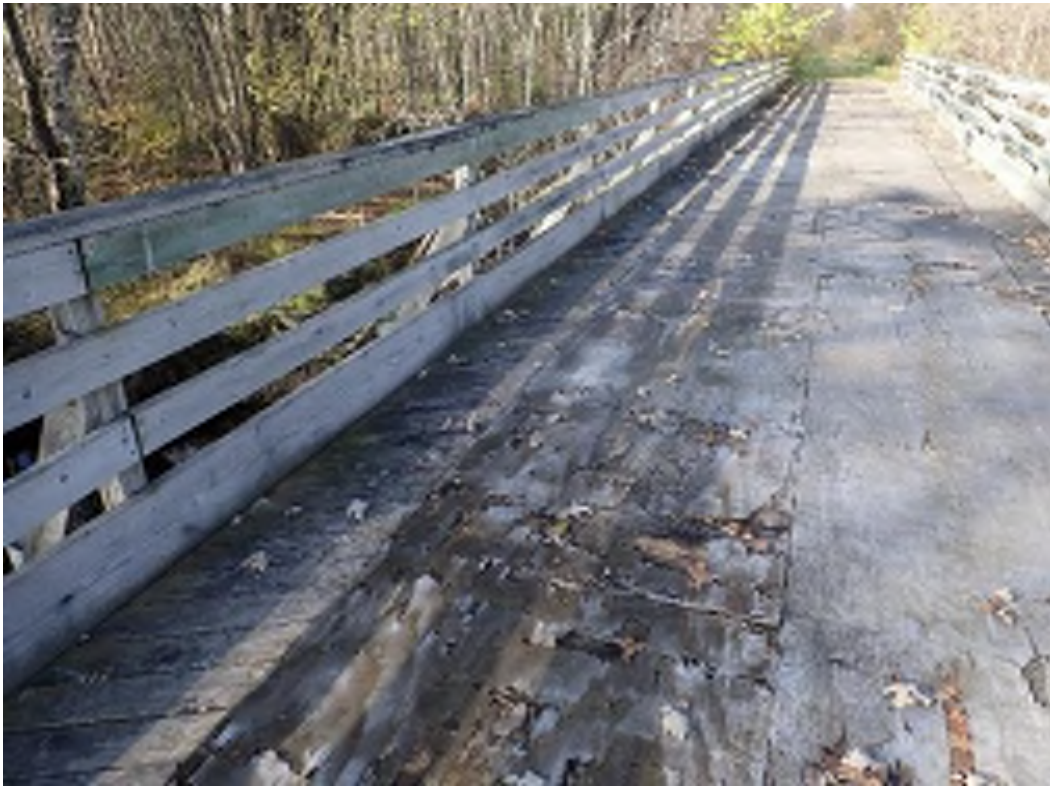
Typical wearing surface deterioration, looking southwest (taken Oct 2025)
