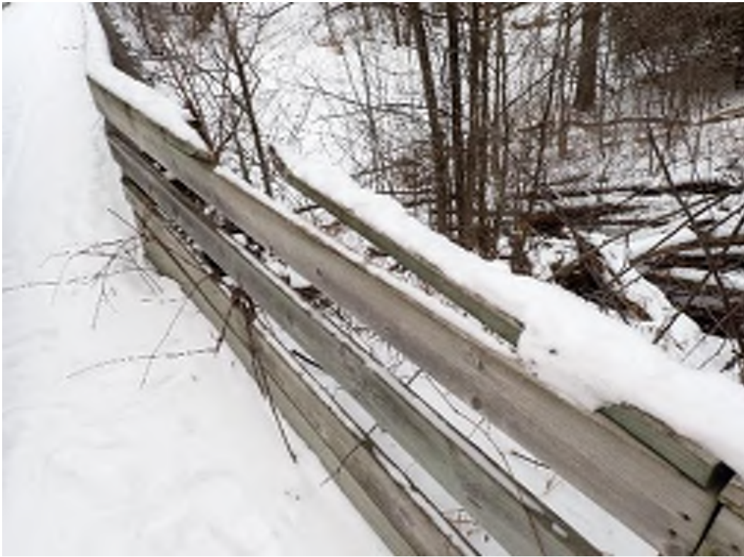
Broken top rail on east end, north side, looking west (taken Jan 2026)
