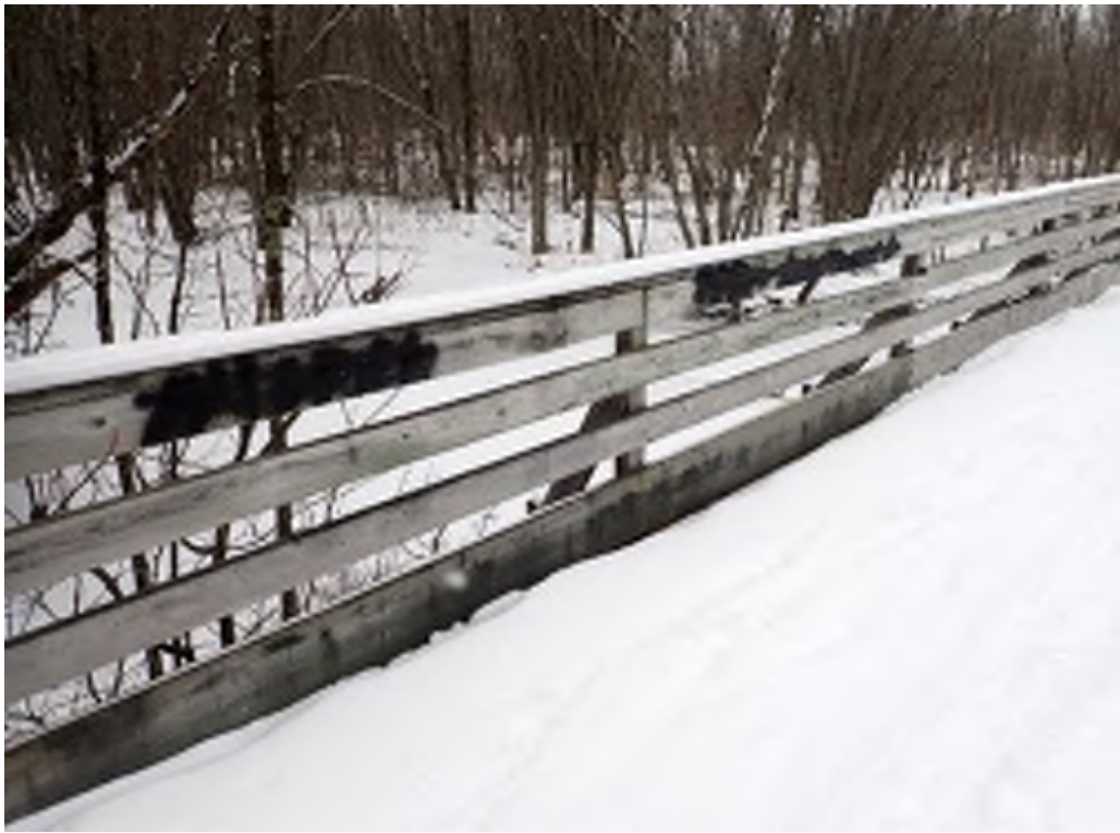
Typical graffiti, looking southeast (taken Jan 2026)
