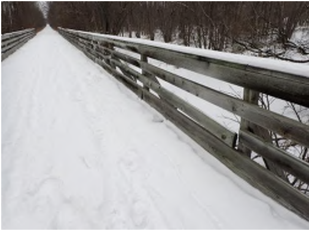
Broken rail connections on north rail, looking northwest (taken Jan 2026)
