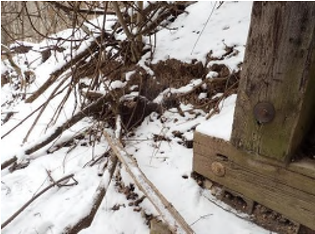
Typical bank erosion on west side, looking southwest (taken Jan 2026)
