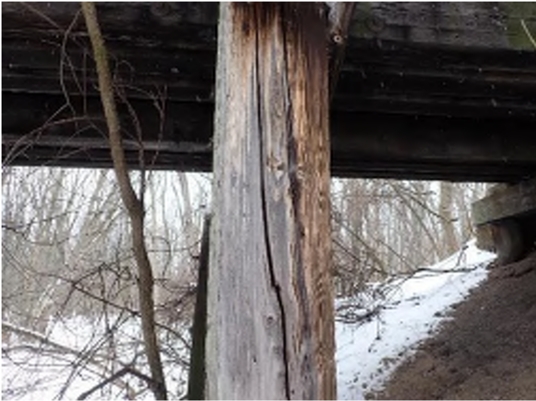
Typical column splits in pier, looking north (taken Jan 2026)
