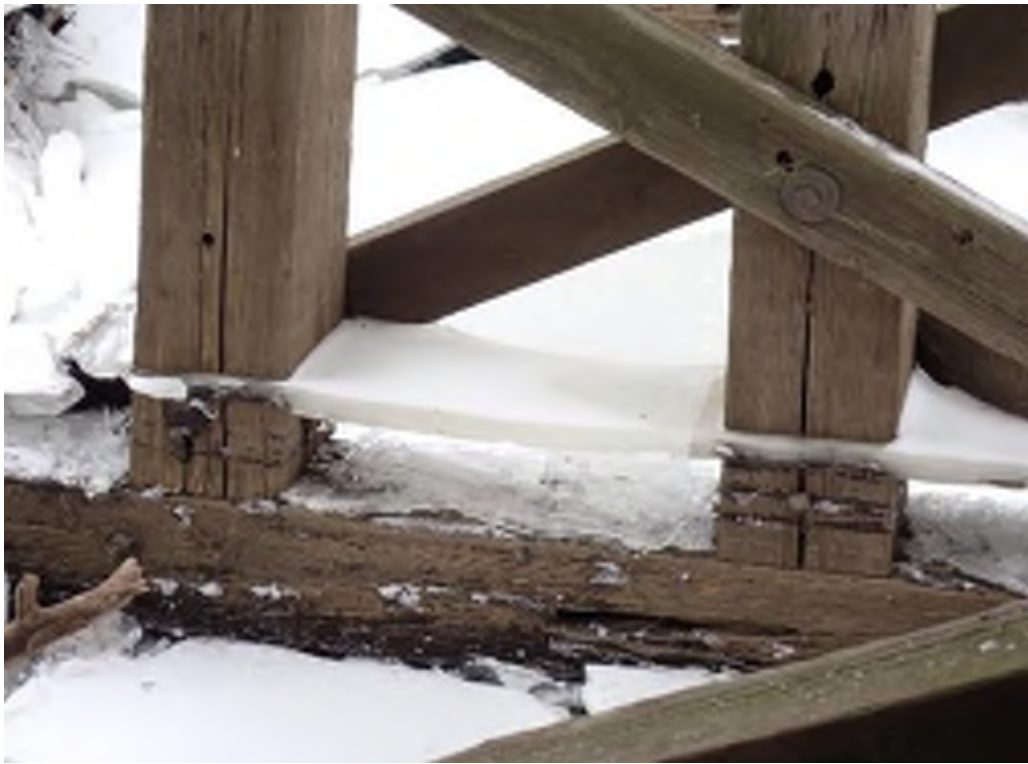
Typical splits in columns near pile cap, looking southwest (taken Jan 2026)
