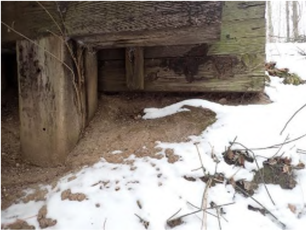
East abutment backwall erosion, looking east (taken Jan 2026)
