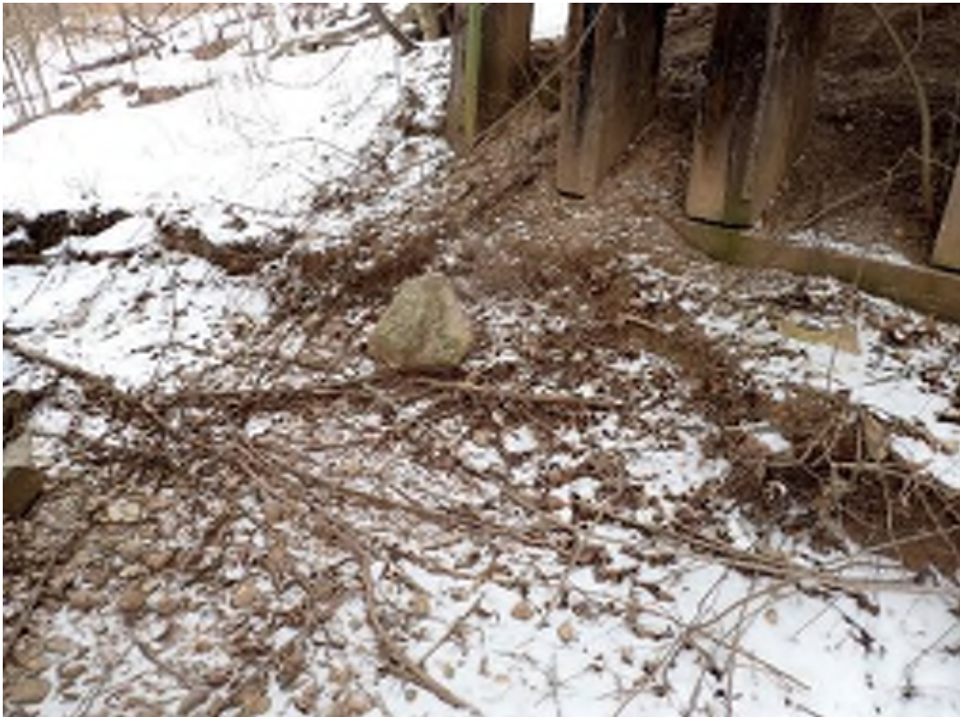
Typical bank erosion on east side, looking northeast (taken Jan 2026)
