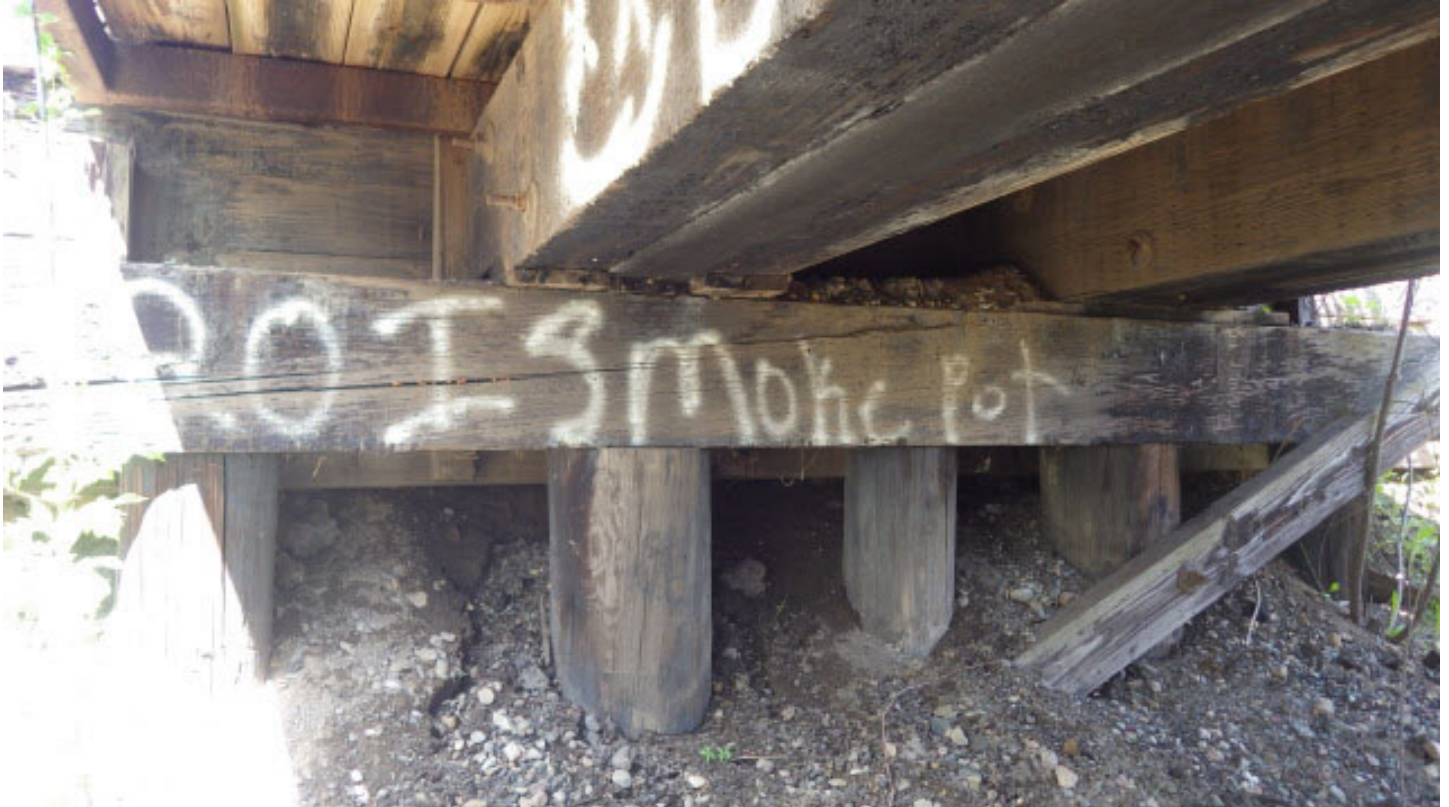
North abutment cap rotten / crushing / fruiting bodies growing from it
