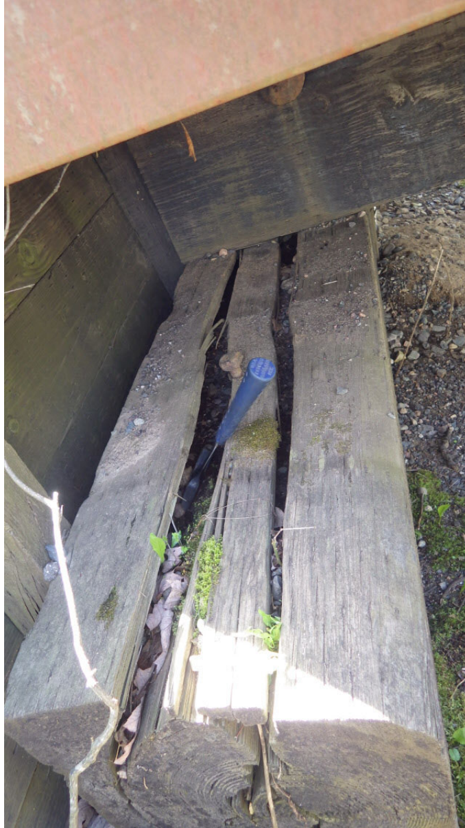
South abutment cap rotten / crushing at east bearing
