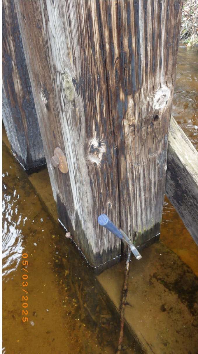
Bent #4 Posts 2 and 4 are hollow
