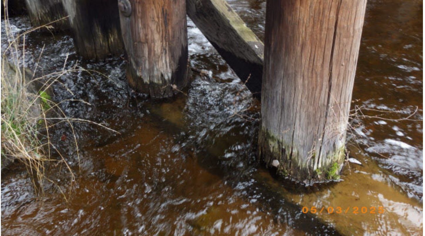
Bottom of posts in water rotten
