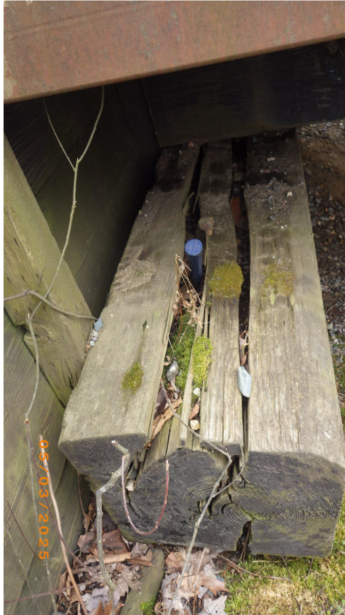
South abutment cap rotten / crushing
