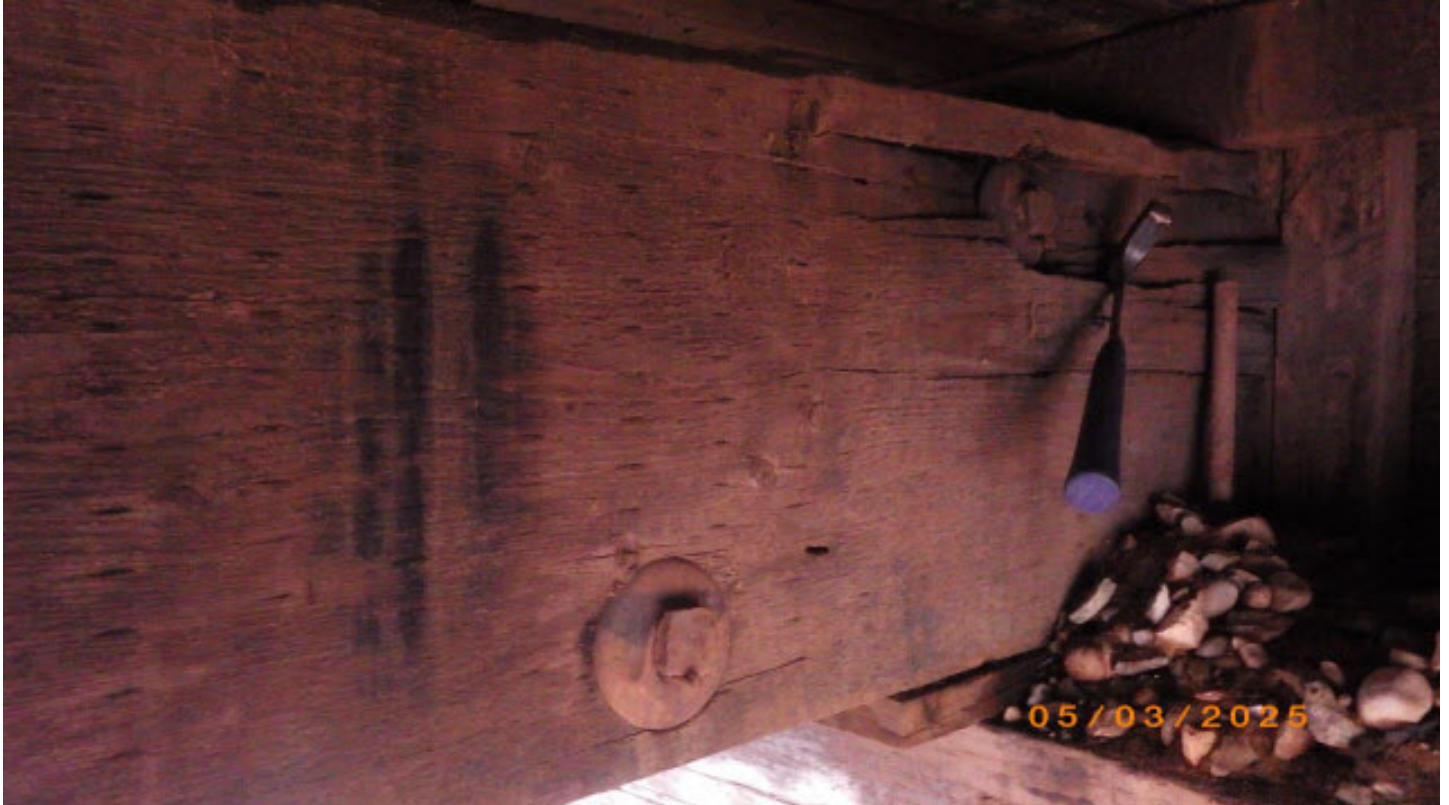
Span 6, girder 3 rotten / crushing at north end
