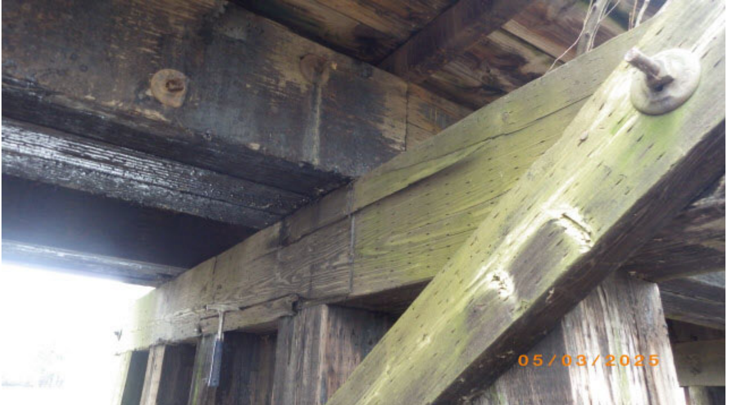
Bent #4 top cap rotten / crushing
