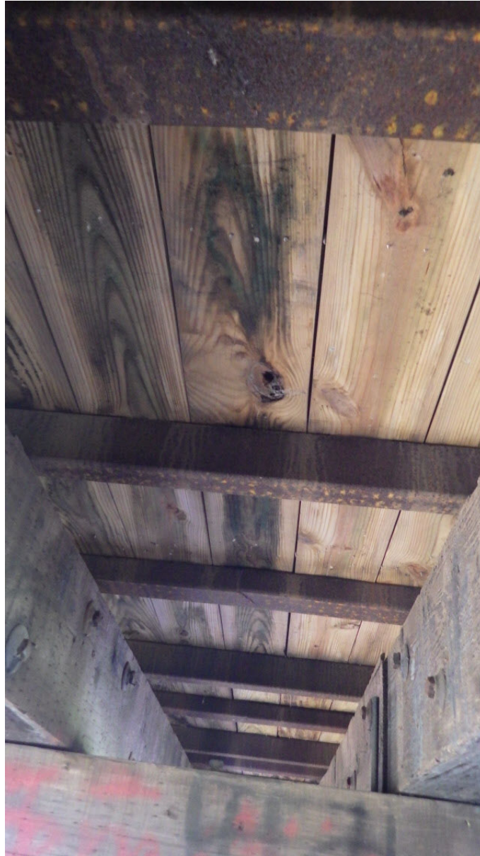
Black staining on deck underside
