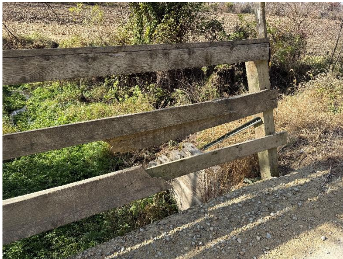
Photo 9 – North End of West Rail.
