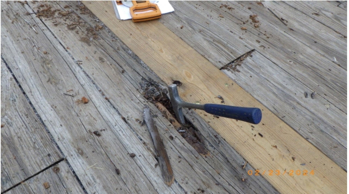
Deck Rot, measurable section loss.
