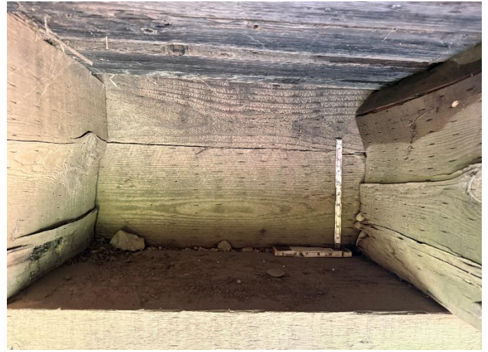
Photo 8 – Beams Crushing Over South Abutment.
